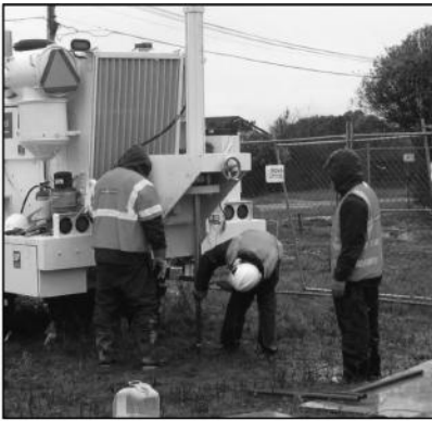
(a) Installing 2D velocity transducers (geophones) and pore pressure transducers (PPTs) with the hydraulic ram on the back of T-Rex.
