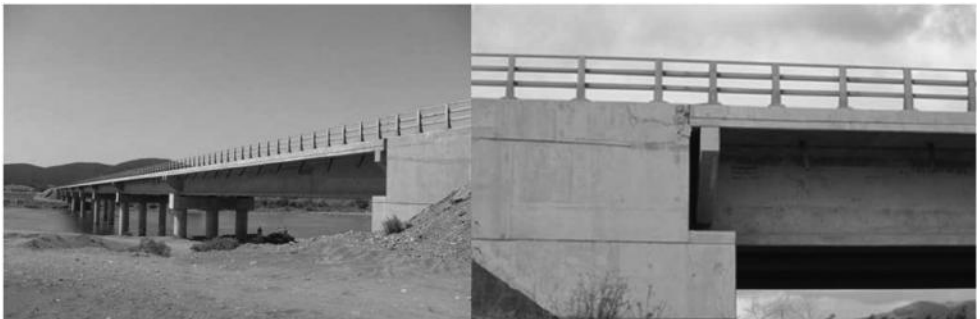
Figure 10. Pre- and post-earthquake views of the Mataquito bridge deck expansion gap. Pre-earthquake photo retrieved January 14 2013, www.panoramio.com/photo/8172577 . Post-earthquake photo from (GEER, 2010).
