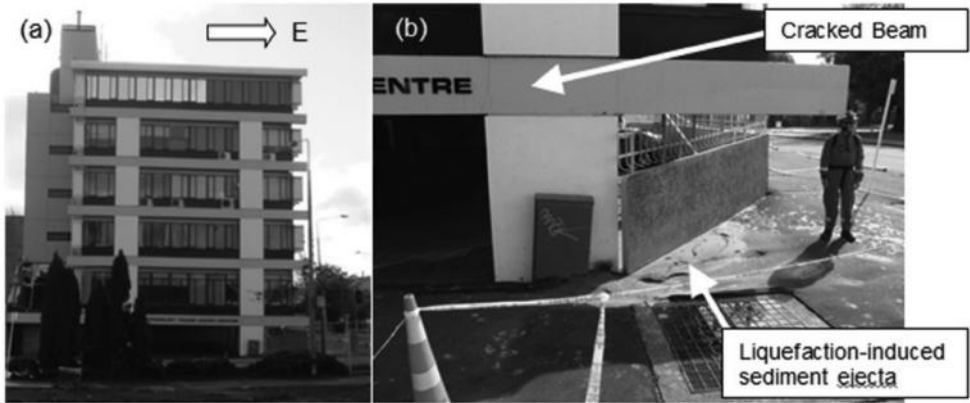
Figure 5. (a) South end of CTUC building showing tilt to the east (taken July 2011) and (b) Close-up photograph of the SE corner of the building (taken March 2011).
