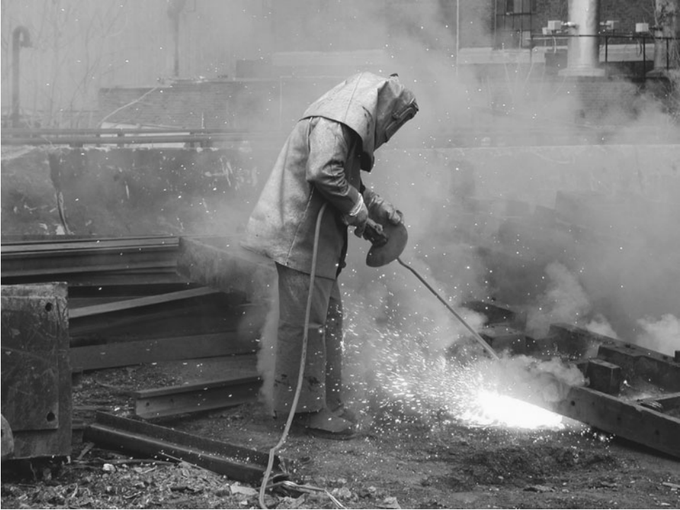
Figure 23-1. This worker is exposed to lead by cutting metal that has a lead-based coating.
