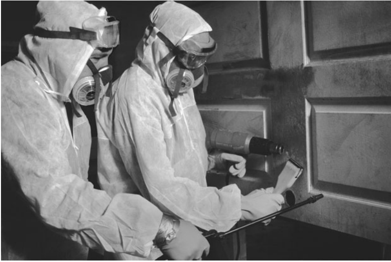
Figure 1-6. Lead-based paint in many older homes still represents a serious health hazard to many young children. This photograph depicts a lead abatement worker with personal protective equipment. Workers performing lead abatement must be trained and certified, and they must carefully adhere to safe practice standards. (Photograph by Earl Dotter.)
