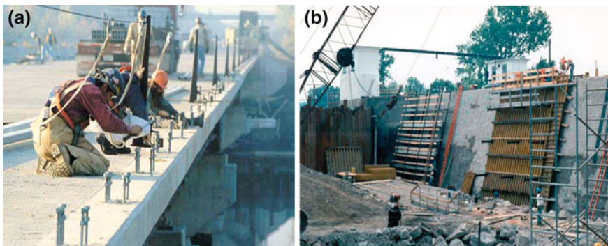
Fig. 5.23 Metakaolin was used on a I-87 overpass and b Reconstruction of erie canal
