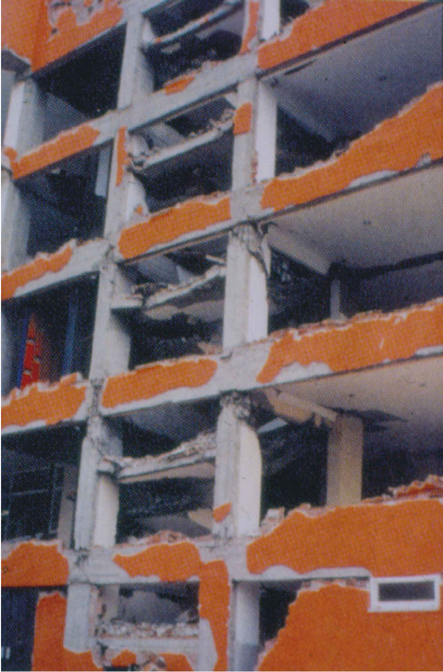
Picture 6.9 Out-of-plane failure of infill walls
