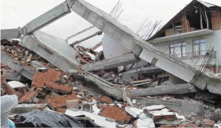
Picture 6.7 Typical beam–column junction failure
