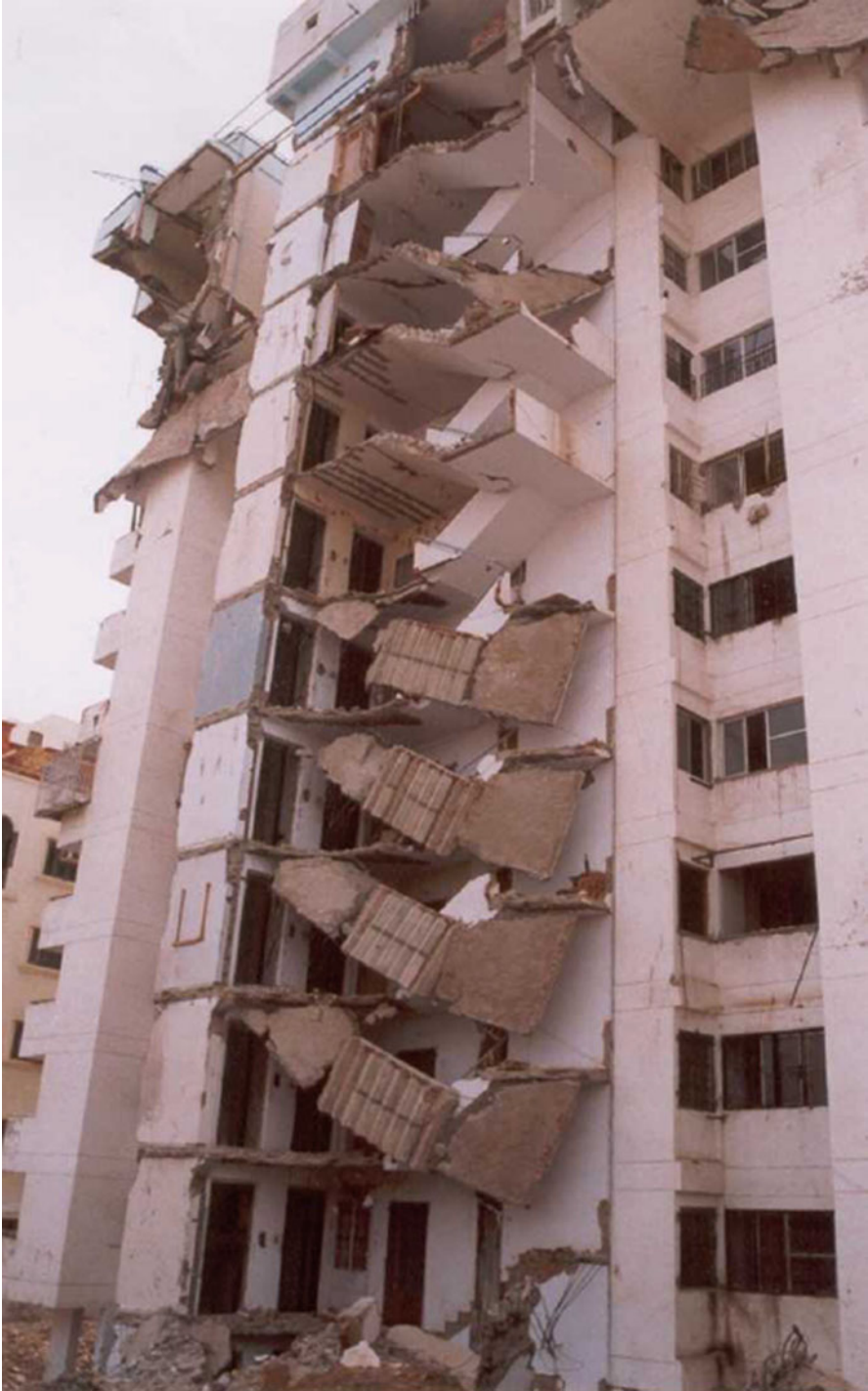
Picture 5.8 Staircase failure
