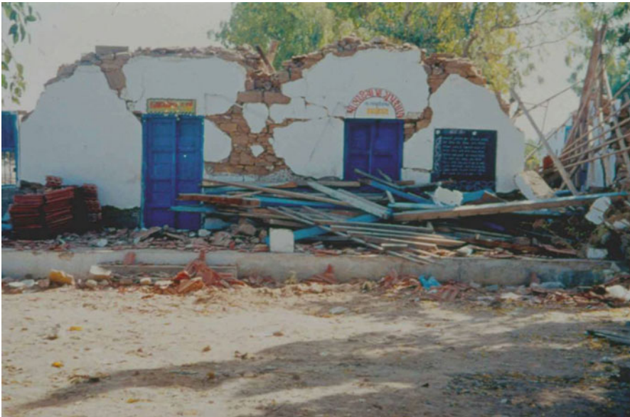
Picture 9.3 Roof slid off the wall
