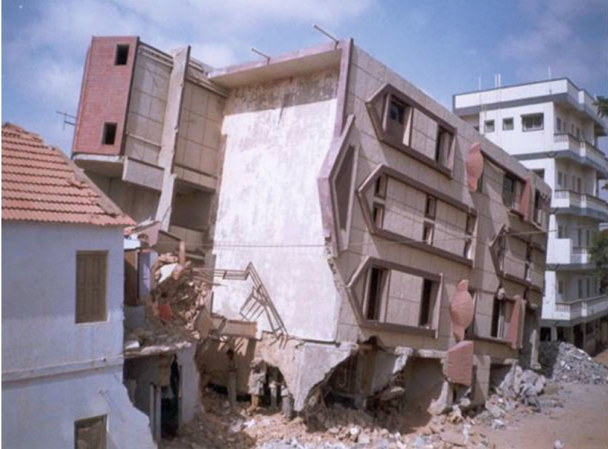
Picture 8.1 Foundation distress
