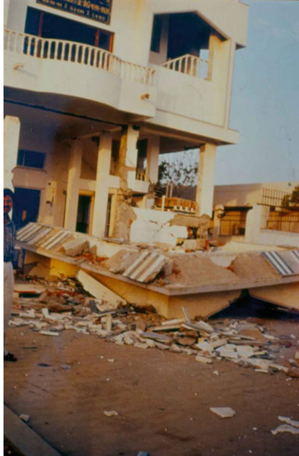
Picture 9.2 Canopy failure
