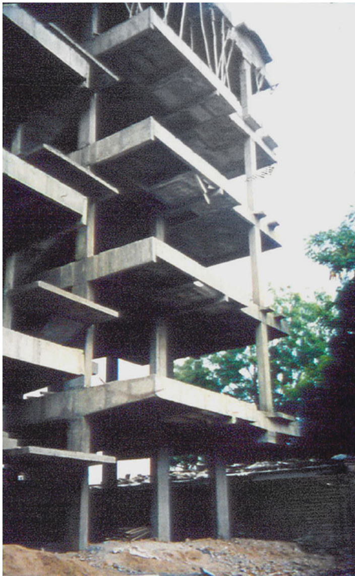
Picture 5.3 Presence of floating columns and columns misaligned
