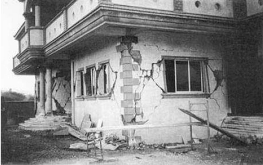
Picture 9.1 Walls not tied together
