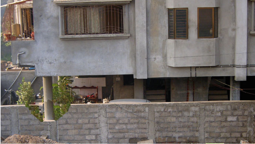
Picture 5.4 Single column supporting heavy load – recipe for distress
