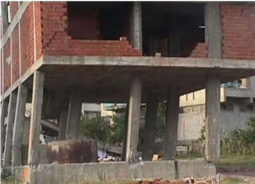
Picture 5.6 Distress due to a soft storey
