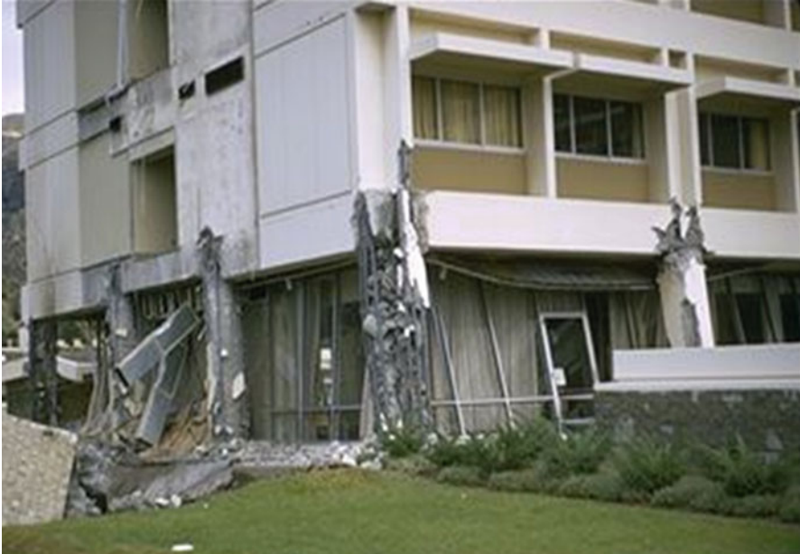
Picture 5.2 Failure of columns supporting end wall
