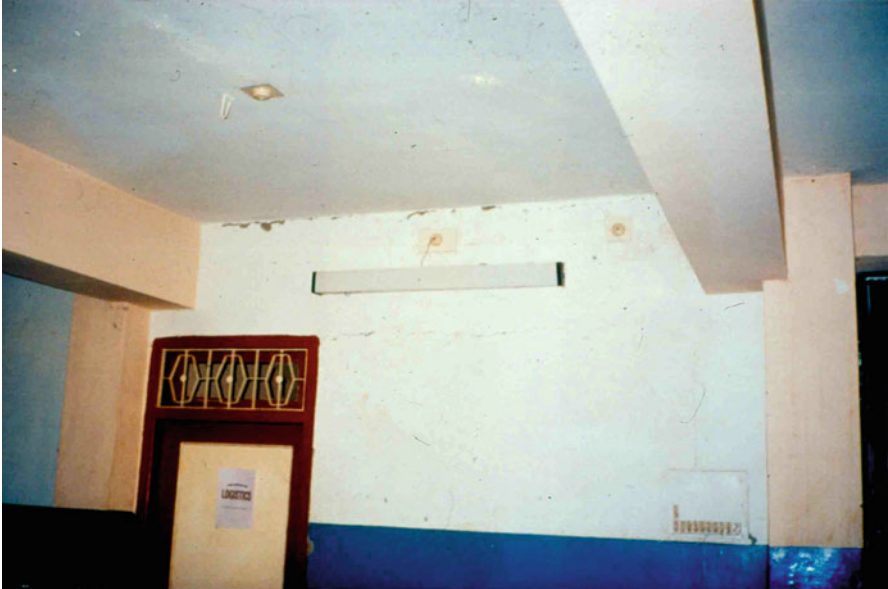
Picture 5.1 Beam and column are not aligned
