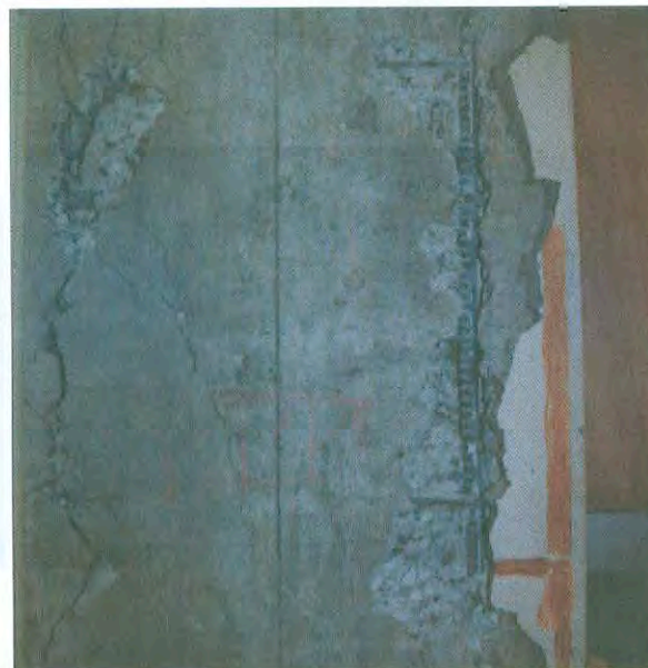
Photo 2-24: Bond splitting cracks were developed along the longitudinal reinforcement in columns of Namioka Hospital, Aomori, in the 1983 Mid-Japan Sea Earthquake; deformed bars were used with round-bar lateral reinforcement; concrete strength was low in this area due to poor coarse aggregates.
