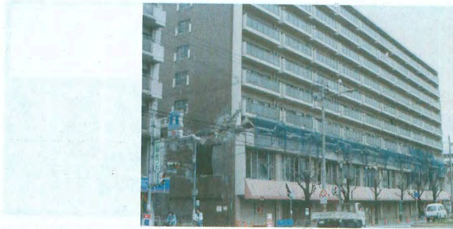
Photo 2-4: Condominium building collapsed in the third storey in the 1995 Hyogo-ken Nanbu (Kobe) Earthquake.
