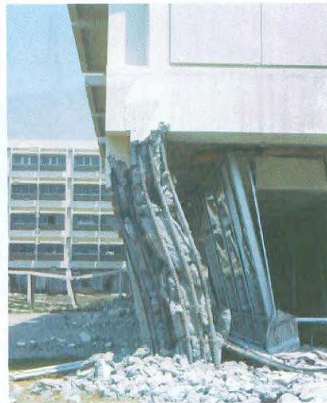
Photo 2- 2: Olive View Hospital, heavily damaged in the ground storey in 1971 San Fernando Earthquake, CA.
