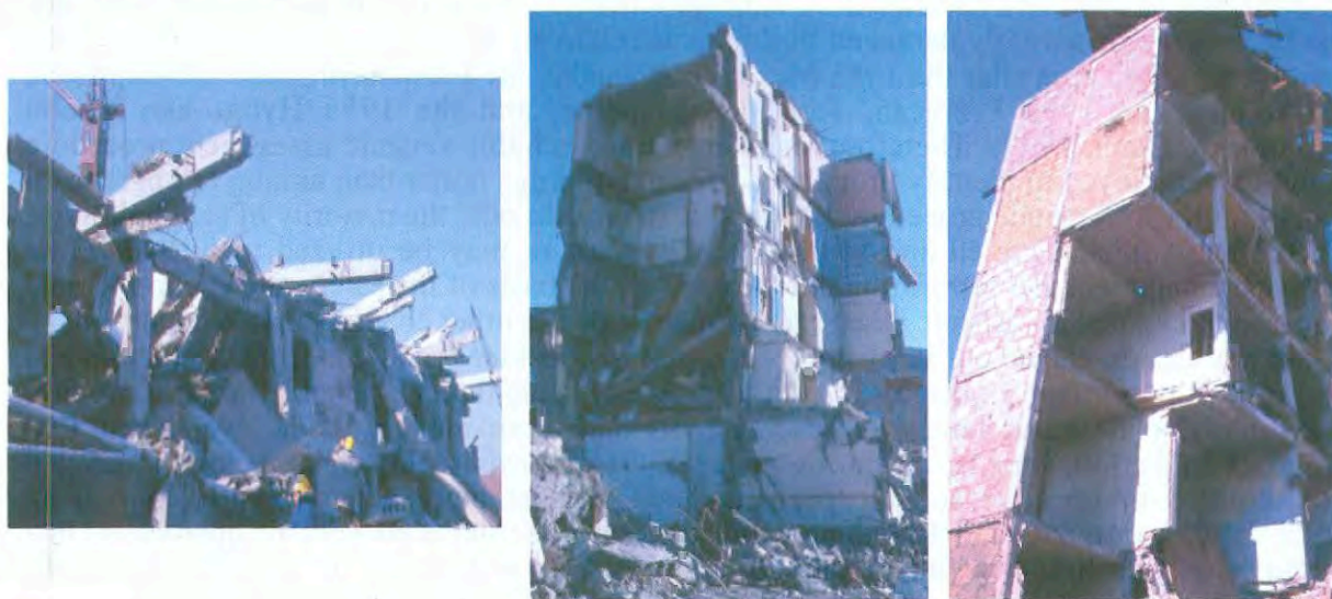
Photo 2-28: Examples of collapse of precast concrete buildings in 1988 Spitak earthquake in Armenia: (Left) Collapse of frame under construction in Leninakan. (Centre) Collapse of building in Spitak composed of wall panels with connections of plain cast-in-situ concrete and hollow-core slabs. (Right) Collapse of building in Leninakan, built of precast and in-situ infilled frame panels
