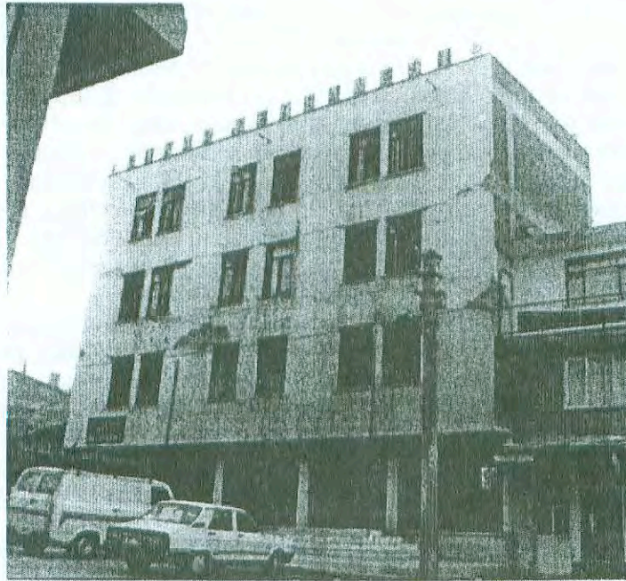
Fig. 7-1: Four storey damaged building in Dinar
