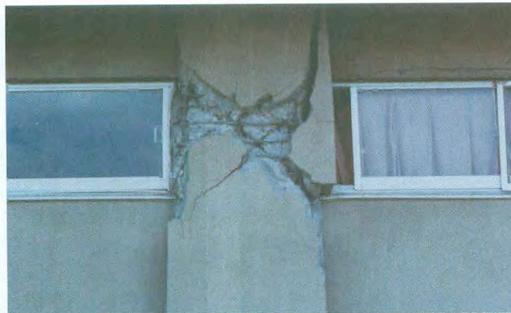
Photo 2-23: In Railway Technical High-school during the 1978 Miyagi-ken Oki Earthquake; non-structural but monolithically cast concrete walls restrained the deformation of a slender reinforced concrete column and caused the lateral deformation to concentrate in a short length
