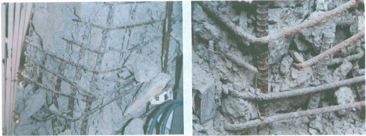
Photo 2-22: Shear failures in columns during the 1995 Hyogo-ken Nanbu earthquake. (Left) Opening of ties at a 90° bend. (Right) Fracture of lateral reinforcement at the corner in a column.
