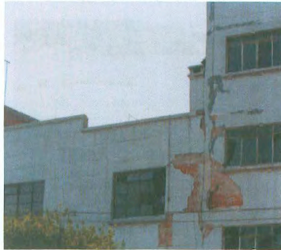
Photo 2-12: Pounding of adjacent buildings in the 1985 Mexico Earthquake
