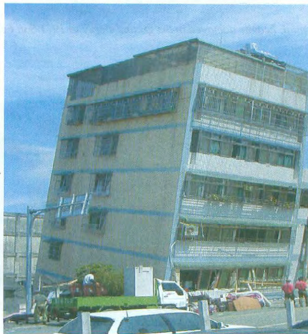
Photo 2-6: First-storey failure of corner building due to torsion in the 1999 Chi Chi Taiwan earthquake. Note open front and wall at the back. Source: NISEE
