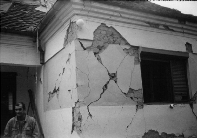
Figure 11. Damage of two store building produced by earthquake.
