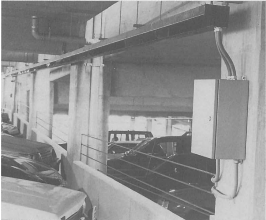
Figure 4-5. CCTV cameras ride along track to improve coverage of parking area. Photo courtesy Video Sentry, Inc.
