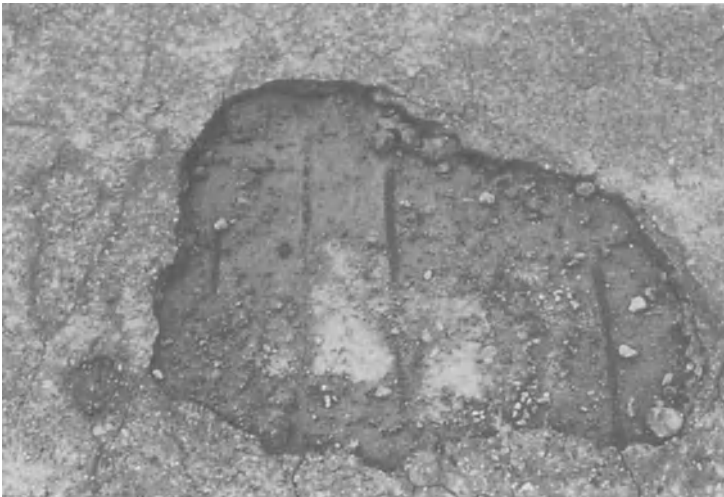
Figure 15-4. Spalling is progressive and steps must be taken to restore and protect the surface from further deterioration.
