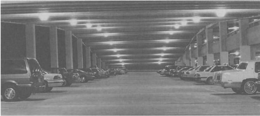
Figure 5-4. Hanging the fixture below the tee stem improves uniformity and vertical illumination but increases potential for glare. Photo courtesy Walker Parking Consultants.
