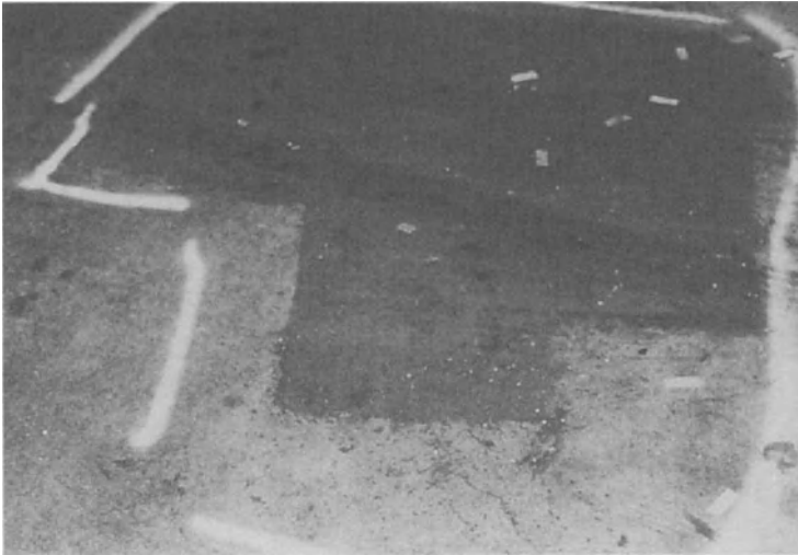
Figure 15-85. Delamination due to continuing corrosion within and beyond patch.
