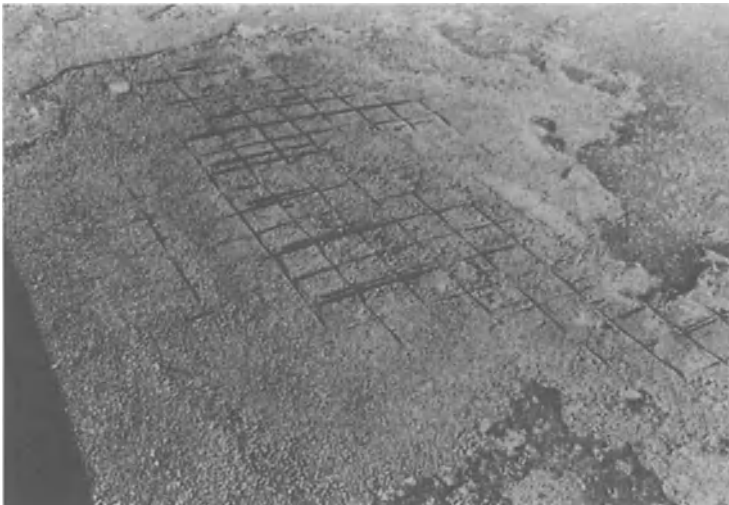
Figure 15-31. Deterioration of non-air-entrained concrete accelerated by poor drainage.
