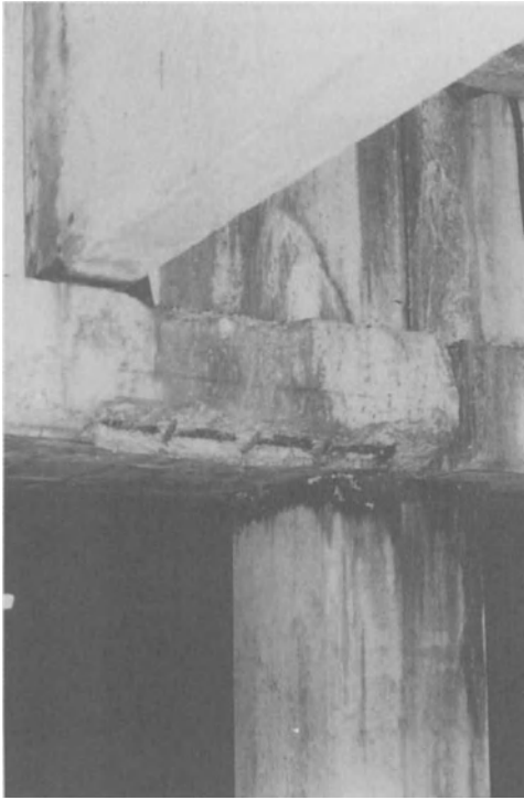
Figure 15-6. Corrosion of reinforcement due to leaching and carbonation of poor quality concrete.
