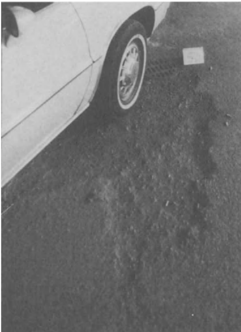
Figure 15-29. Scaling adjacent to drain can contribute to ponding and progressive deterioration of concrete.
