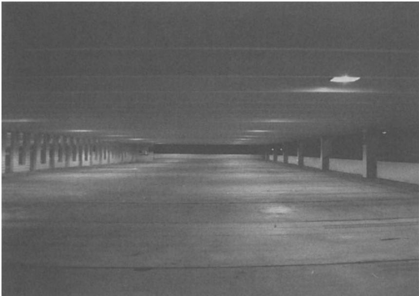
Figure 5-2. Uniformity of illuminance is critical to parking structure lighting. Photo courtesy Quality Lighting, Inc.
