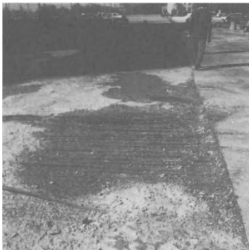
Figure 15-81. Severe deterioration of underlying concrete covered by asphaltic material overlay.
