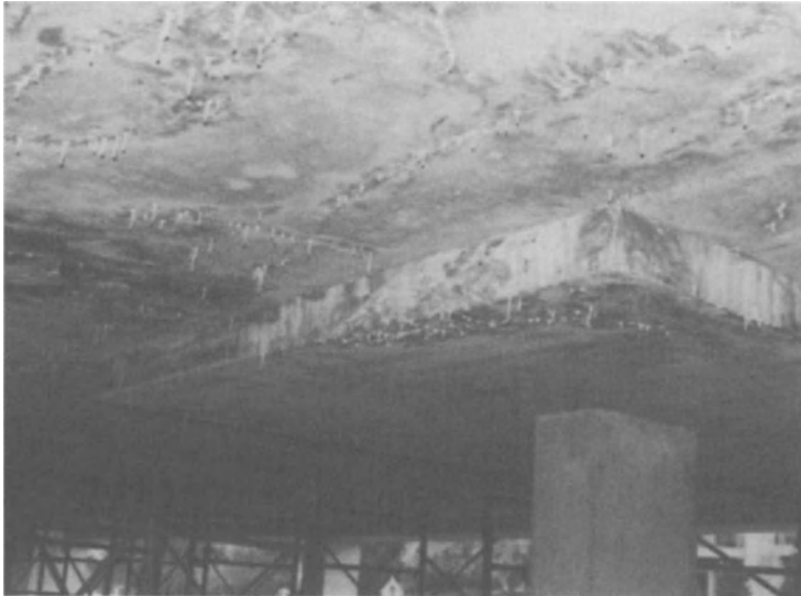
Figure 15-40. Formation of stalactite on slab underside due to continued leaching.
