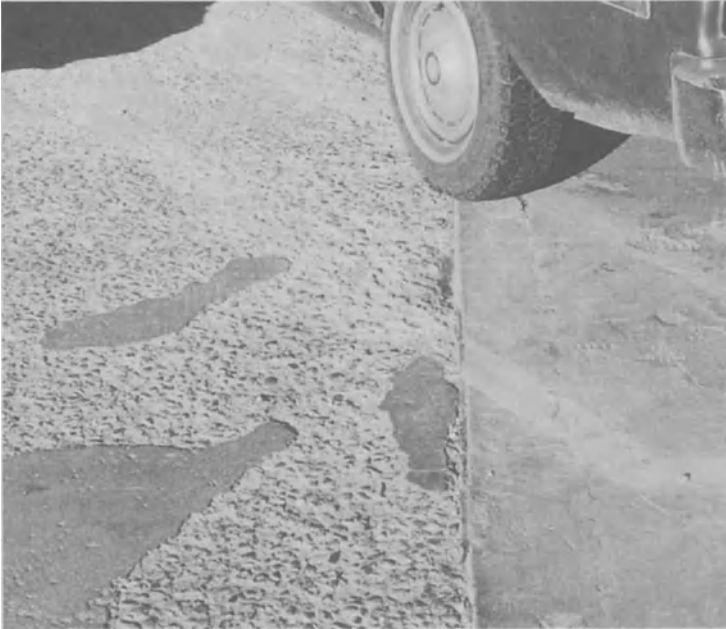
Figure 15-30. Scaling at construction joint.
