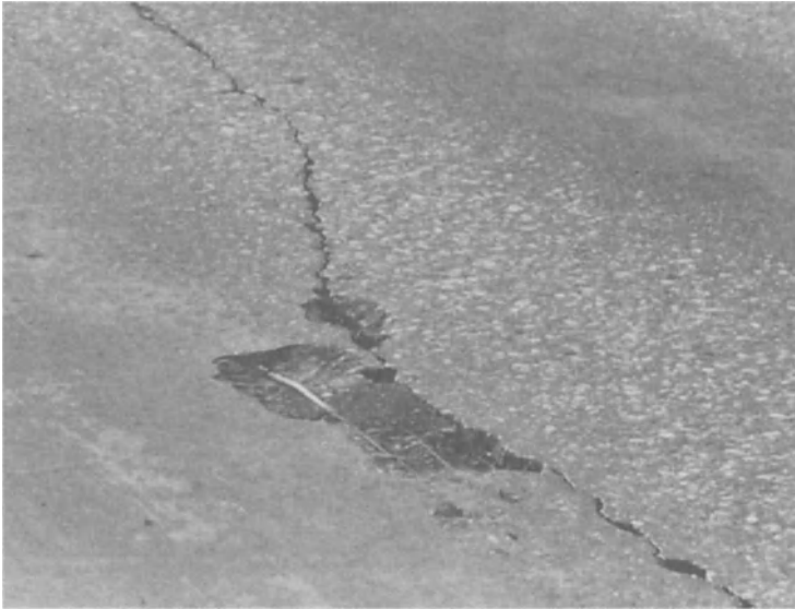
Figure 15-42. Surface abrasion and cracking.
