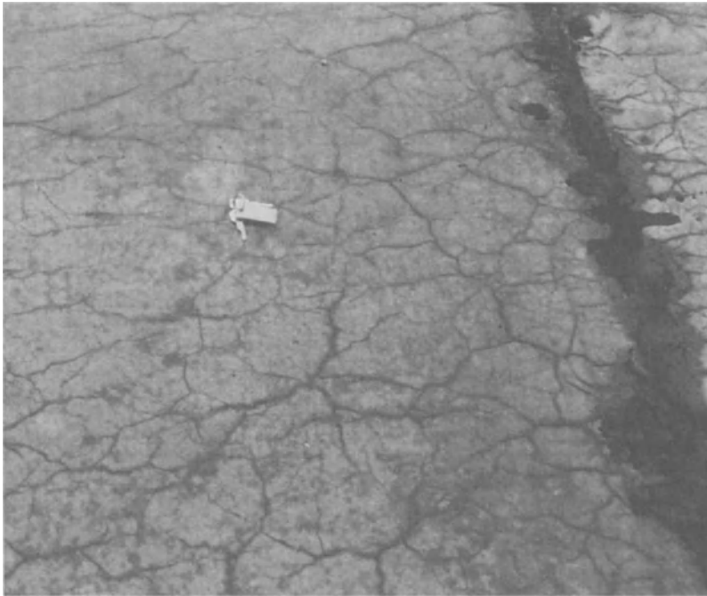
Figure 15-34. Pattern surface cracks on floor slab due to drying shrinkage.
