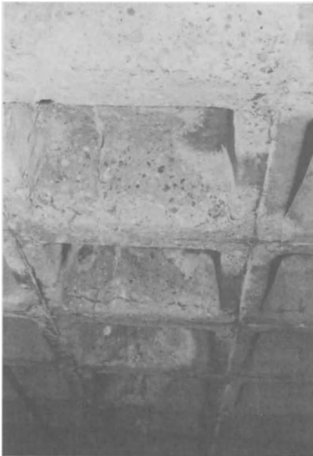
Figure 15-33. Scaling on underside of slab.
