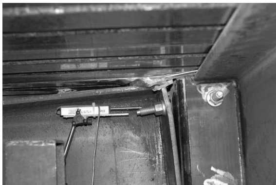
Figure 12: Severe buckle at column face and end plate.
