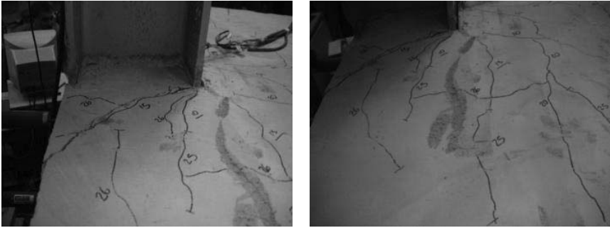
Figure 10: TRSS concrete slab cracking.
