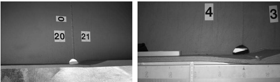
Figure 2: Geometrical imperfections in a large bridge girder, mainly caused by welding distortion.
