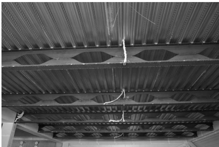
Figure 1: Thermocouples located at the midspan on the castellated beams and its connections
