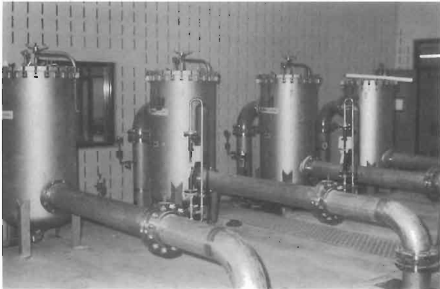
Figure 1. Battery of cartridge filters used for water pretreatment in an RO process.
