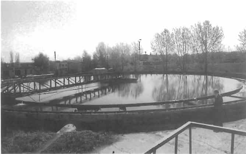
Figure 7. Clarifier used in a wastewater treatment plant.
