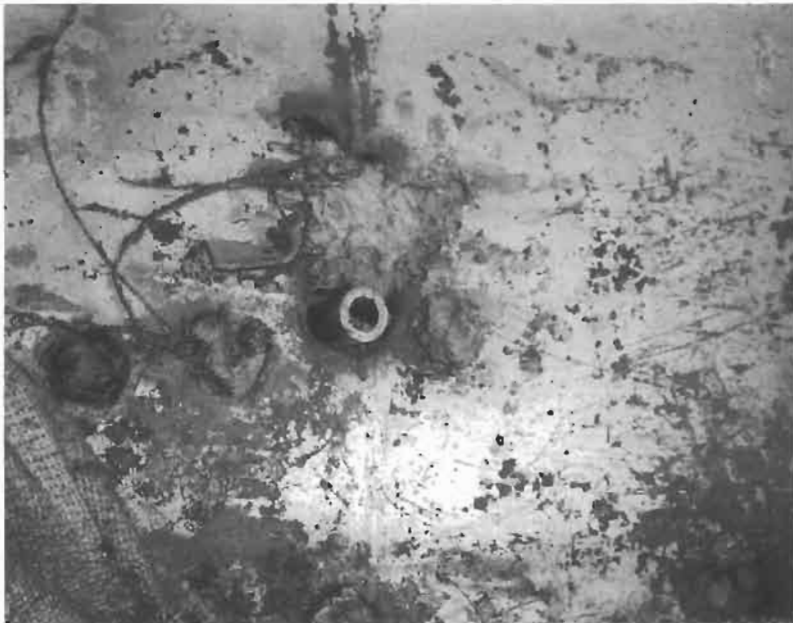
Figure 16. Shows severe pitting and corrosion on the wall of a steel underground storage tank.
