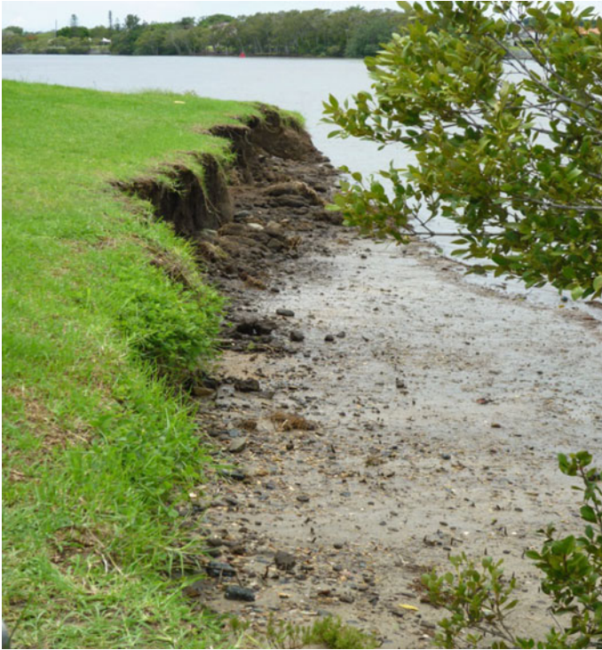
Fig. 1.2 Stream bank erosion due to the increased runoff volume
