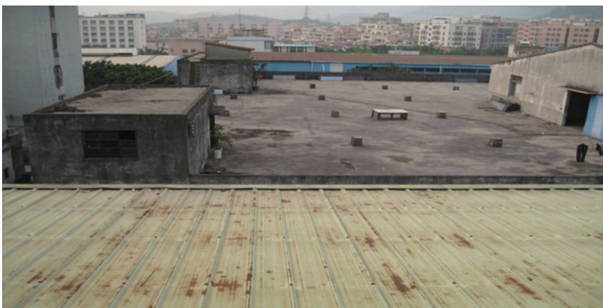
Fig. 1.7 Corroded roof surface
