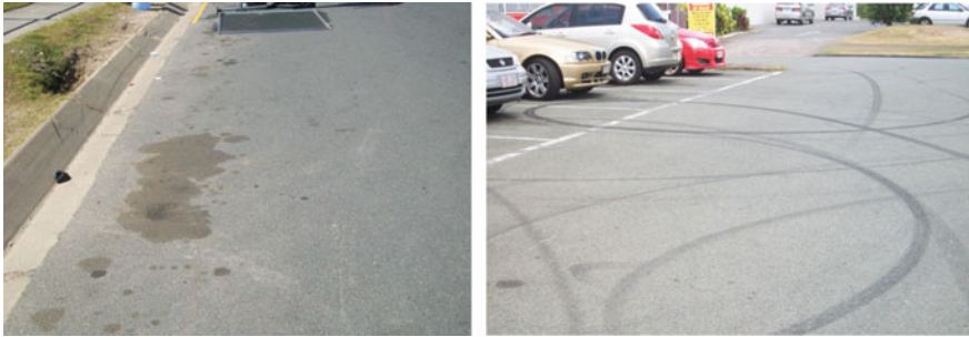
Fig. 1.3 Tyre wear and engine oil leakage on road surfaces
