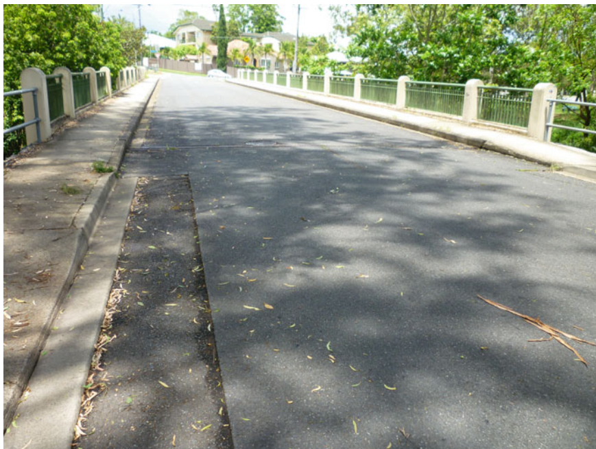
Fig. 1.5 Plant debris on road surface
