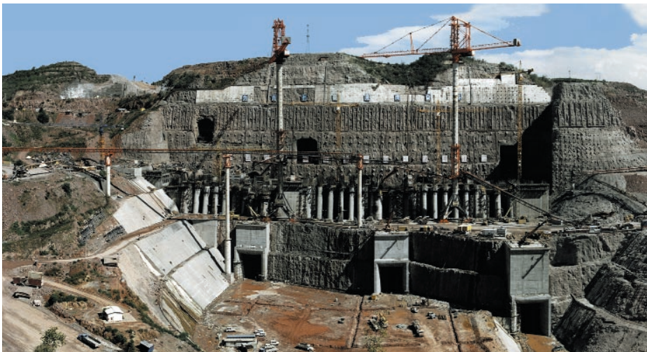
FIGURE 5.3.-2. Intake at Xiaolangdi.
