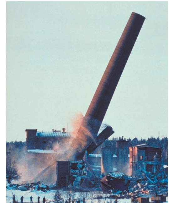
FIGURE 5.2.17. Old, 15 m in diameter, 92 meter high chimney was blasted down on February, 1998, at Imatra, Finland.
