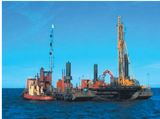
FIGURE 5.2.-15. The Kokkola Channel. The project was to increase the nautical depth of the access channel from 11 meters to 13 meters over a length of 18 km. This involved dredging approximately 2 million m 3 . Dredging activities began in September 1995 and will be completed at the end of July, 1998. Upon completion, the Kokkola Channel be-come one of Finland's five deepest channels. The total excavation of granite was 66.500 m 3 and total area to be pre-treated by blasting is 150 000 m 2 . Almost 15,000 holes between 3 - 4 meters (most holes 115 mm in diameter) were drilled. Tamrock's rock drill and a power pack are used in this project on drill mast constructed by the contractor.
