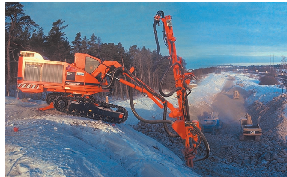
FIGURE 5.3.-1. Typical view of railroad construction site - TAMROCK Ranger 700 working a bench drilling project in Sweden. The Arlanda Rail link connection between downtown Stockholm and the Arlanda airport will cut the duration of the trip from 35-50 minutes to 19 minutes. The rail system will be ready in autumn 1998. This work site consists of many open-bench excavation and tunneling projects. The project has a total of 8.6 km of tunnels and three stations beneath the airport. Rock type varies from mica schist to granodiorite. Hole sizes are 32-102 mm depending on the scale of excavation. Bench heights are 10-15 meters in the typical highway or railway cutting project.
