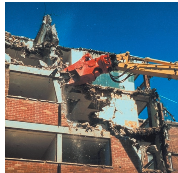
FIGURE 5.3.-4. An English demolition contractor, CDC Demolition Ltd., from Woodbridge, Suffolk, pulled down a 14-floor apartment building in Bristol. CDC used an RC 22 cutter crusher with a digging machine for this project. The first phase included pulling down the upper five floors with two 3-ton mini-diggers that were rented from the David Meek Plant. Both machines were equipped with Rammer hammers: S 22 and S 22 CITY. Immediately after the completion of the first phase the RC 22 continued the demolition and pulled down the rest of the building.
