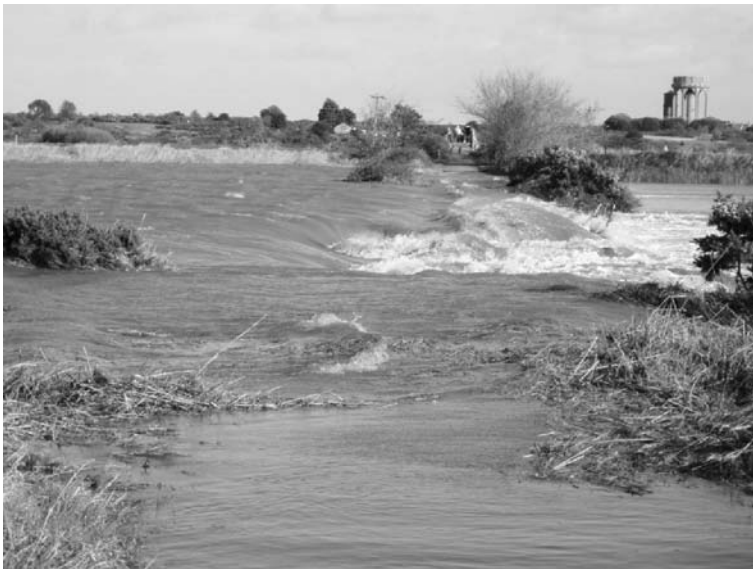
Figure 5.3 Breached embankment and footpath, Bailey Bridge Footpath, Walberswick, Suffolk, UK, arising from a combination of high tides and torrential rainfall in November 2007 (courtesy of Halcrow Group Ltd).
