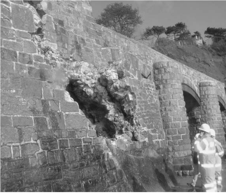
Figure 7.6 View of the damaged wall from the seaward side, showing removal of stone blocks and pointwork (courtesy of Network Rail).
