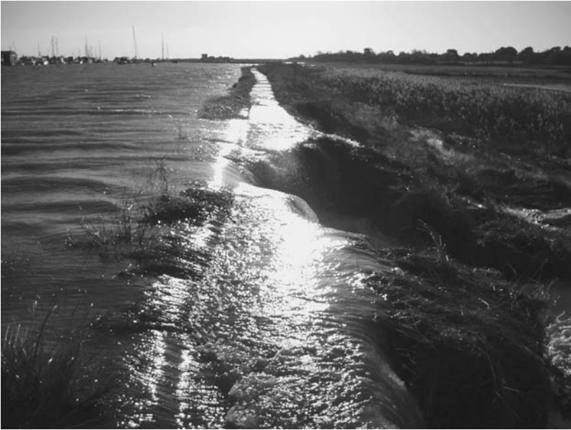
Figure 6.3 Overflow of Robinson's Marsh embankment, Suffolk, UK. Erosion of the backface of the embankment is evident and is a precursor of the formation of a breach (courtesy Halcrow Group Ltd).
