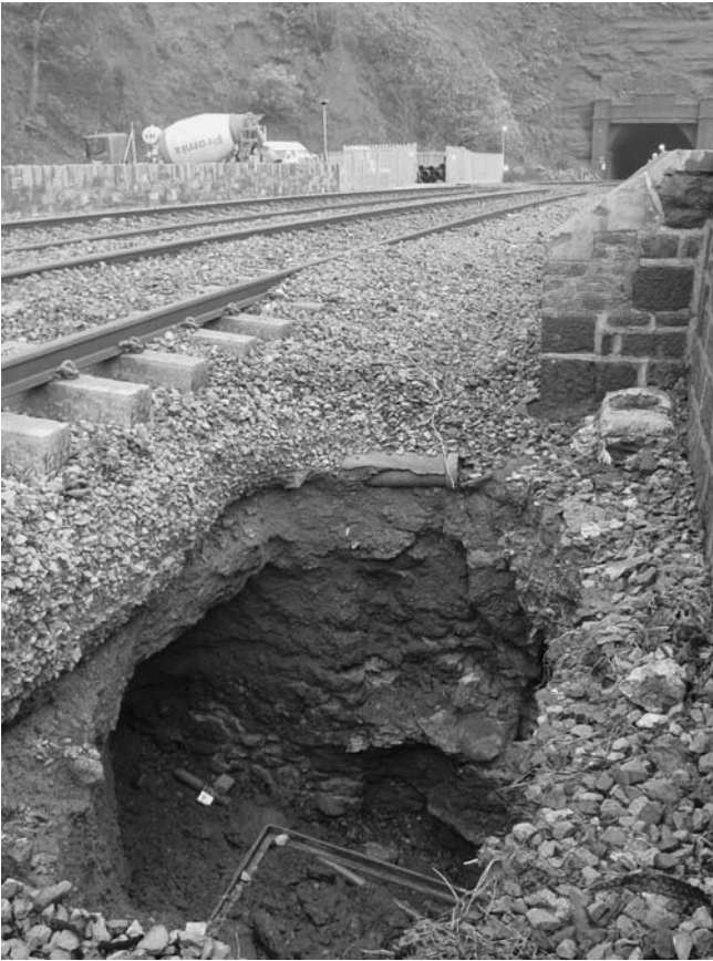
Figure 7.5 Erosion of material between the rail track and wave wall as a result of severe storm action (courtesy of Network Rail).
