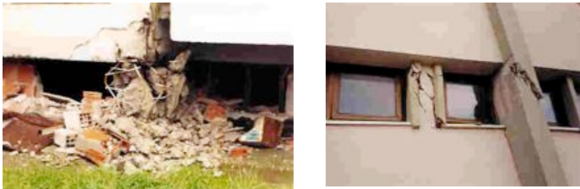
Fig. 4: Damaged short columns due to insufficient shear strength (1999 earthquakes in Duzce and Kocaeli)
