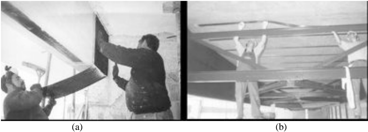
Fig. 3: (a) Hand lay-up of CFRP sheets or fabrics. (b) Application of prefabricated strips.
