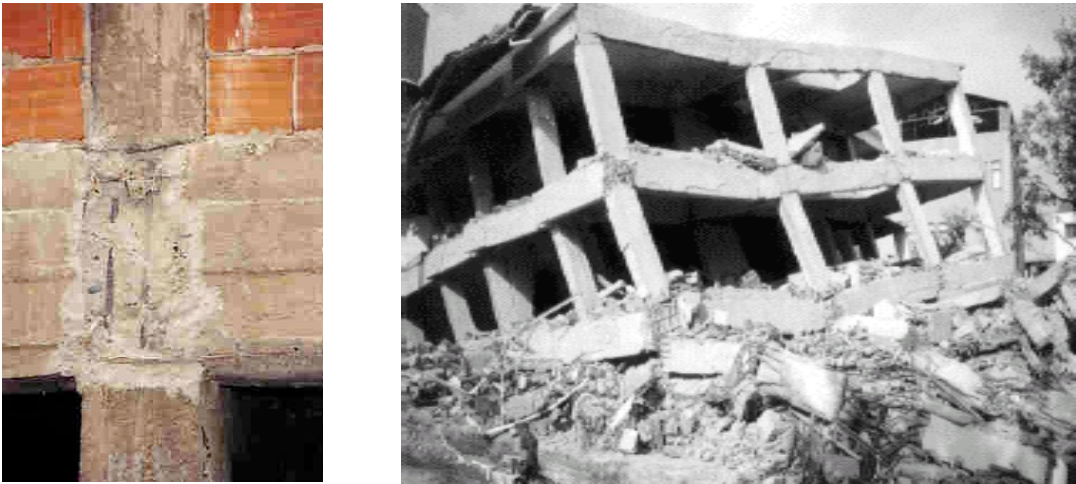
Fig. 7: Failure of beam-column joints
