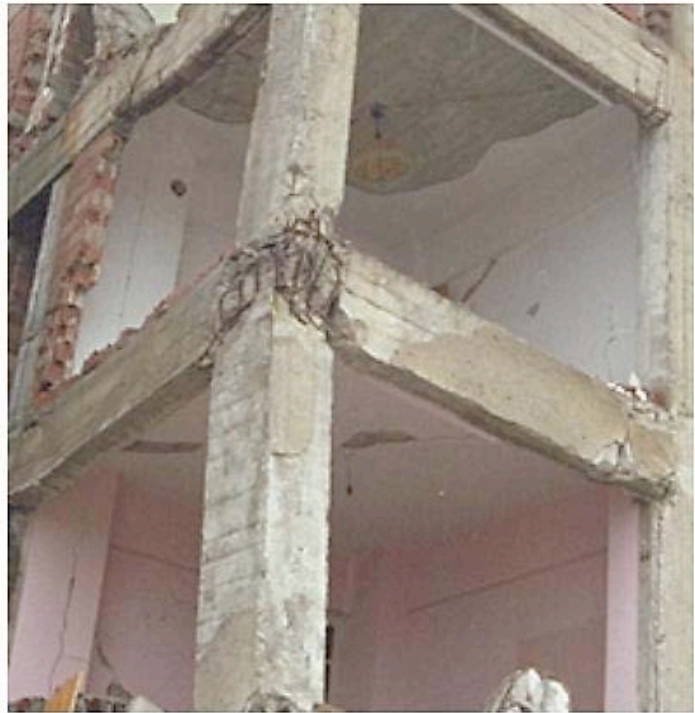
b) Detailed view of beam-column joint damage
