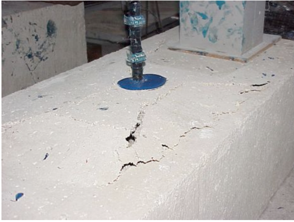
Fig. 13: Pullout failure of CFRP anchor
