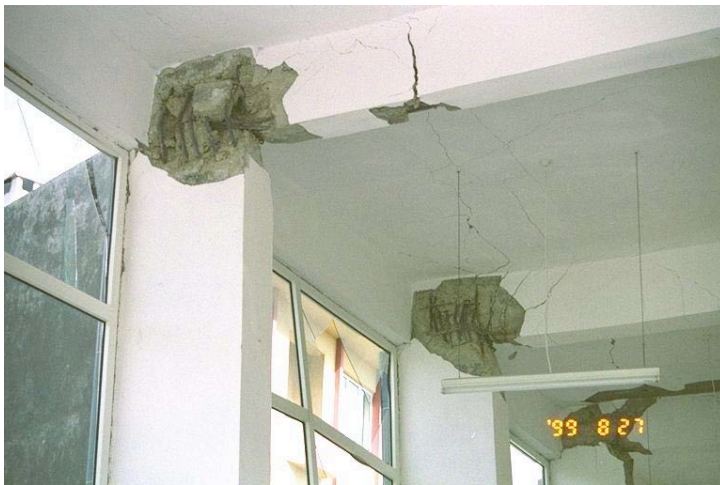
Fig. 4: Damage to a new RC moment-frame beam-column joints in 1999 Kocaeli earthquake [Sezen et al., 2000]
