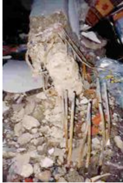
Fig. 22: Damage due to lap splice deficiency in Kaynasli (Duzce earthquake 1999)
