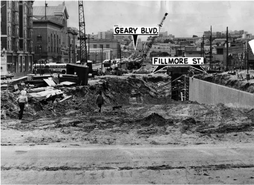
Figure 6.1 First construction in Western Addition Redevelopment area widening Geary Street and directing it into an underpass at Fillmore Street, 1960. Photo of east end of tunnel was taken from Buchanan Street. Just above tunnel entrance is Fillmore Street. San Francisco History Center, San Francisco Public Library.
