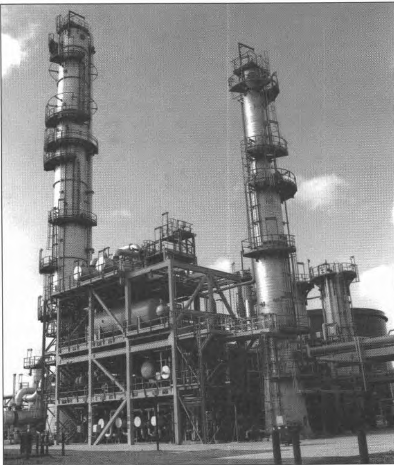
Isomerisation Unit at Elf / Murco / Gulf Refinery, Milford Haven, Wales, showing the deisohexanizer.
