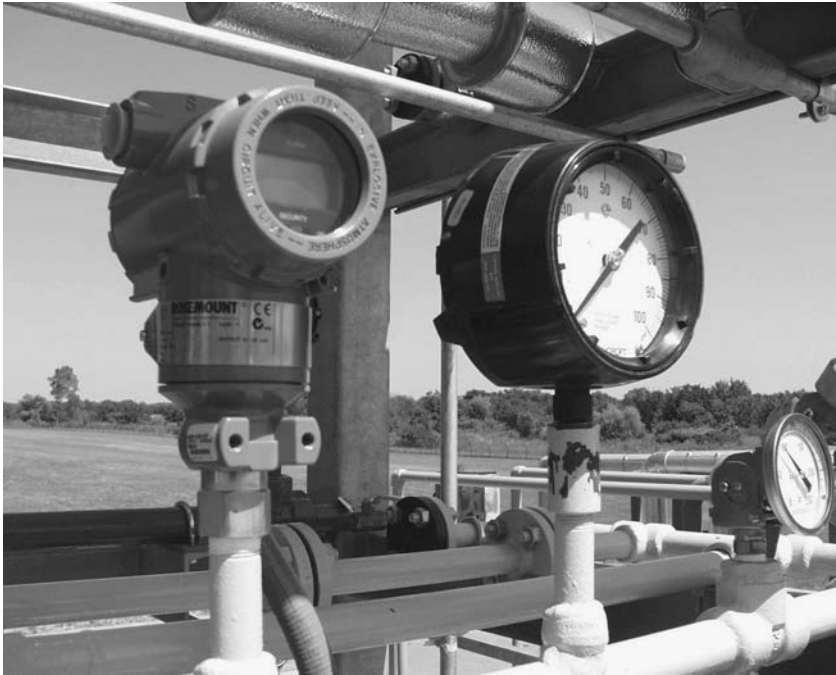
FIGURE 8.18 Pressure transmitter (left) and pressure gauge (right).
