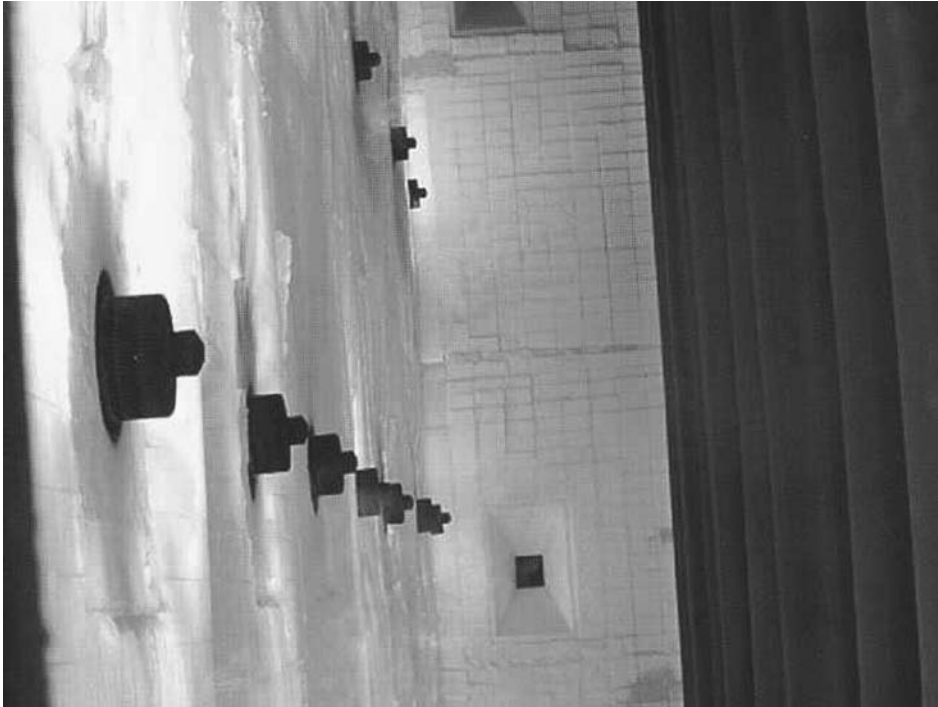
FIGURE 15.4 Forced-draft radiant wall burners in an ethylene-cracking furnace. (Courtesy of John Zink Co., LLC.)
