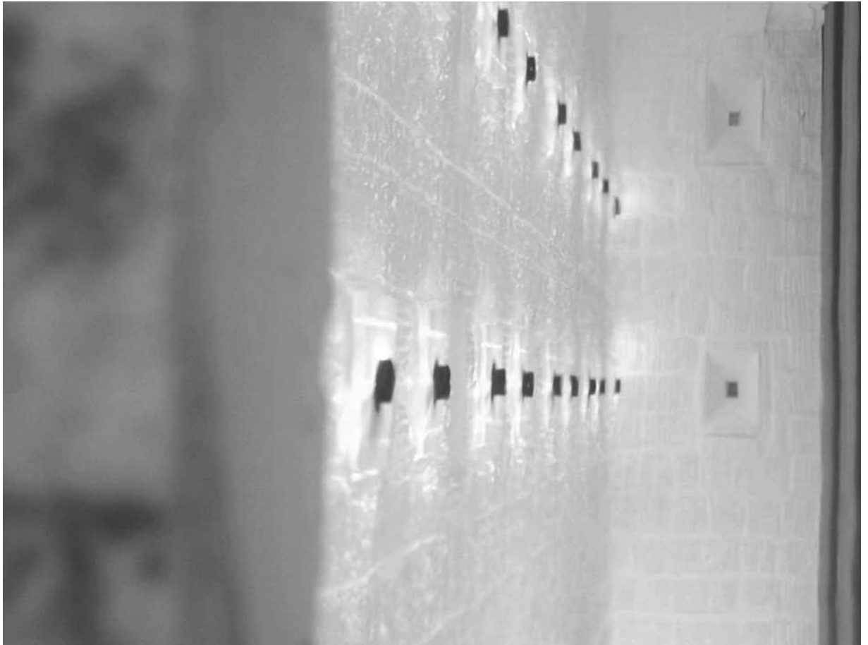
FIGURE 15.1 Radiant wall burners (natural draft) firing in an ethylene-cracking furnace. (Courtesy of John Zink Co., LLC.)
