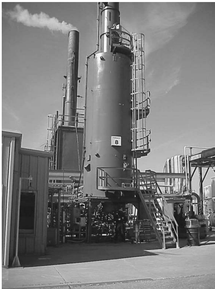
FIGURE 9.4 Test furnace for simulation of upfired tests. (Courtesy of John Zink Co., LLC. 21 )
