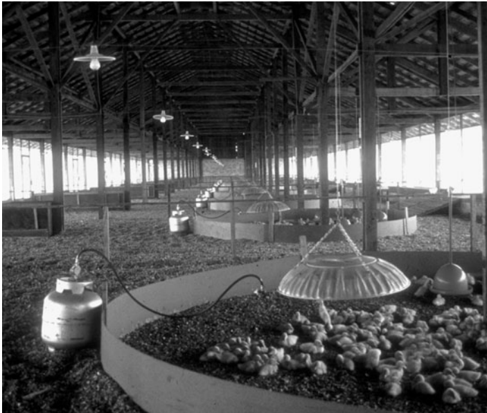
Fig. 3.17. Intensive naturally ventilated brooding accommodation.
