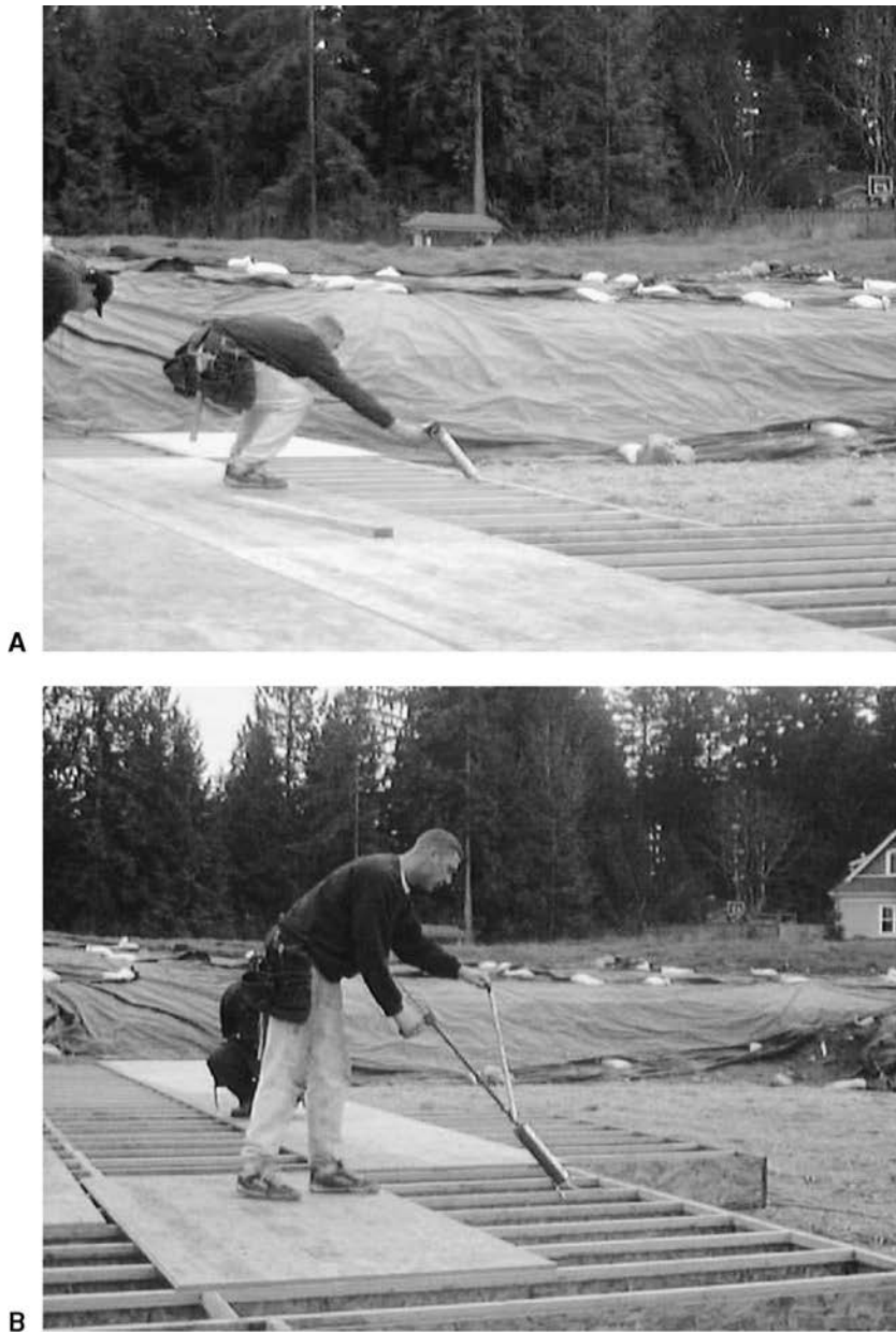
FIGURE 23-5 ● (A) Traditional method of applying glue to floor joists. (B) New method using commercially available extended gun ($50 retail). A handle was added to the gun to reduce hand/wrist fatigue (parts less than $10). Job times were the same for each of the two methods. (Photographs by Barbara Silverstein.)
