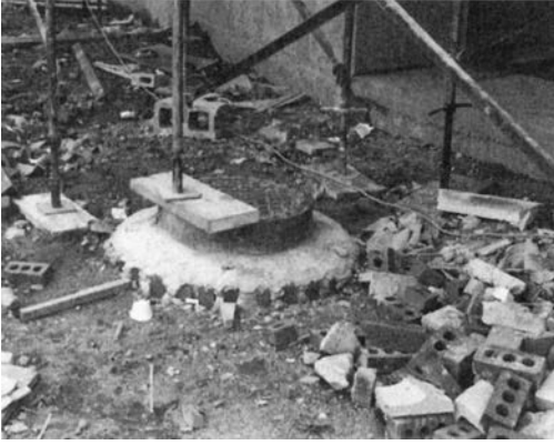
FIGURE 22-2 ● Example of poor housekeeping on a construction site. Loose bricks, lumber, and other debris create a potential tripping hazard for workers.
