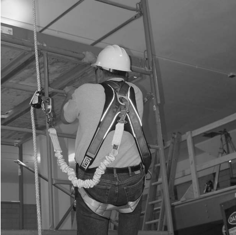
FIGURE 22-5 ● Worker wearing a full-body harness with attached lanyard (Photograph courtesy of the Construction Safety Council.)
