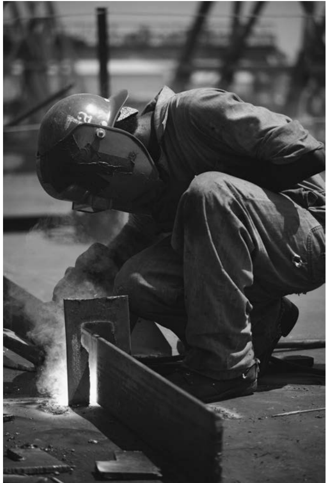
FIGURE 22-4 • Example of worker using multiple forms of personal protective equipment: hard hat to minimize and protect the worker's head from falling objects; a shield and safety glasses to protect the worker's face and eyes from flying particles and damaging irradiation; and gloves to protect the worker's hands from burns, cuts, and flying particles. (Source: Photo Disc, Inc.)
