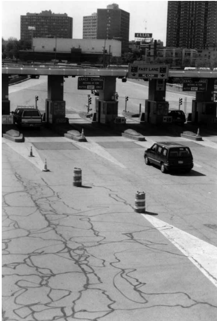
Plate 22 The fast lane on the Massachusetts turnpike in Boston: a classic example of the use of information technology to support local infrastructural bypass and the construction of a premium network space. Cars equipped with transponders enter the tolled highway without stopping. Tolls are electronically debited from users' bank accounts. Photograph: Stephen Graham
