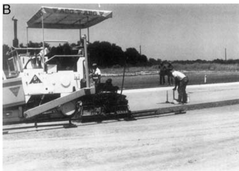
FIGURE 12.3 Static nuclear density gauges in use during construction of (A) conventional PCC pavement 19 and (B) roller-compacted concrete. 11 (A, Photo courtesy of FHWA; B, Photo courtesy of Kirby T. Meyer, P.E. Austin, TX. Reprinted with permission from Malisch, W.R., Conc. Constr. , 33, 13, 1988.)
