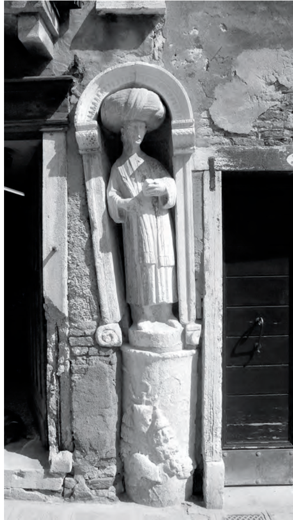
FIG. 147 The slow collapse of the stones of Venice in the Campo dei Mori. Photo by Raoul Mörchen.
