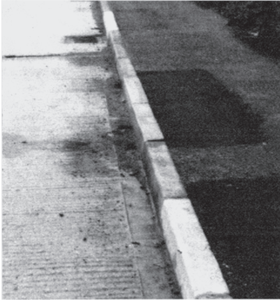
Fig. 8.18. Defective kerbs with only partial replacement.
