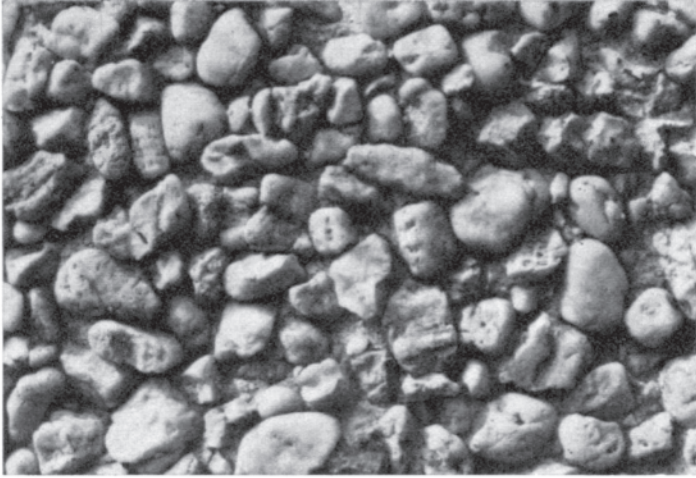
Fig. 6.8. Over-exposed aggregate finish.
