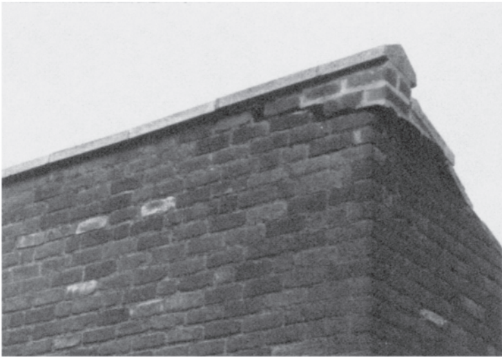
Fig. 8.22. Sulphate attack on concrete coping causing expansion.
