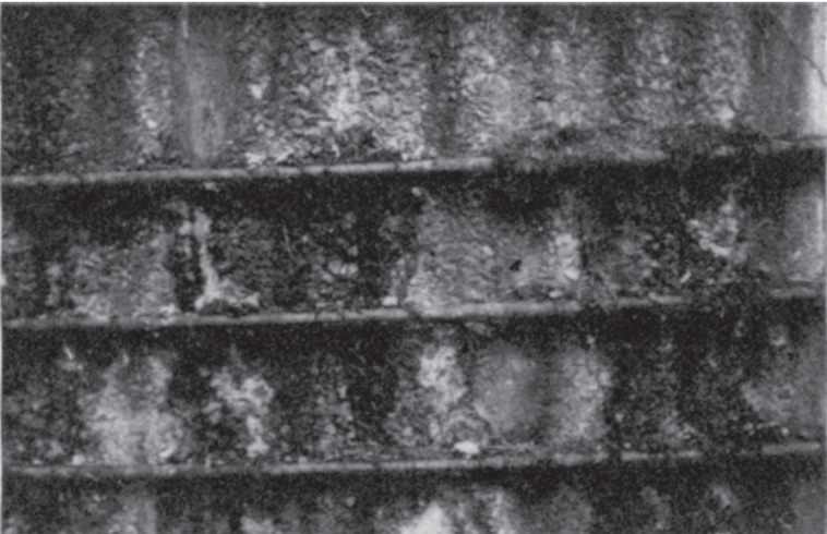
Fig. 8.24. Effect of grass silo acid on concrete surface.
