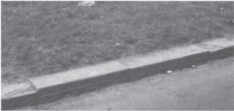
Fig. 8.7. Badly bedded kerbs.
