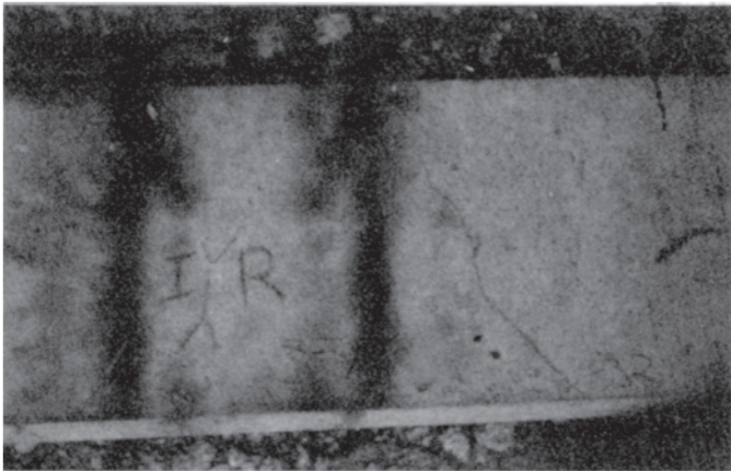
Fig. 10.2. Cracked and re-cracked reinforced concrete beam repaired twice.
