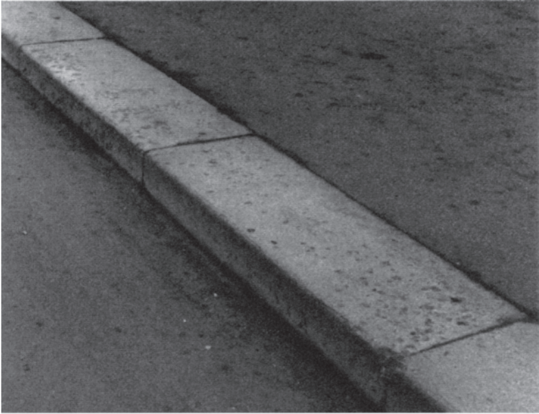
Fig. 8.19. De-icing salt surface spalling—kerbs.
