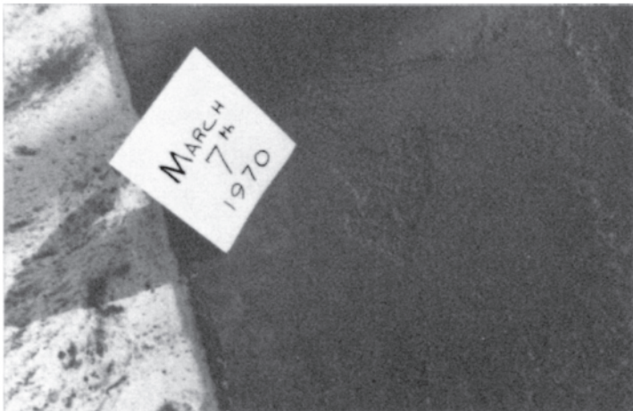
Fig. 8.20. De-icing salt spalling—paving slab.
