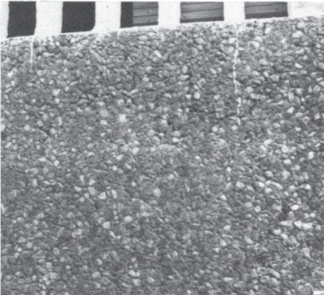
Fig. 6.5. High coarse/fines ratio in exposed aggregate work.
