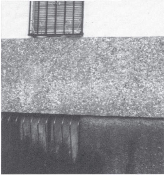
Fig. 6.4. High coarse/fines ratio in exposed aggregate work.
