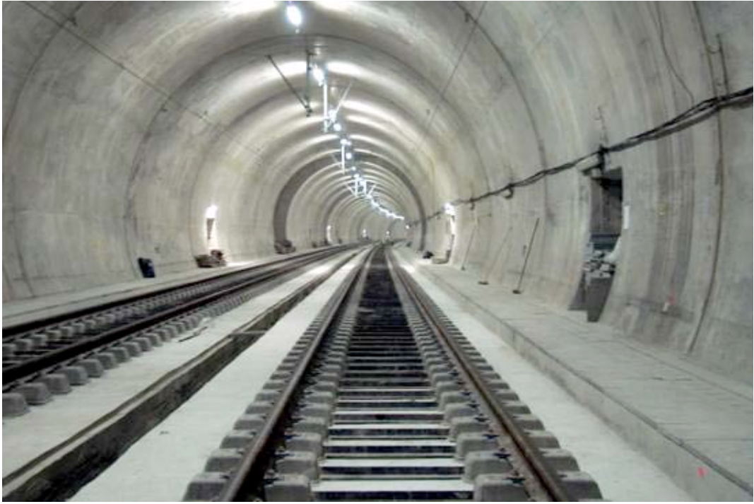
Figure 2-4: Slab track in tunnel, Reseau Ferre de France, Marseille tunnel high speed line (2003)
