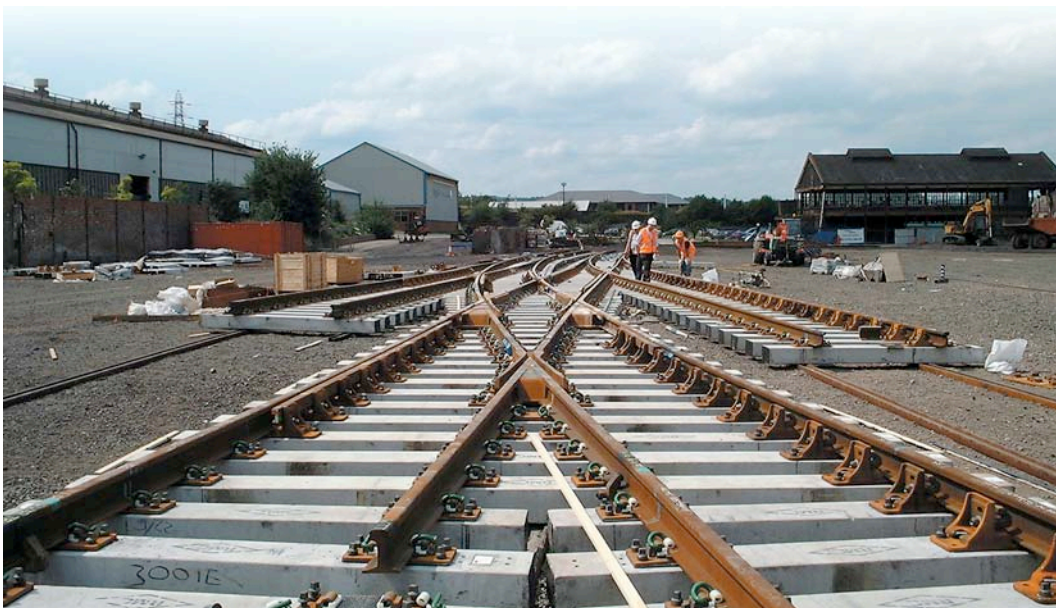
Figure 2-3: Trial assembly of crossover before installation, Balfour Beatty Rail Products, Sandiacre, UK (2004)
