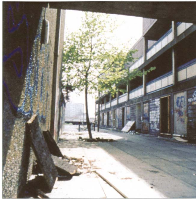
Decline through neglect: deck access blocks in Hulme, Manchester prior to demolition (English Partnerships)
