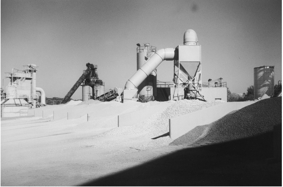
Plate 6.9 Knockout box primary dust collector (upper right).
