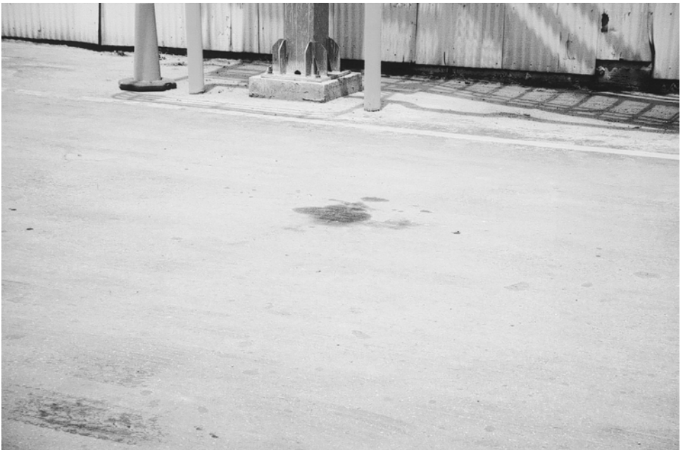
Plate 8.4 Moderate oil spillage damage.
