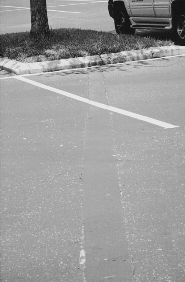
Plate 8.18 Utility cut patch.
