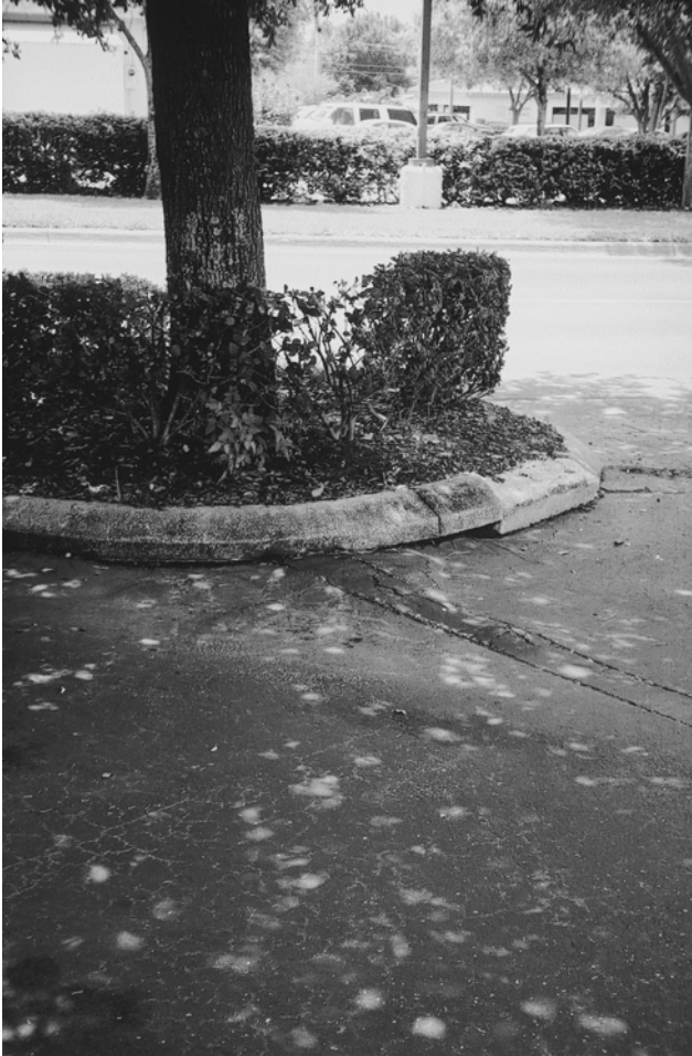
Plate 8.11 Distortion caused by a tree root.
