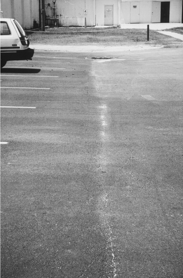
Plate 8.17 Water induced longitudinal crack.
