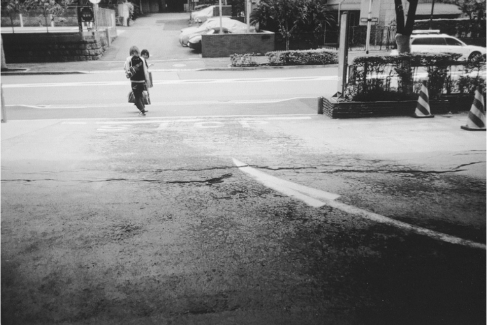
Plate 8.21 Spalled transverse crack.
