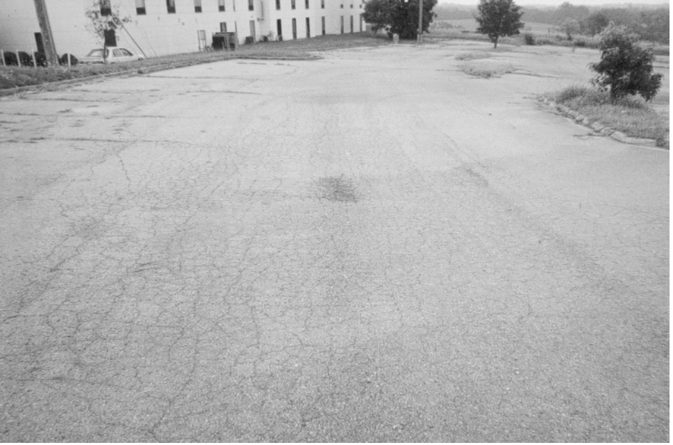
Plate 8.26 Medium to severe alligator cracking.
