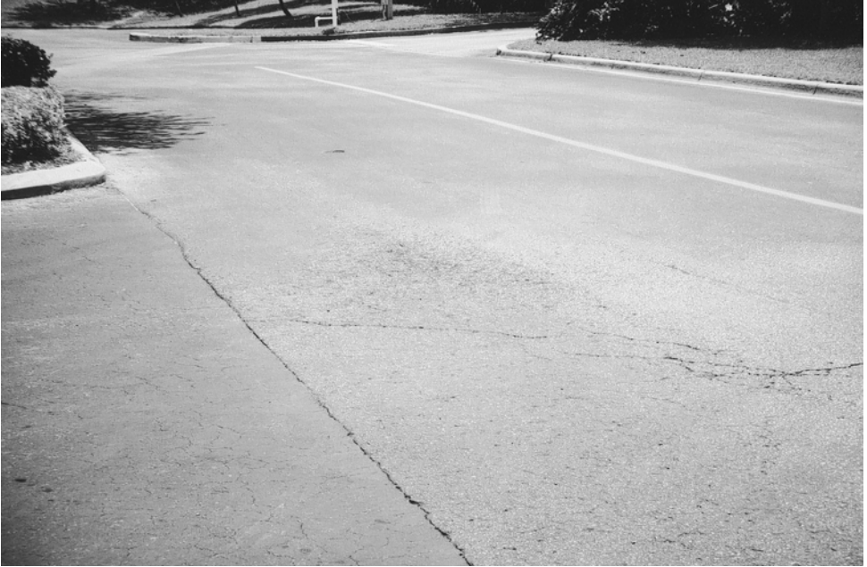
Plate 8.7 Wheelpath raveling and alligator cracking.
