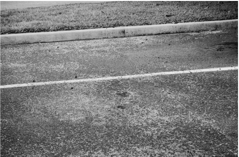
Plate 8.6 Raveling due to stripping.
