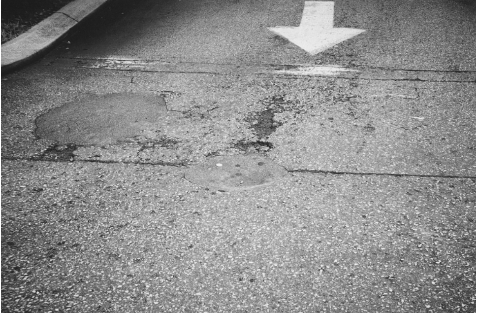
Plate 8.3/ Transverse crack and pothole.
