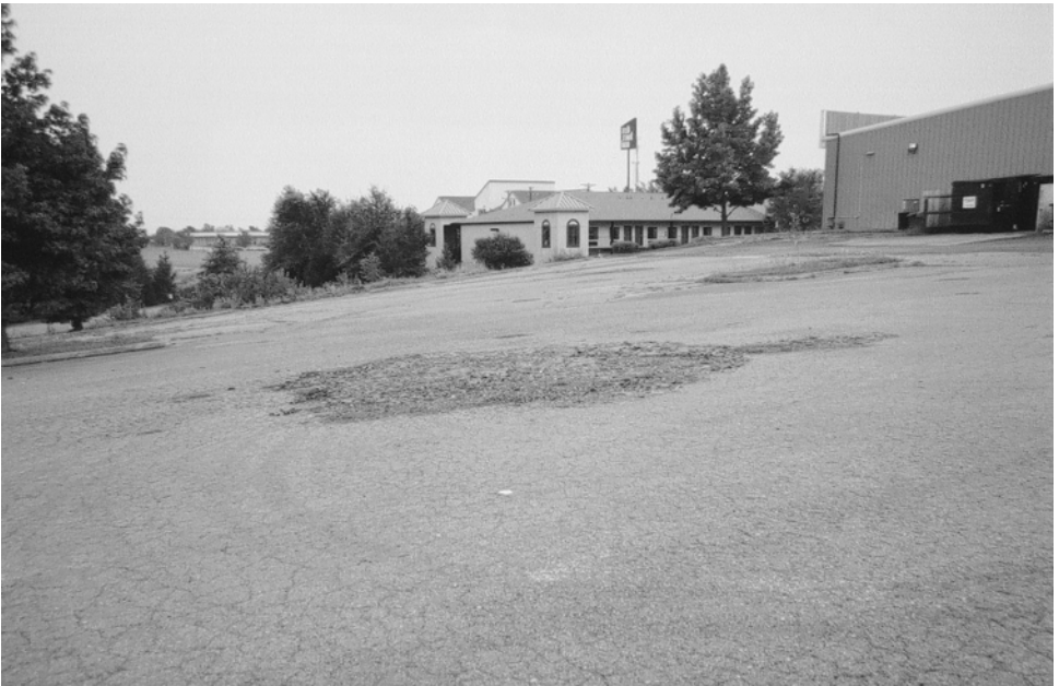
Plate 8.27 Severe alligator cracking.
