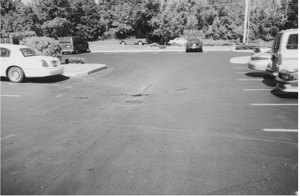
Plate 8.29 Water induced pothole.
