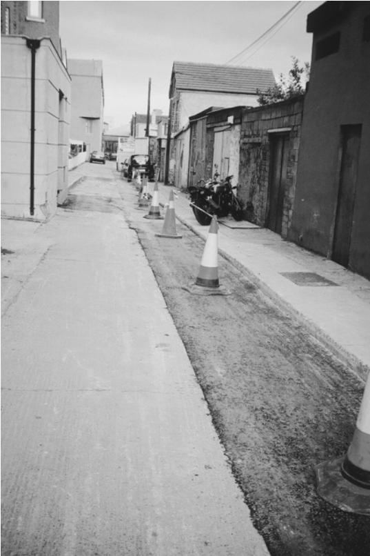
Plate 9.2 Utility cut patch.
