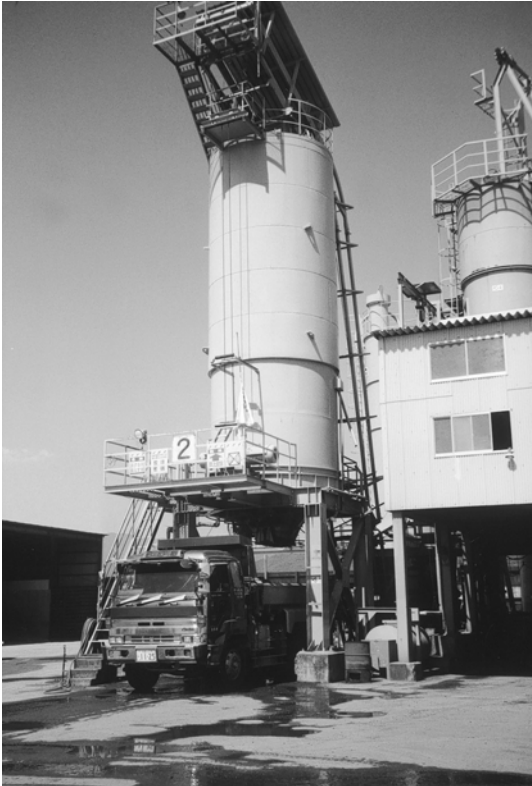
Plate 6.5 HMA storage silo.
