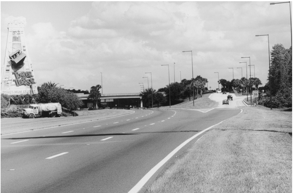
Plate 8.9 Low severity rutting.
