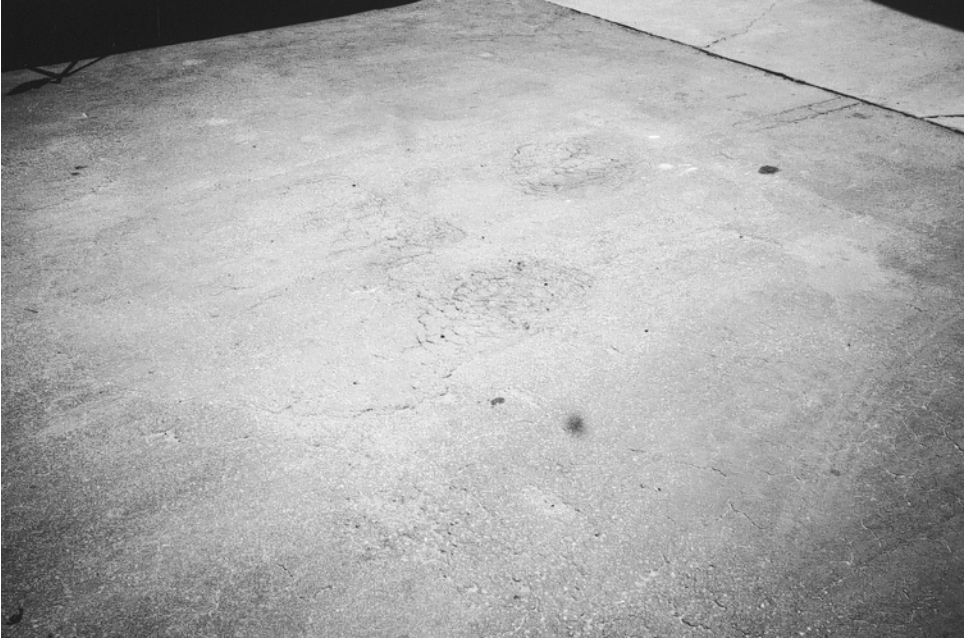
Plate 8.25 Alligator cracking beginning to form a pothole.
