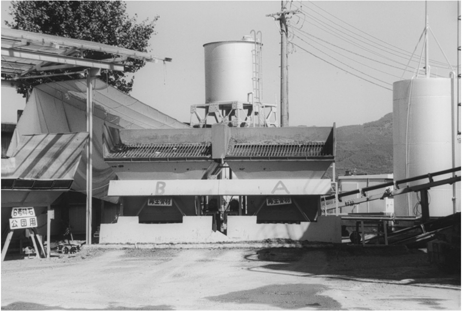
Plate 6.8 RAP feed bin.
