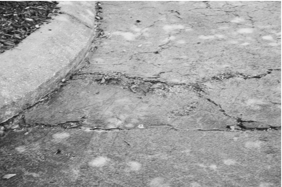
Plate 8.30 Rupture and pothole.
