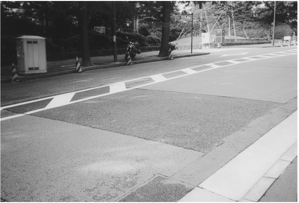
Plate 9.1 Pavement distress patch.
