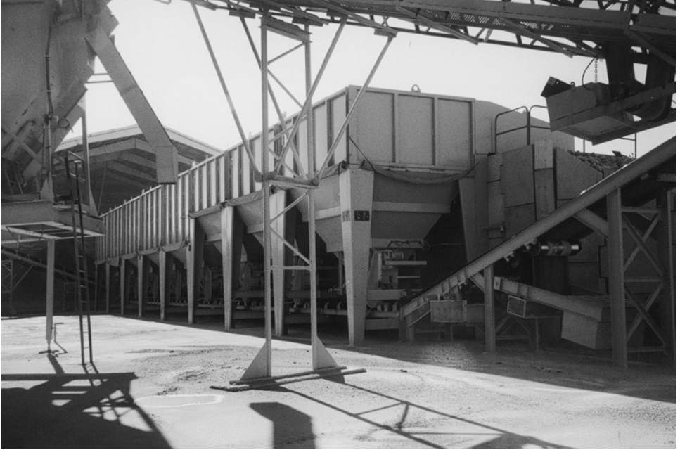
Plate 6.10 Large cold feed system for a drum mix plant.
