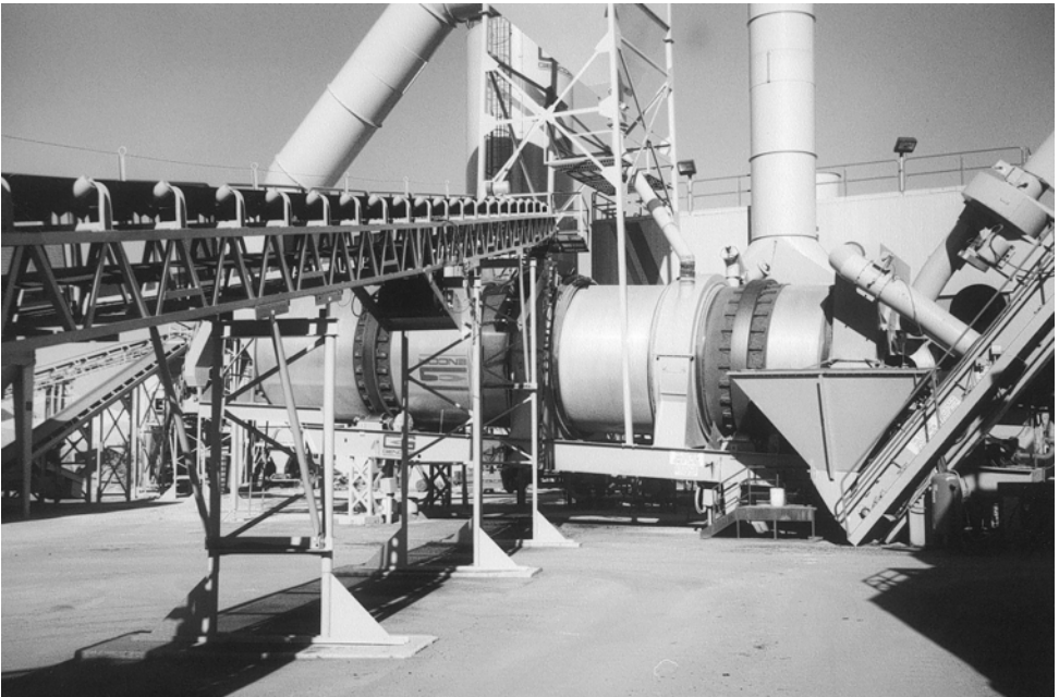
Plate 6.13 RAP conveyor on a drum mix plant.
