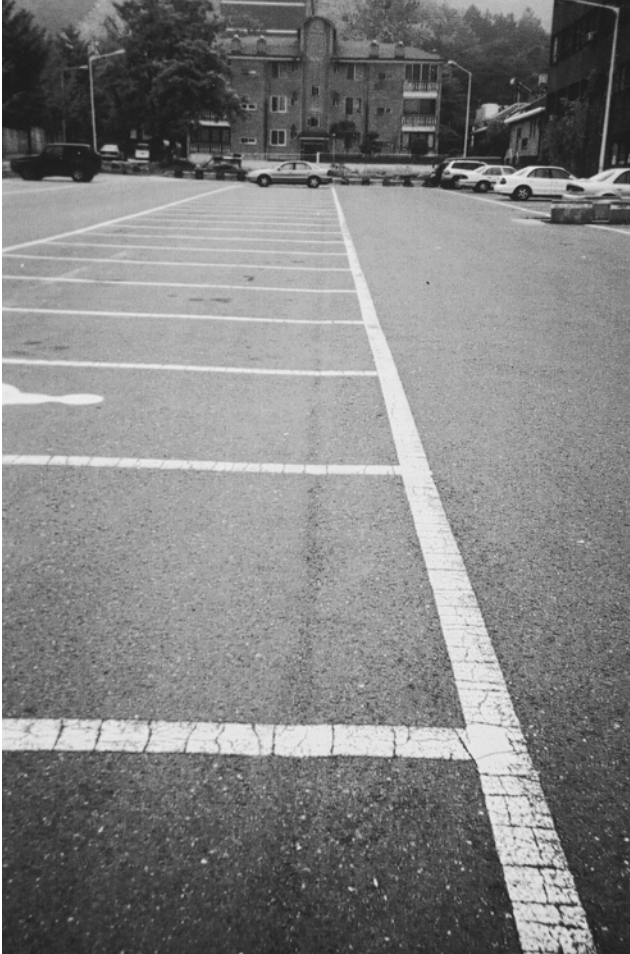
Plate 8.16 Longitudinal crack at construction joint.
