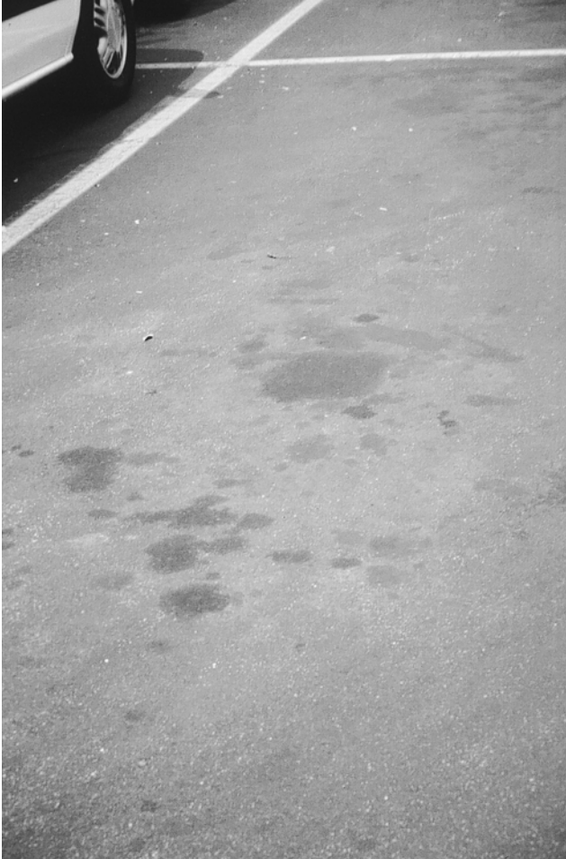
Plate 8.2 Oil spillage in a parking stall.
