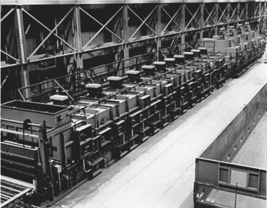
FIGURE 10.21 Photograph of a roller hearth furnace. (Courtesy of Electric Furnace, Salem, OH.)
