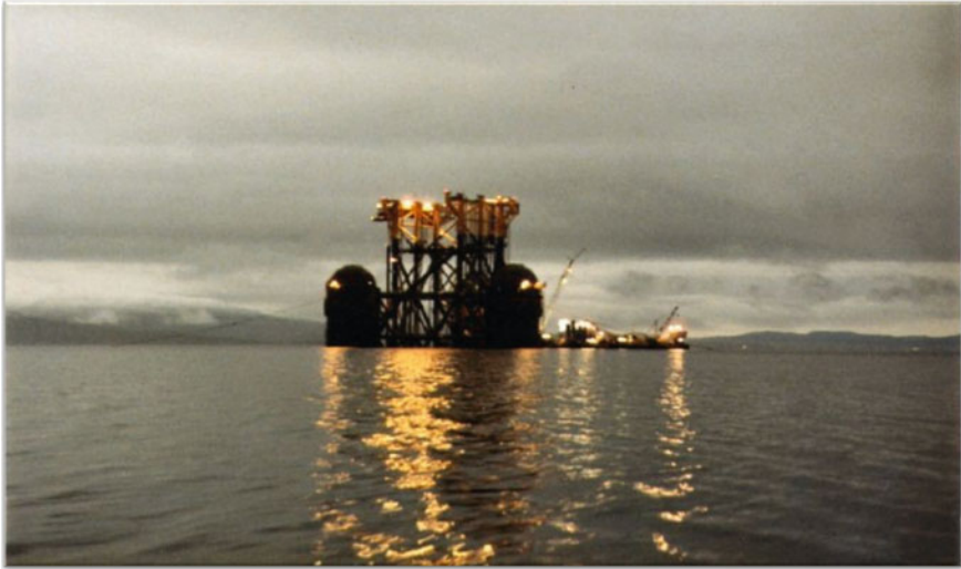
Fig. 3.7 Maureen substructure waiting for the mating with the topsides. The Mating operation was the first HIDECK floatover technology application (courtesy of Oil Rig Photos)
