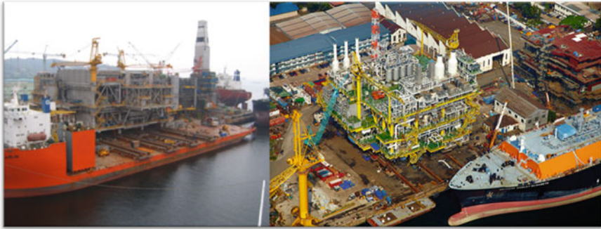
Fig. 5.2 The skid beam and grillage design for the two projects should be basically the same. On the left is the topsides of GN platform to be loaded out to the installation vessel; on the right is the installation vessel for the integration of the MDPP platform of CPOC (courtesy of Technip and Sembcorp respectively)
