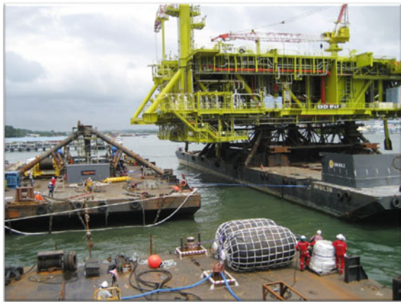
Fig. 6.19 The operation of transfer the Kikeh topsides from the transportation barge to the floatover barge was carried out at harbor of Labuan, East Malaysia. The floatover barges were hooked up with the topsides one by one with the first one approached from the starboard of the transportation barge (courtesy of Murphy Oil Corporation and Technip) [18]
