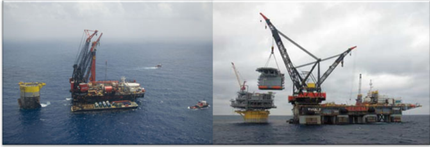
Fig. 2.50 In early 2009 HMC installed the integrated topsides of the Perdido with a 9773 ton single lift by their SSCV Thialf, a record for the US part of the GOM. The living quarter was then put on the topsides. It took two weeks to complete the installation (courtesy of HMC and Shell)
