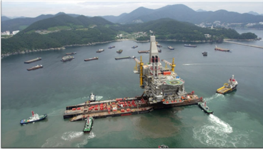
Fig. 10.1 The heaviest single vessel floatover in open water—the integration of GBS platform Arkutun-Dagi completed in 2014. The total installation weight was 42,000 tons (courtesy of HMC) [1–3]
