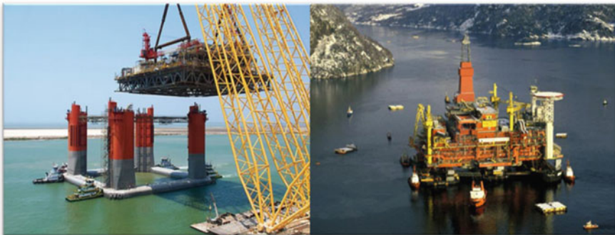
Fig. 2.25 The integration site should be carefully selected for successful mating operation. On the left is the topsides installation by heavy lifting for WHO DAT topsides. On the right , it shows the topsides of Statfjord B being carried out on barges near the mating site ready for floatover (courtesy of KOS and StatOil)
