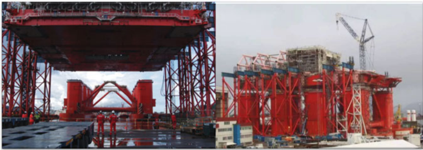
Fig. 2.43 Aker H6-e semisubmersible drilling rig was integrated at the drydock of Aker Stord yard (courtesy of Aker Solutions)
