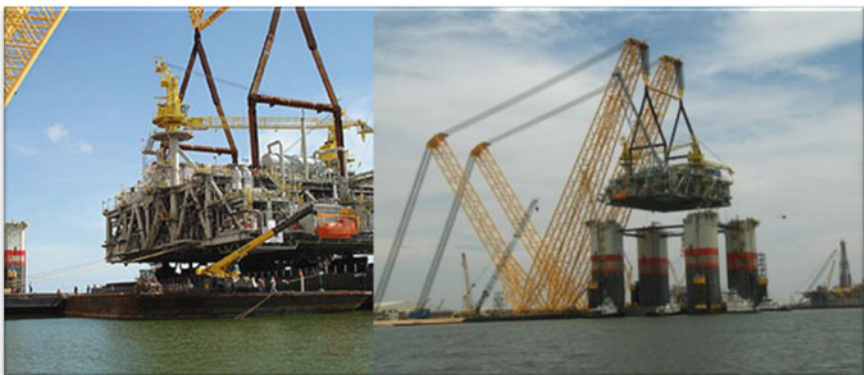
Fig. 2.31 The platform integration of Chevron Blind Faith DDS. The topsides is an integrated topsides. HLD (Heavy Lifting Device) lifted the integrated topsides from the transportation barge ( left ) and put on the hull ( right ) (courtesy of Rigzone and KOS)
