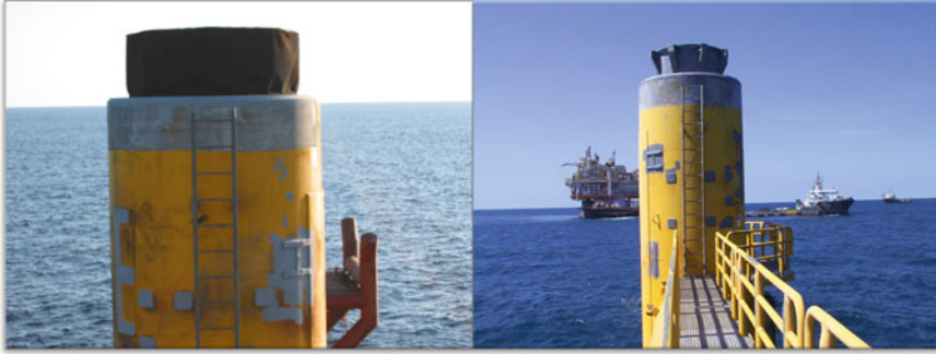
Fig. 9.11 On the left , it shows the LMU is under the weather protection cover before the field preparation; on the right , the LMU is ready for the floatover operation (Photo credit to Bayu Undan project)
