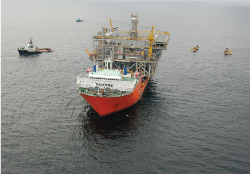
Fig. 3.5 The floatover installation of Nigeria East Area 1 B GX platform with the topsides weighing 12,381 t. There are more than 27 open water floatover worldwide so far (courtesy of boskalis)
