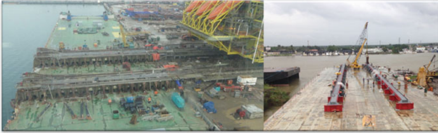
Fig. 9.5 Skid beam layout on the vessel: the left picture shows the skid beams for transverse loadout of KBB platform topsides and the right picture shows the skid beams for the loadout operation to pull the topsides onboard the vessel from the stern ( Left photo courtesy of COSCO and credit of the right photo to a barge modification project)
