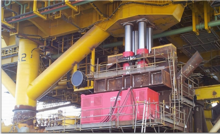
Fig. 9.16 The DSU with hydraulic jacks is ready for the retract after the topsides weight is 100% transferred to the jacket (Courtesy of Dorman Long Technology) [4, 5]
