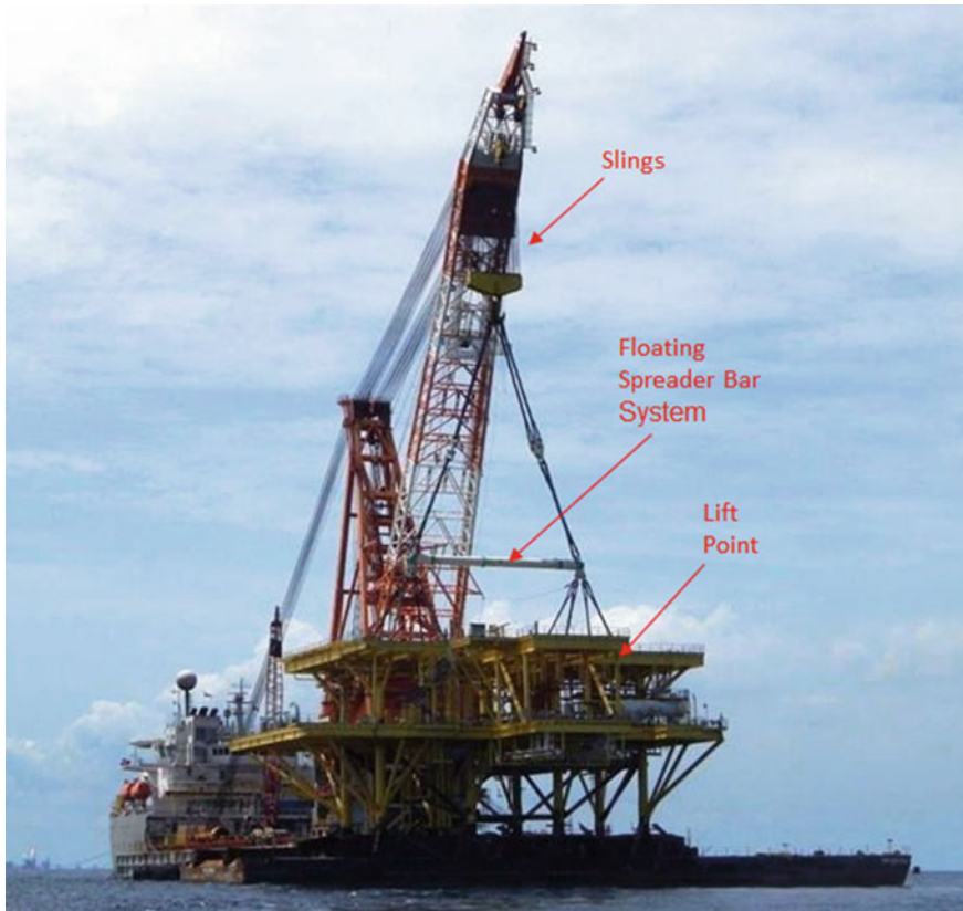
Fig. 1.26 The mechanism of the topsides lifting by crane (Courtesy of Shanghai Salvage Bureau)
