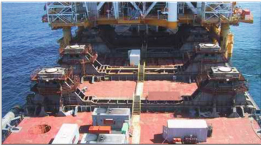
Fig. 9.17 Floatover vessel is moving off the jacket slot after the completion of the topsides installation (Courtesy of Dorman Long Technology) [4, 5]
