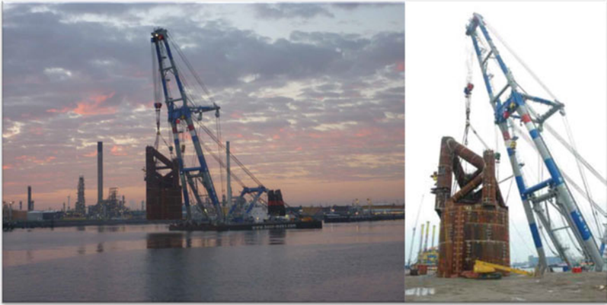
Fig. 2.13 Suction bucket with leg stiffening frame on the top is lifted by Matador 3 and put in position to be connected to the platform leg (courtesy of ©Heerema Fabrication Group)
