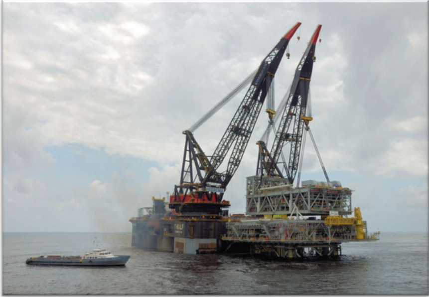
Fig. 2.51 The Center Module was lifted and put on the MSF of the Chevron TOL (Tombua Landana) compliant tower platform in offshore Angola (courtesy of Chevron)
