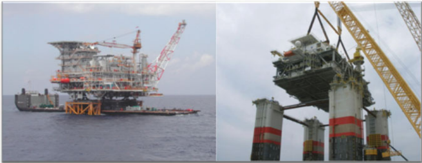
Fig. 1.21 The platforms were integrated with different approaches—Floatover versus Heavy Lifting (Credit to the BP Lan Tay and the Chevron Blind Faith projects)
