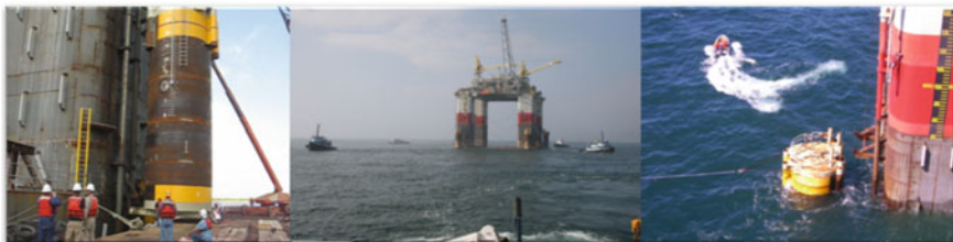
Fig. 2.27 Temporary sponsons for handling inshore towing stability issue. The left shows the sponsons are installed at quay; the middle shows the platform under tow with sponsons attached. The right shows one of the sponsons was just separated from the hull column (credit to the Blind Faith T&I project)
