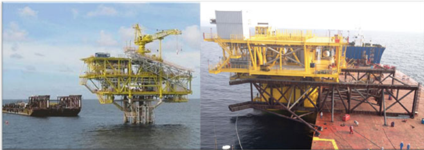
Fig. 10.11 On the left is the floatover equipment by the ICON Engineering Pty Ltd for installation topsides up to 1200 tonnes. The photo on the right is the installation of the 1500 ton topsides of the CX-15 platform for EPZ Energy of Peru (courtesy of ICON Engineering and HortonGMC respectively)
