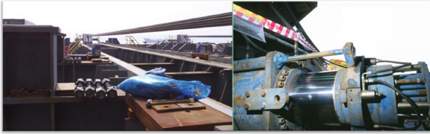
Fig. 9.8 Strand jack pulling system: on the left is shown the strand cables connected to the fixed anchorage installed on the upper deck of the transportation/floatover vessel; on the right is the strand jack hooked up with the DSS supporting the topsides (Photo credit to Bayu Undan project)
