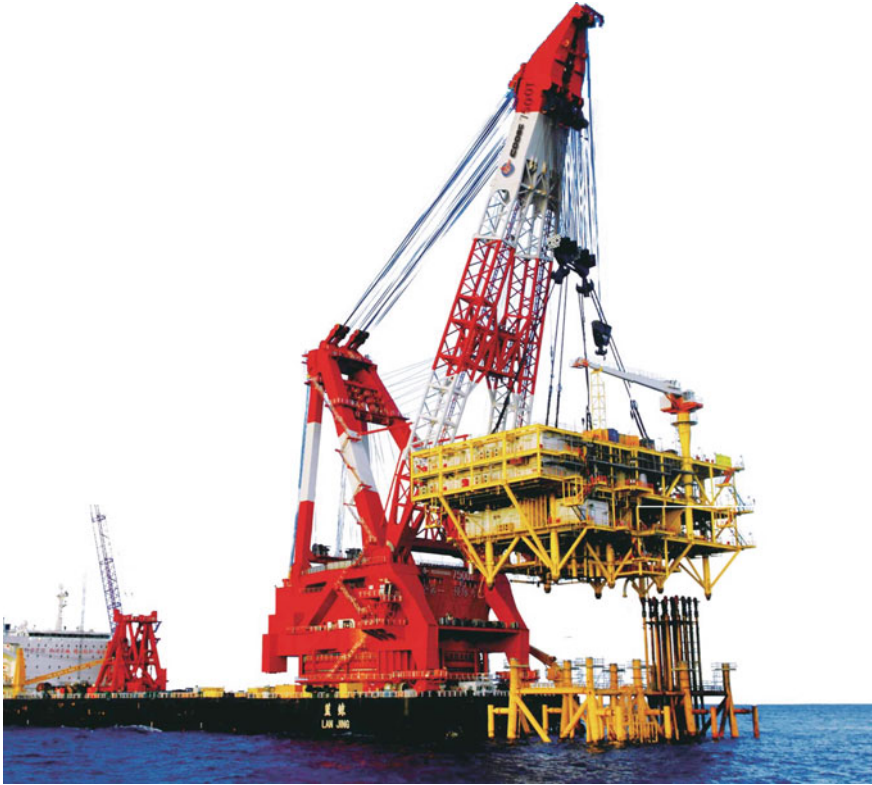
Fig. 3.1 Smaller and light topsides can be lifted by Derrick Vessels (courtesy of COOEC)
