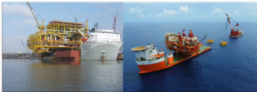
Fig. 10.8 DP floatover: on the left is the first DP floatover installation of Bunga Raya topsides in Malaysia, 2003 using COSCOL MV Tai An Kou; on the right is the DP floatover of Huizhou 25-8 DPP topsides in South China Sea, 2014 (courtesy of Talisman and CNOOC respectively)
