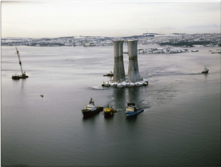
Fig. 2.26 Condeep Statfjord B was towed to the integration site at Yrkje Fjord in Vindafjord. (Courtesy of Statoil)
