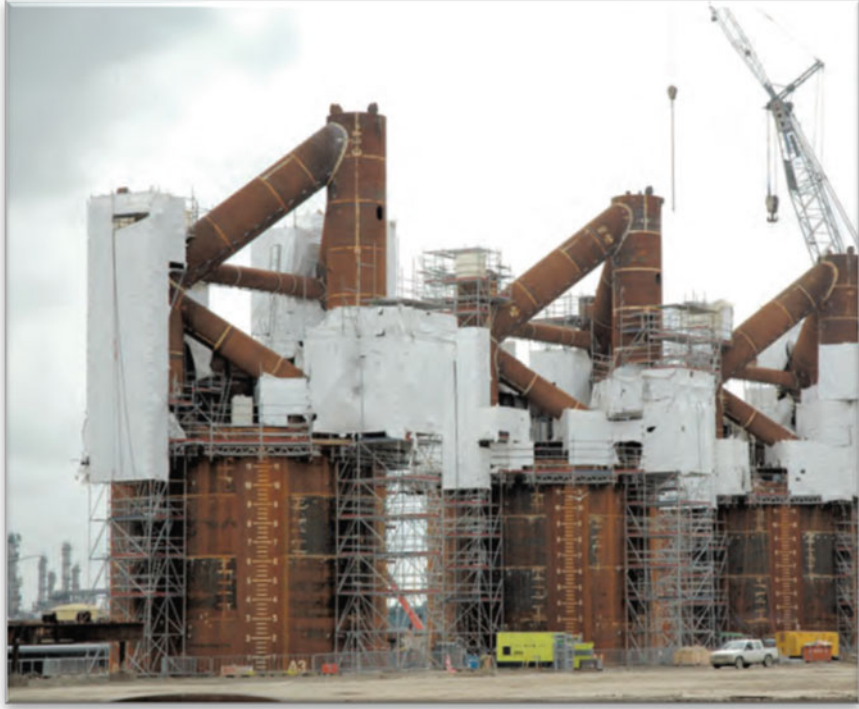
Fig. 2.11 For each suction pile, the leg-stiffening frame was already welded to it and the assembly was ready to be connected to the platform leg (courtesy of Han Heilig, publisher of Offshore Holland, the Netherlands)
