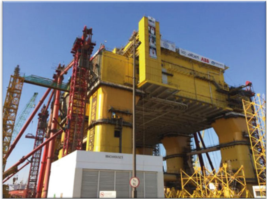
Fig. 2.45 The topsides of the Dolwin Beta was lowered on the columns of the semisubmersible look-like GBS hull, the ALE's gantry system can be seen clearly (courtesy of Drydocks World and ALE)
