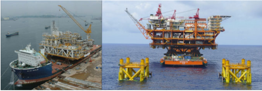
Fig. 3.9 There are more DTVs and large capacity barges available globally and the MOB/DEMOB is much easier and faster comparing to HLCVs. On the left is the loadout of the Bayu Udan topsides on Dockwise's DTV Blue Marlin. On the right shows the successful floatover installation of HZ25-8 topsides (courtesy of bayu udan project and CNOOC) [13]
