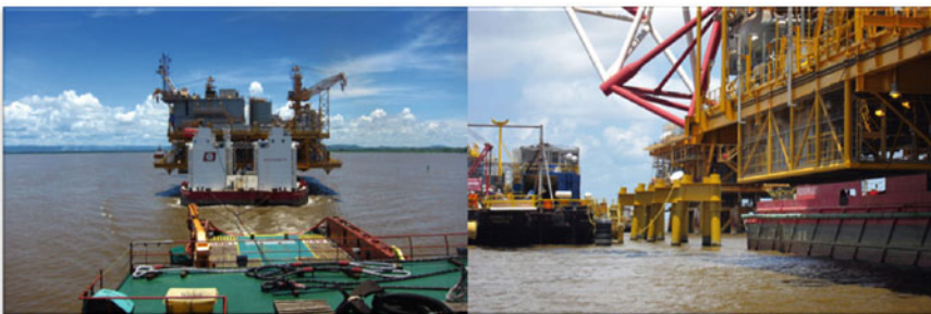
Fig. 10.2 COROCORO CPT Topsides was installed using floatover method in 2011. The water depth was only 5.6 m (courtesy of ConocoPhillips)
