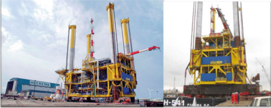
Fig. 2.12 Loadout of F3-FA topsides. On the left , it shows the topsides was being loaded out to the transportation barge at the fabrication yard. On the right the topsides was first moved on board Heerema barge H-541 and then positioned on Boa Barge 35 (courtesy of ©Heerema Fabrication Group)
