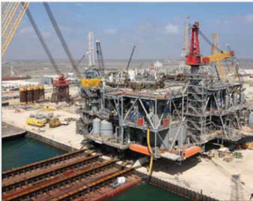
Fig. 1.13 Lightweight single lift topsides for Shell Perdido Spar was loaded out from Kiewit Ingleside yard (Courtesy of Shell) [16]
