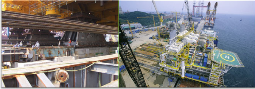
Fig. 9.10 Topsides skidding operation: on the left , the topsides is at the edge of the quay and ready to be moved onto the link-beam; on the right , the topsides weight transfer is continuing (Photo credit to Bayu Undan project)
