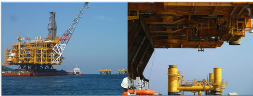
Fig. 2.54 SHWE platform integration in Bay of Bengal, Myanmar. The weight of the topsides is 26,000 Mt carried by the COOEC barge HYSY 229 (courtesy of Dockwise)
