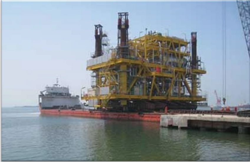
Fig. 10.5 Application of the “strand jack lifting technique” to the 6200-ton topsides in West Bohai Bay of China. The four (4) columns at each corner of the topsides are equipped with strand jacks for lifting the topsides (courtesy of ALE)
