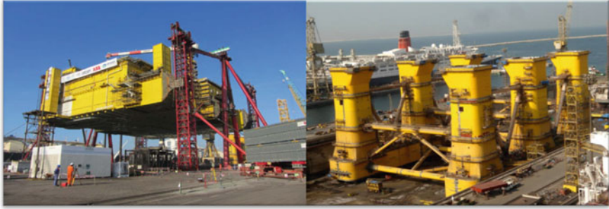
Fig. 2.44 Both of the topsides and the hull were built in the drydock of the Drydocks World yard at Dubai, the topsides was fabricated in the drydock (courtesy of Drydocks World and ALE)
