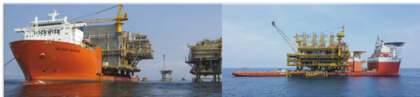
Fig. 5.7 Pre-mating stage. On the left is the GN platform integration using UNIDECK method in West Africa with 18,000 tonne topsides and on the right is the MDPP platform integration using HIDECK method in Southeastern Asia with 19,000 tonne topsides. Both projects used Dockwise's HLV Black Marlin (courtesy of Dockwise)
