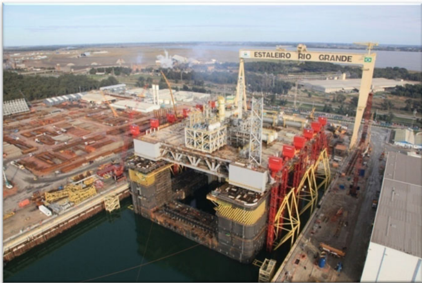
Fig. 2.42 The topsides and the hull were aligned and ready for mating (courtesy of Petrobras)
