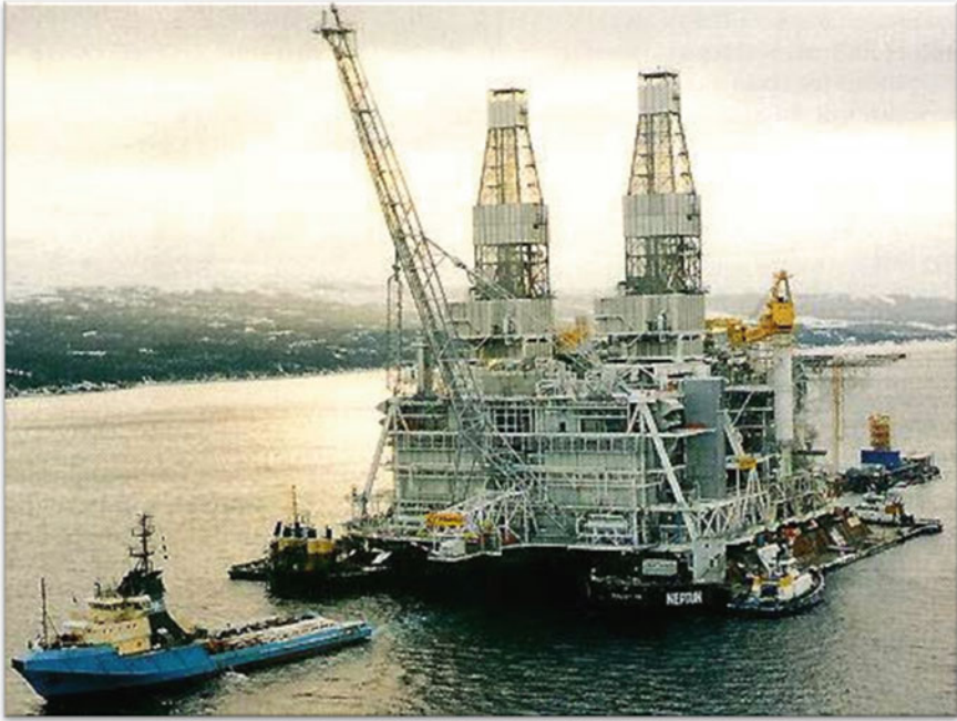
Fig. 6.4 Hibernia topsides was towed to the inshore mating site (courtesy of HMDC) [6]
