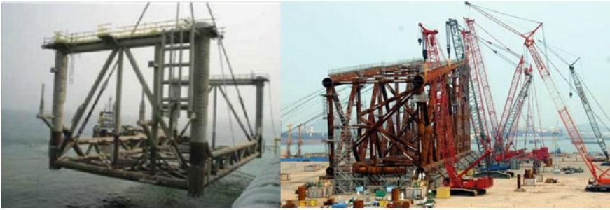
Fig. 1.15 Jacket design with consideration of topsides installation (Courtesy of Chevron and COOEC respectively)
