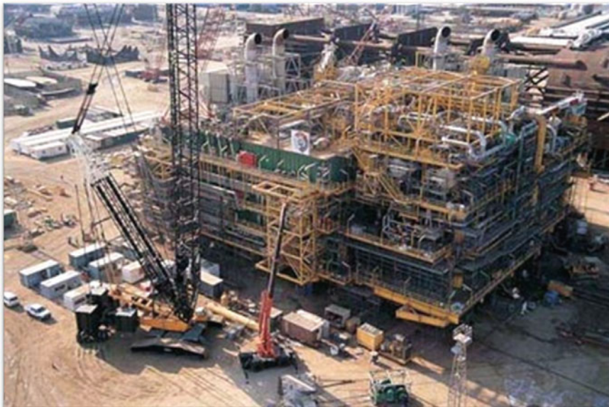
Fig. 1.11 The Integrated topsides AMP1 for Amenam/Kpono project (Courtesy of Elf Petroleum Nigeria)
