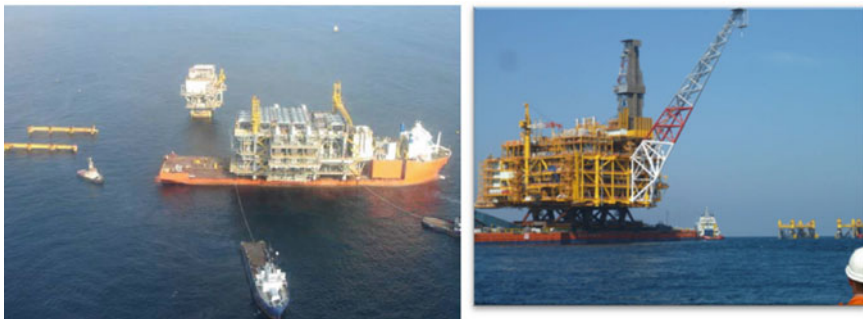
Fig. 5.5 Except the capability of topsides elevation adjustment by the jacking system for UNIDECK method, no big difference in project execution for the two methods. On the left is the GN platform integration using UNIDECK method and on the right is the SHWE platform integration using HIDECK method (courtesy of Dockwise)
