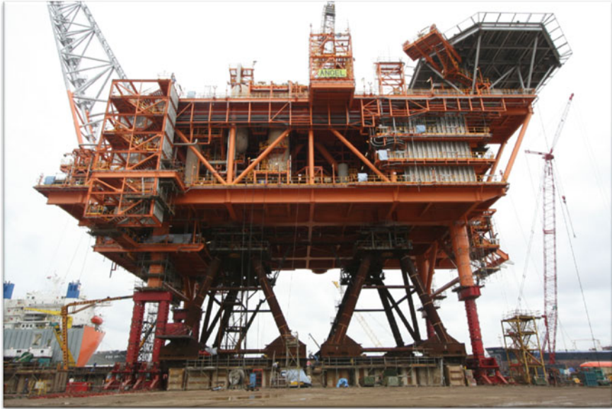
Fig. 8.11 The DSF designed for Angel platform topsides transportation is much higher comparing to other projects (courtesy to Woodside Angel project)
