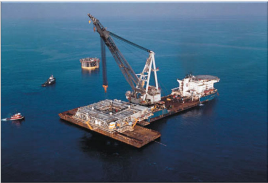
Fig. 2.52 The McDermott DB-50 was preparing to lift up the lower deck of the Genesis spar topsides (courtesy of McDermott)
