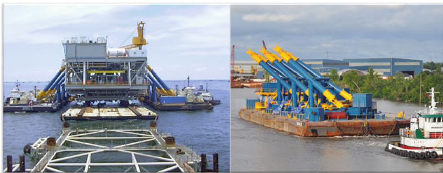
Fig. 6.13 The Versatruss heavy-lift system. On the left shows the floatover topsides installation using the Versatruss heavy-lift system in Lake Maracaibo, Venezuela, in 1999. Three platform integration operations were successfully carried out. On the right , it recorded the long journey of the system to Saudi-Arabia for two topsides installation in 2010 (courtesy of Versabar Inc.)
