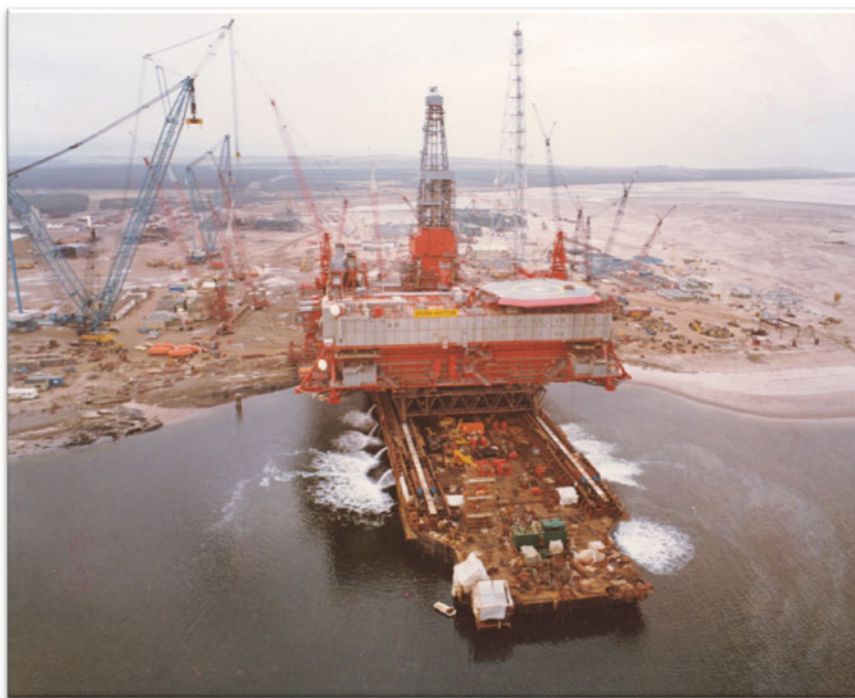
Fig. 4.7 The topsides of the Hutton TLP was a HIDECK design and fully commissioned before the inshore mating with the Hull (Courtesy of ConocoPhillips)
