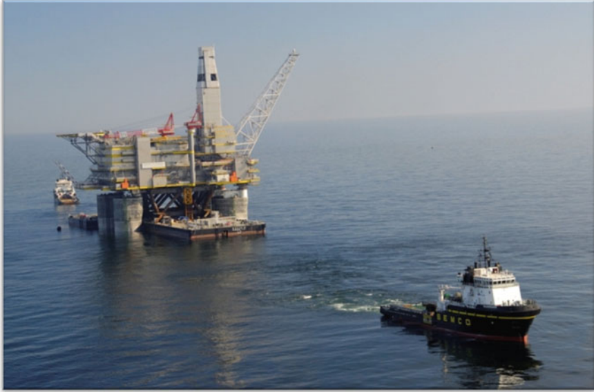
Fig. 2.56 Sakhalin II project PA-B platform floatover topsides installation (courtesy of Posh Terasea Offshore Pte Ltd.)
