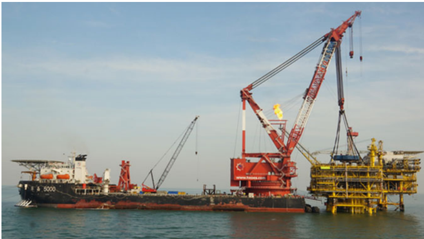
Fig. 2.47 The topsides of a fixed platform was installed by a crane barge (courtesy of CNOOC)
