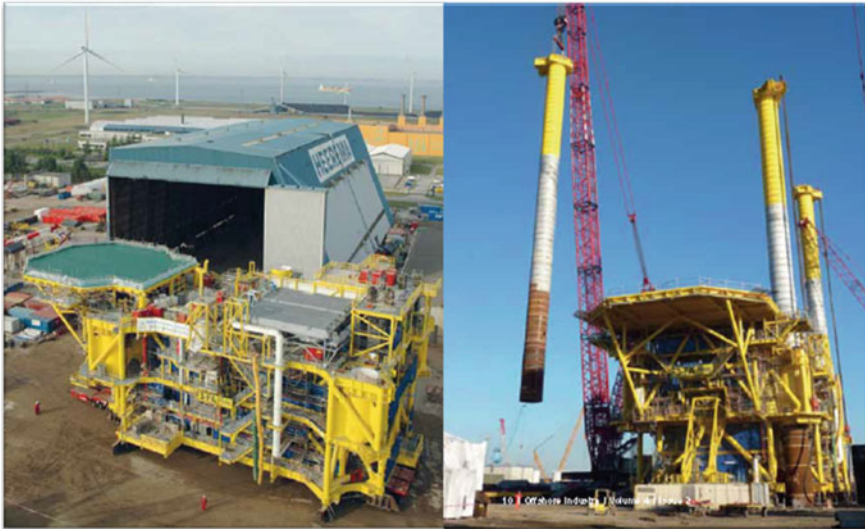
Fig. 2.10 On the left , the fabrication of the 4000 t topsides is completed and moved out from the fabrication hall and ready for the leg installation; on the right shown the installation of the legs by the yard crawler cranes (courtesy of Centrica Energy)
