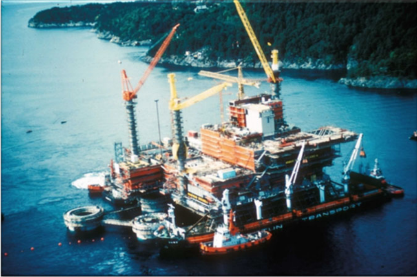
Fig. 2.32 Mating operation of Statfjord A. The topsides was not an integrated topsides, a few modules were installed on the MSF which is carried by two tankers and then floated over the shafts of the base which was only a few meters above the water surface (courtesy of Norwegian Petroleum Museum)
