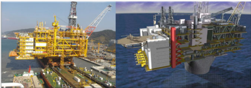
Fig. 3.8 Very heavy topsides is no longer rare now. On the left is the topsides of SHWE A-1 platform weighing about 30,000 tonnes and on the right is the under construction Hebron GBS of which the platform integration will use catamaran floatover with the mating load up to 40,000 tonnes (courtesy of shell and warleyparsons) [11, 12]
