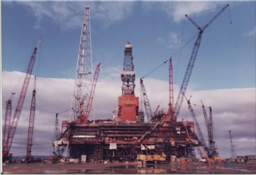
Fig. 2.37 The topsides of Conoco (UK) Ltd's Hutton TLP was under construction at Ardersier Yard (courtesy of Oilrig-Photos)
