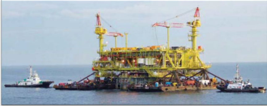
Fig. 2.58 Murphy's Kikeh truss spar platform integration offshore Malaysia in November, 2006 was the first open water catamaran floatover operation and was successful (courtesy of Technip)
