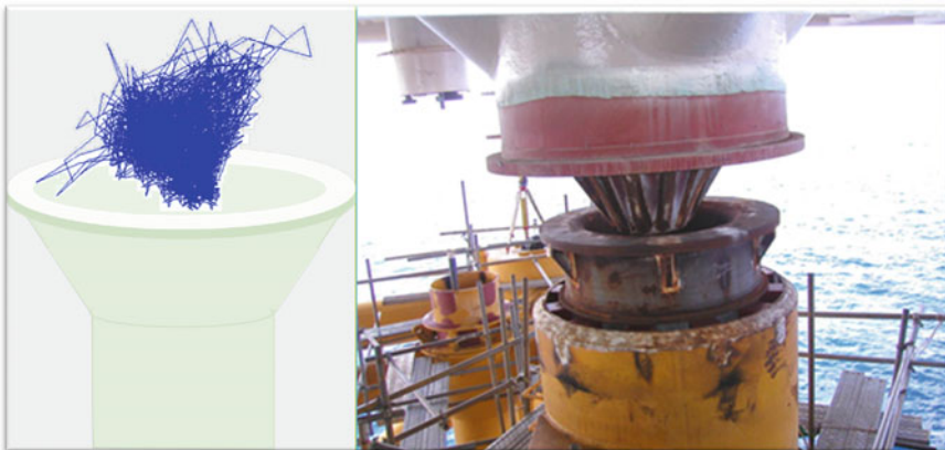
Fig. 9.14 In the pre-mating stage, the stabbing cone is engaged with the LMU. On the left , from the stabbing cone movement traces it can be seen that the motion does not go exceeding the opening of the receiving cup horizontally (Photo credit to Lan Tay project)
