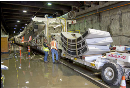
Figure 9. RTV transporting segments (Image credit: sfmta.com)
