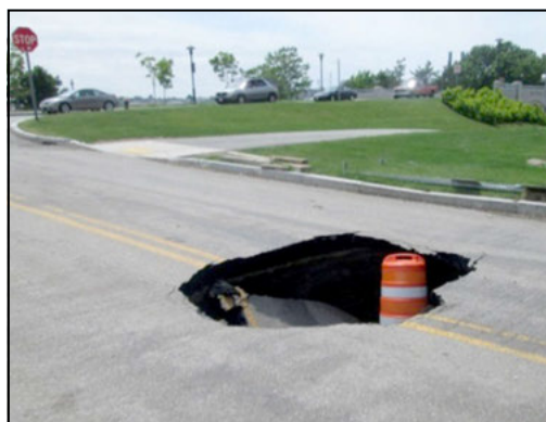
Figure 4. Sinkhole due to microtunneling
