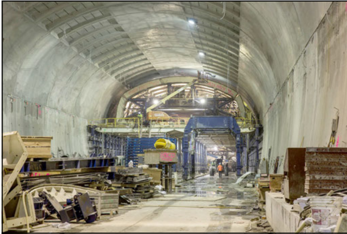
Figure 6. Photograph of public station cavern final lining with exposed coffers and formwork system in view
