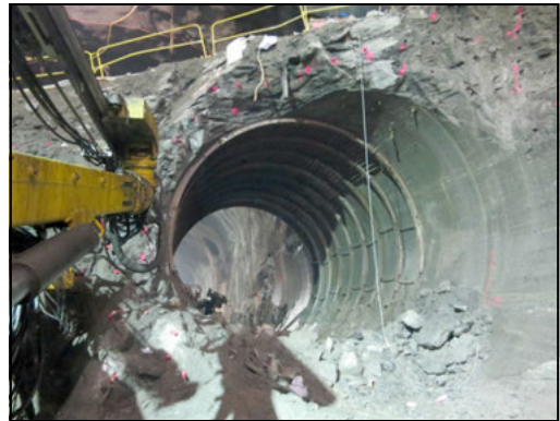
Figure 13. Final stage in the station cavern—for the removal of the rock surrounding the TBM tunnel
