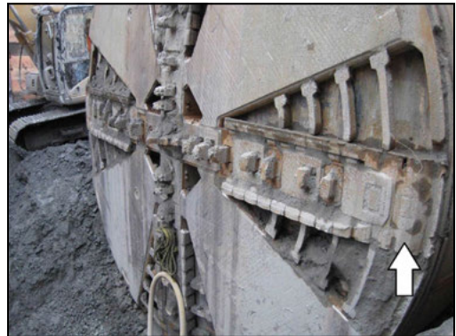
Figure 13. Severe wear of cutterhead and cutting tools
