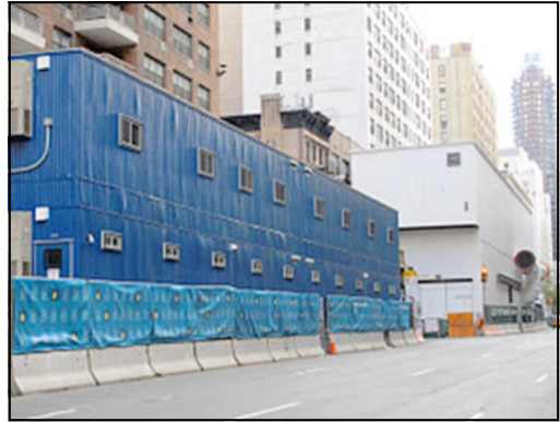
Figure 18. Construction site on 2nd Avenue showing features of field office (blue) and Muck House (white)
