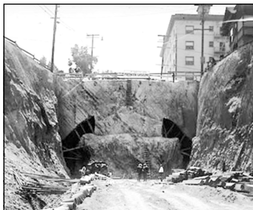
Photo 2. Stacked drift construction for the Second Street Tunnel, ca. 1921 (Courtesy of University of California, Los Angeles, on behalf of the UCLA Libraries Special Collections)
