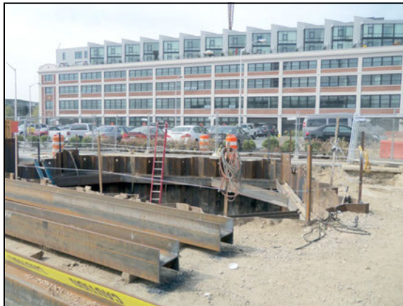
Figure 3. The CSO-013 diversion chamber excavation, with Forest City's Foundry Lofts apartments in the background. Forest City worked directly with their residents and their contractor to minimize construction impacts.
