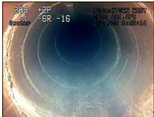
Figure 2. Circumferential cracks with precipitates (white “rings”)
