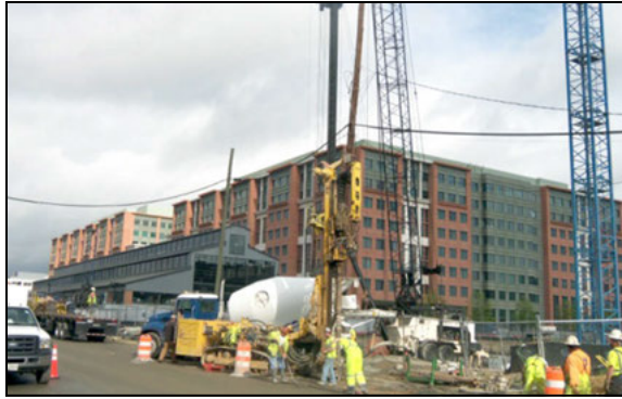
Figure 8. Tunnel crews working adjacent to crews working on Forest City’s Twelve12 mixed-use development. The transit mixer belonged to the building contractor, but the drill rig is part of the tunnel project. Both projects reported to the Forest City Washington.
