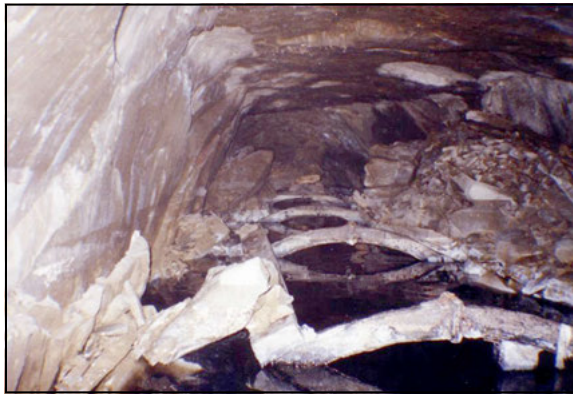
Figure 6. Deteriorating condition of the existing wastewater tunnels
