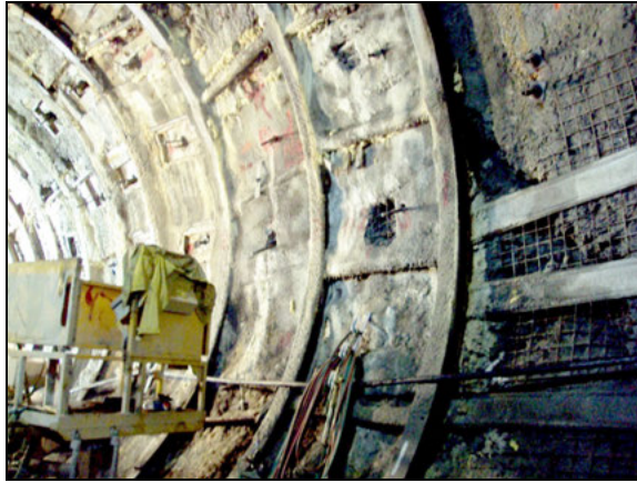
Figure 7. MAI bolts installed through cellular grout into minimum 10-ft (3-m) sound bedrock
