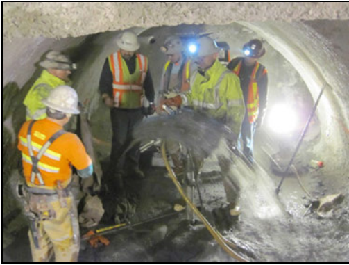
Figure 3. Groundwater encountered at Cross Passage 17 channelized through probe hole
