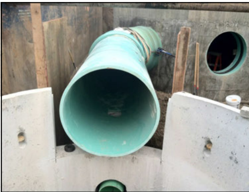
Figure 11. Typical 914 mm (36 in) sewer
