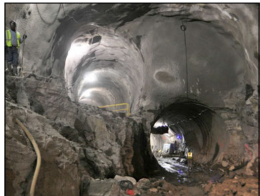
Figure 14. Completion of the G3 and G4 tunnels at the Stub Cavern—with a final separation of only 6 feet
