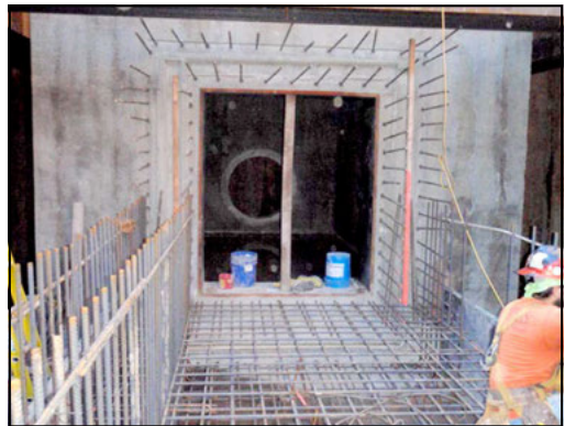
Figure 13. Typical screen and gate structure with approach channel
