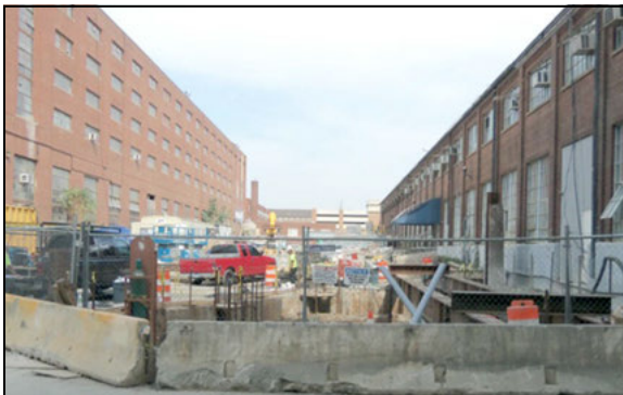
Figure 7. The CSO-014 excavation and receipt shaft were immediately adjacent to two historic Washington Navy Yard buildings that Forest City is planning to renovate as part of the overall area redevelopment program
