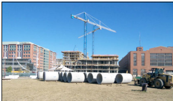
Figure 9. During one phase on the project, Forest City allowed storage of sewer pipe on a vacant lot for about 3 weeks. Small accommodations such as this helped the project succeed.
