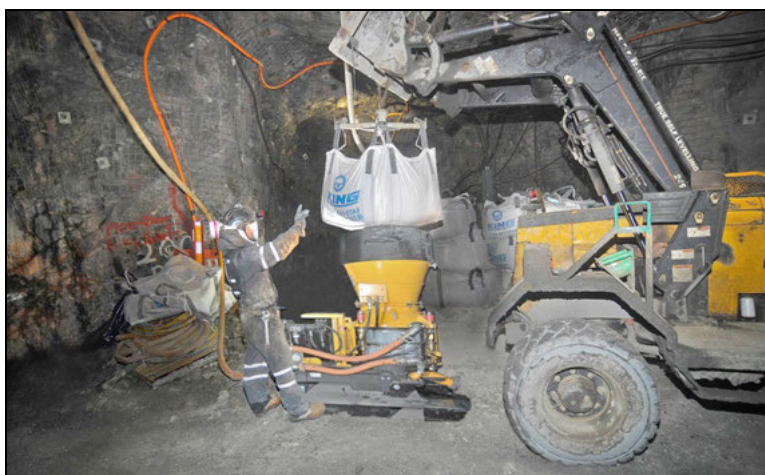
Figure 1. Aliva 252 dry-mix shotcrete machine being loaded with a dry, pre-mixed, pre-packaged shotcrete mix in a bulk bag
