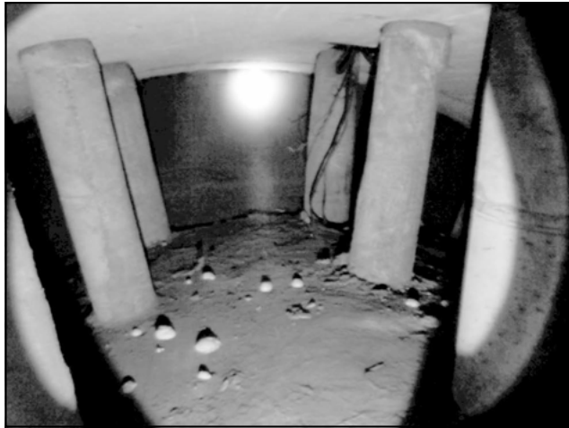
Figure 4. Embedded hangers in existing void space between main tunnel and ventilation arch wall
