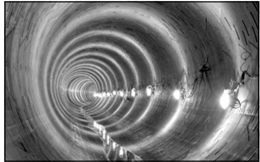
Figure 1. Lewis and Clark, TBMs began excavation from the Nicolai Shaft. Lewis completed the journey north, under the river to the Confluent Shaft and then to the Swan Island Pump Station Shaft. Clark completed its journey and broke through on July 29th, 2005 at the Clay Street Shaft. This work is complete and the tunnel became 100% operational in December 2006.
