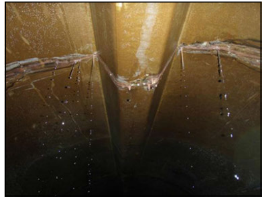
Figure 4. Pink precipitates at cracks with water inflows
