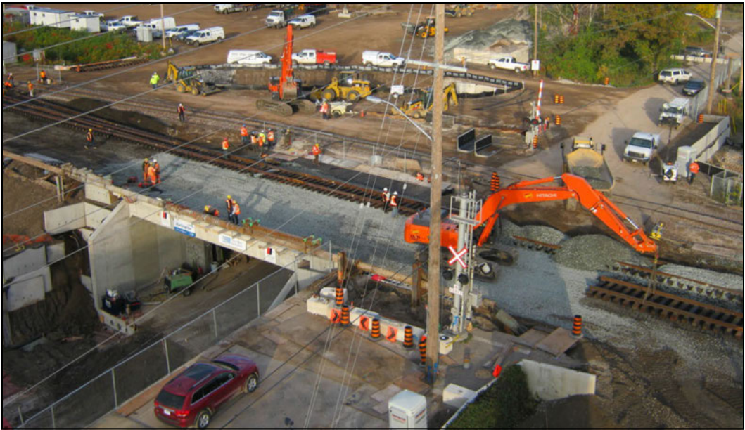
Figure 5. Underpass structure in its final position with the rail tracks being replaced Monday afternoon
