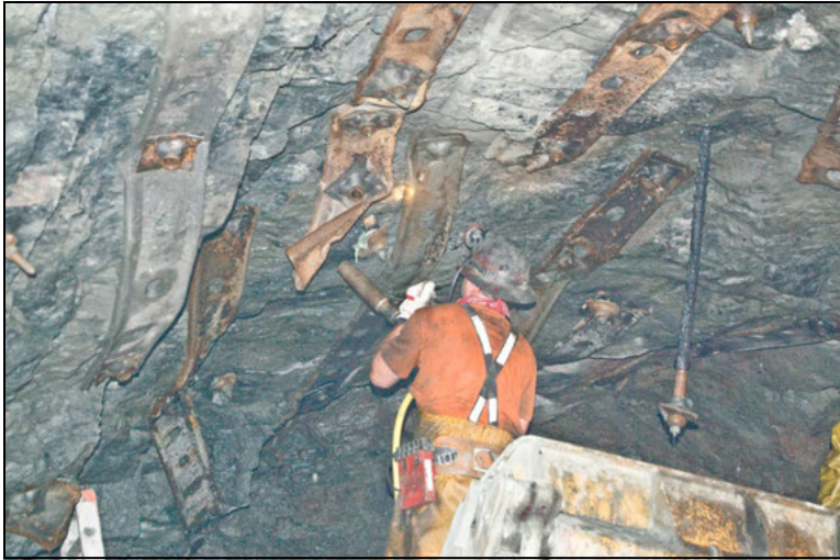
Figure 1. Installing “permanent” anchor bolts next to “temporary” friction anchors and mine straps already in advanced stages of corrosion
