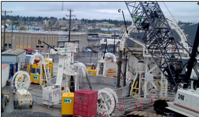
Figure 5. Vertical shaft machine system viewed from the surface including: (a) a shaft liner hoist; (b) a vertical shaft machine hoist; and (c) the utility line guidance tower
