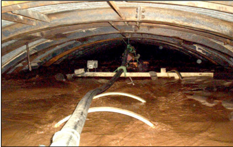
Figure 9. Parbati TBM buried in silt
