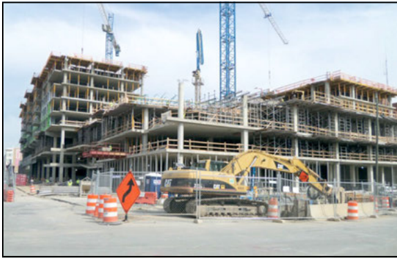
Figure 2. The CSO-013 manhole shaft (cat excavator) sits directly in front of the Twelve12 building construction project. Casual observers would think they are the same project, but they are unrelated.
