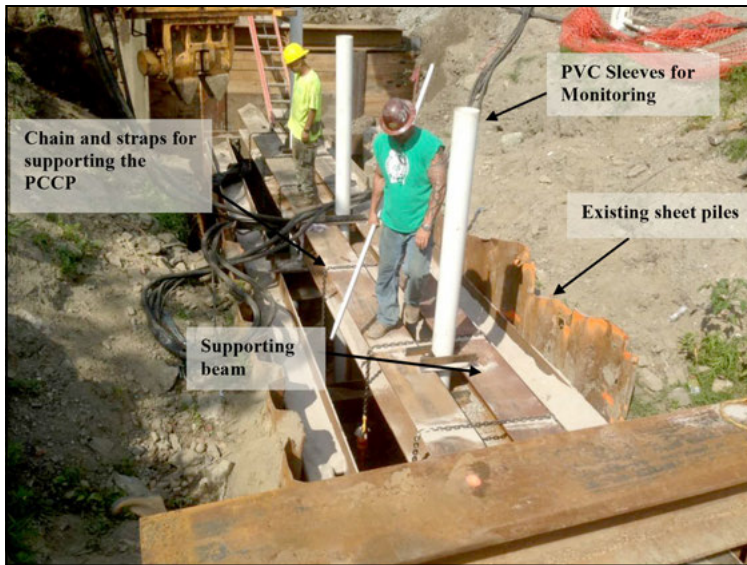
Figure 8. Support system and utility monitoring for 42-in PCCP
