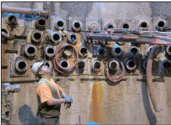
Figure 8. Compensation grout array at Ellis Street shaft
