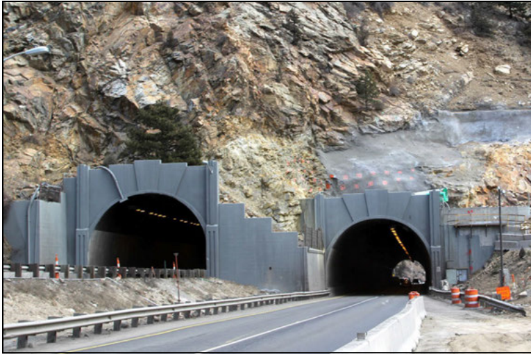
Figure 1. West side portals before the start of the widening with the eastbound tunnel portal on the right
