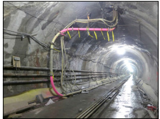
Figure 15. Concrete slicklines in G3 running tunnel connected to the 66th Street pumping station
