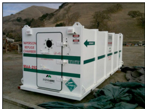
Figure 9. Refuge chamber used in tunnel heading
