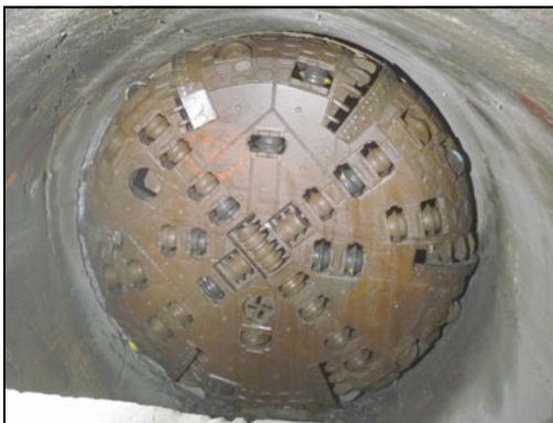
Figure 4. Removal of the double-shield SELI TBM (no tolerance for protruding rock support)
