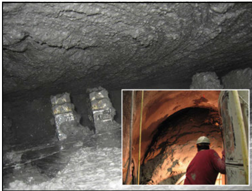
Figure 7. Tunnel face in soil with stand-up time (Insert shows fast raveling ground)
