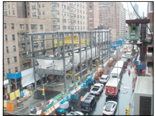
Figure 11. Construction of one of two Muck Houses erected at the site—for efficient materials handling
