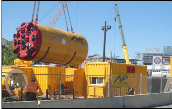
Figure 5. Northeast Remesco’s microtunnel boring machine “Go Yard” being readied for launch in the shadow of the Washington National’s baseball stadium
