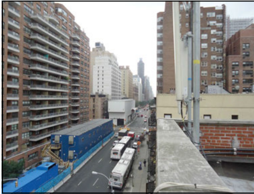
Figure 17. Construction site on 2nd Avenue showing the field office (blue) and Muck House (white)
