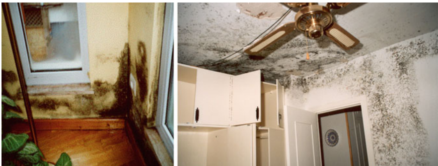
Fig. 5.19 Condensation dampness from façades (left) and roofs (right)
