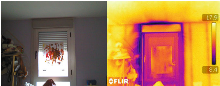
Fig. 5.5 Origin of infiltrations through the blind box cassette. Detection by means of blower door and thermography
