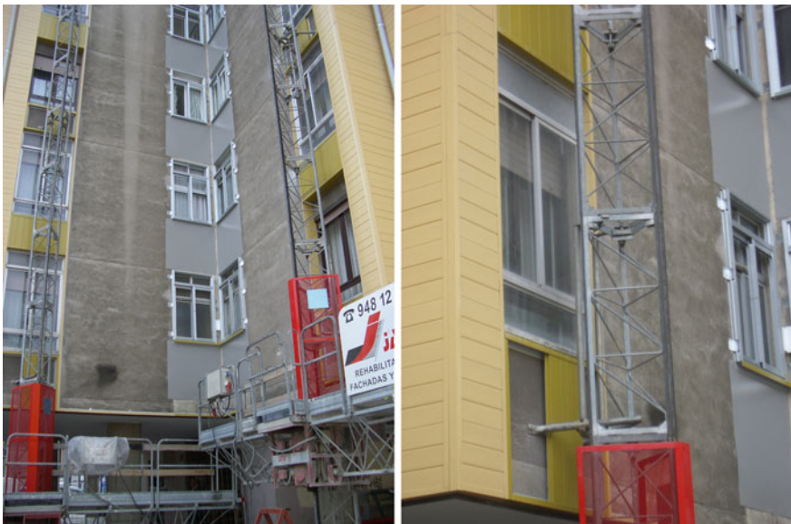
Fig. 5.6 Intervention in windows: placement of a new window outside the existing one
