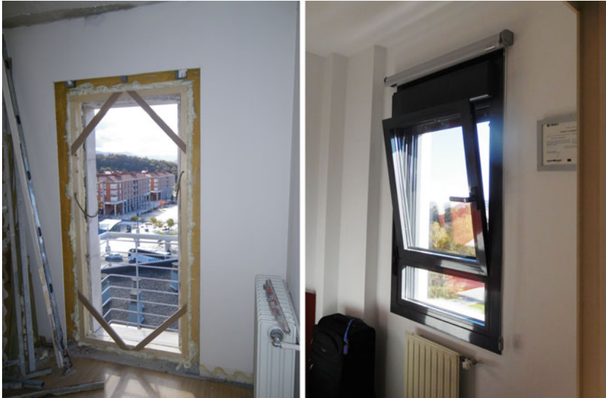
Fig. 5.23 Replacement of window in process (left) and replacement of windows with blind box cassettes by monoblock system (right)
