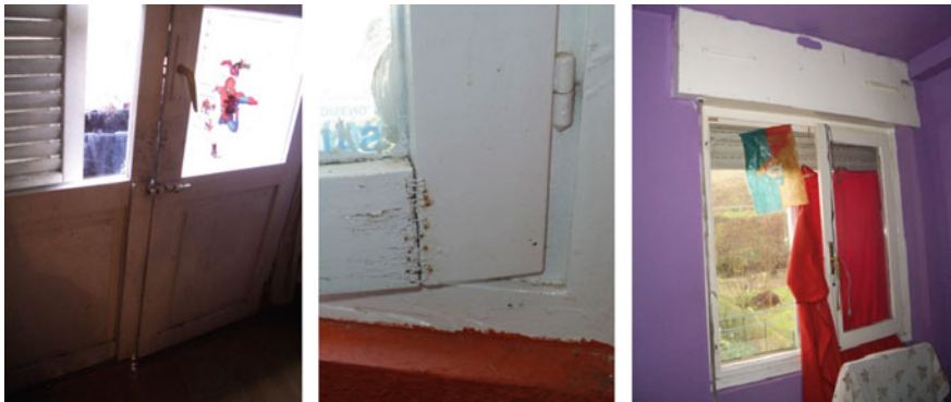
Fig. 5.24 Condition of windows found on inspection of dwellings
