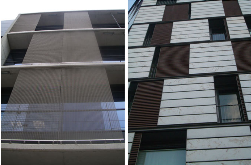
Fig. 8.39 Examples of shading in contemporary buildings: fixed (e.g. in Logroño, Spain) or movable (e.g. in Barcelona, Spain)
