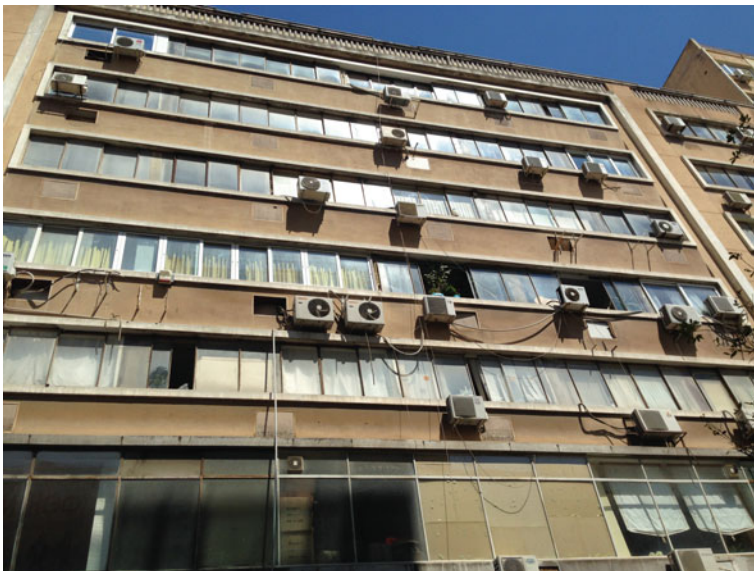
Fig. 8.38 Extensive use of air conditioning devices without control in the façades. Athens (Greece)
