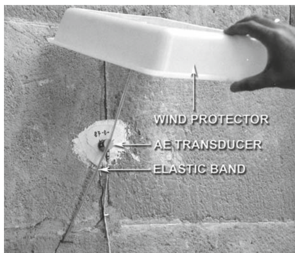
Fig. 18.8 Transducer protection system during AE monitoring
