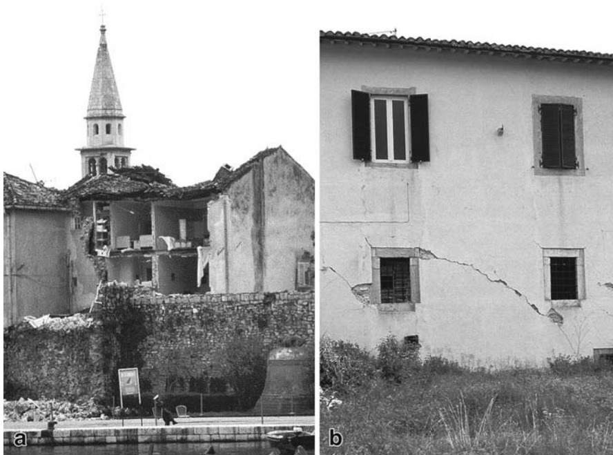
Fig. 17.2 Typical earthquake damage to stone-masonry heritage buildings: a out-of-plane collapse of perimeter walls and b typical shear cracks in the walls
