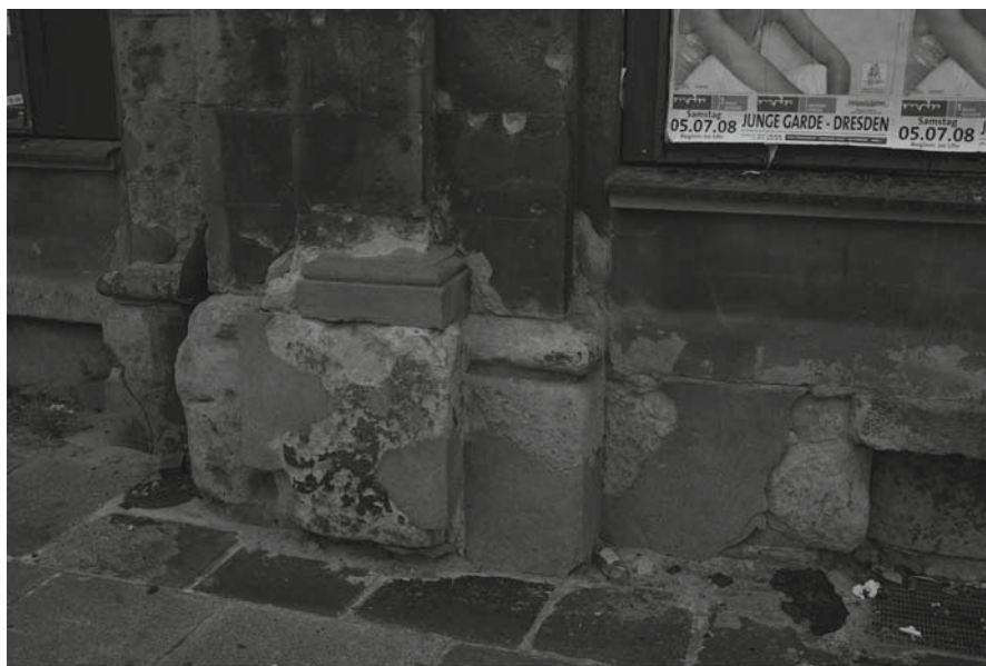
Fig. 8.9 Cotta sandstone in the base of a building from the late 19th century (Jahnstraße). The decayed sandstone was partially covered with repair mortars
