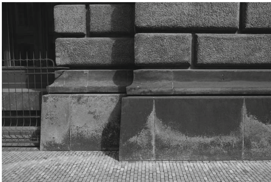
Fig. 8.5 Granodiorite from Lusatia, used in the bases of the building of the Academy of Fine Arts in Dresden, is in a stable condition after 115 years of exposure to splash water
