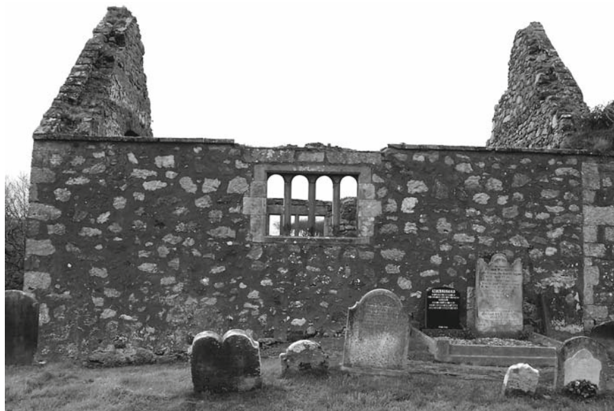
Fig. 7.2 ‘Rigid’ mortar at Bonamargy Friary, causing ‘box-work’ appearance
