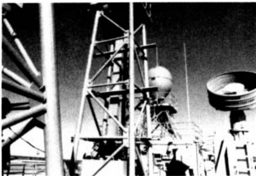
Figure 4-20(b) Enclosing Mast Cable Runs Within EMI Trunk
