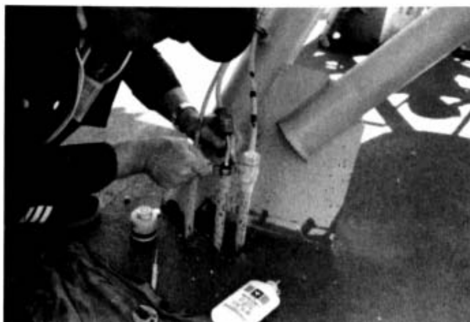
Figure 4-17 Careful Grounding and Sealing of Cable at Deck Entry Points
