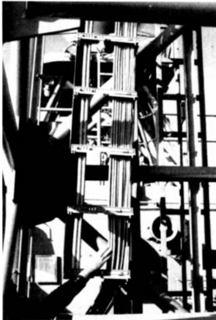
Figure 4-20(a) Enclosing Mast Cable Runs Within EMI Trunk
