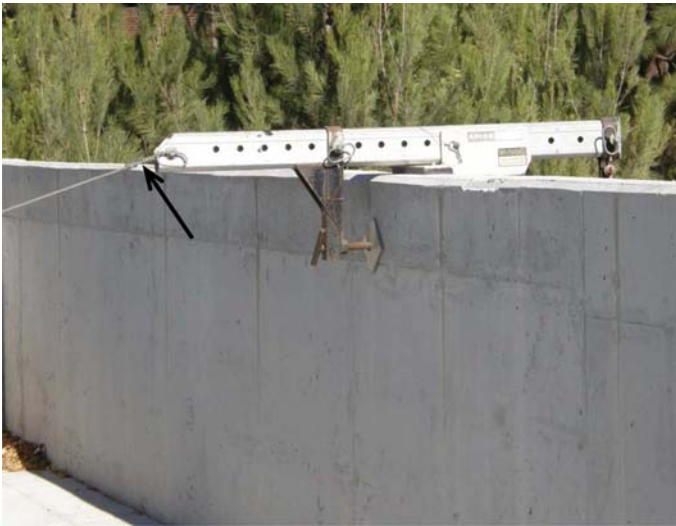
Figure 3. Parapet clamp with outrigger arm. Note the tieback cable at the interior end of the outrigger arm (black arrow). Similar to Figure 2, the clamp is temporary equipment provided by the contractor and outside the scope of this guideline.
