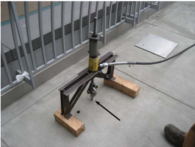
Figure 11. Tension load testing a threaded insert in a concrete slab (black arrow). In this case, the anchorage is intended to resist a vertical upward force, so that is the direction of the applied test load. A reaction frame is used to move the reactions against the slab away from the insert so that the concrete is tested against breakout. Source: Figure 9 in Larson et al. (2014); copyright ASCE.
