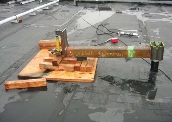
Figure 14. Example of appropriately oriented testing of lifeline anchorages perpendicular to the roof edge to the right. The maximum applied moment is equal to that generated by the 5,000-pound horizontal force at the top of the anchorage. The test is slightly more rigorous than the actual factored load would generate because the load applies a net uplift force rather than a net horizontal shear force; this deviation is generally small, conservative, and typically unavoidable.
