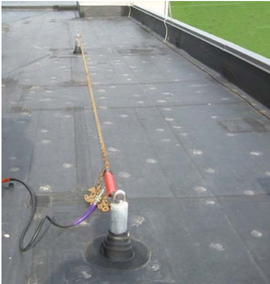
Figure 13. Example of anchorages being tested parallel to the roof edge. If these anchorages are to be used when accessing the building façade to the right or left sides of the photo, the test load is not being applied in a direction capable of verifying their suitability for that use. Source: Figure 15 in Larson et al. (2014); copyright ASCE.
