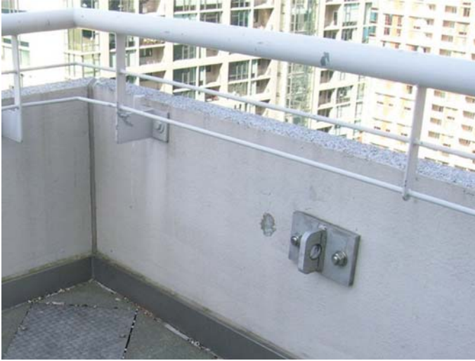
Figure 6. Lifeline or fall arrest anchorage installed on a parapet/guardrail wall.
