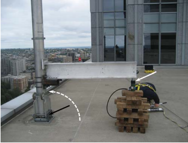
Figure 8. Load testing a davit base (black arrow). The horizontal member is a test beam and not part of the dedicated system. The solid white arrow indicates the hydraulic ram. The cribbing under the ram allows the ram to be positioned at the correct elevation and also spreads out the load applied to the roof. The curved white dashed arrow indicates the overturning moment created by the hydraulic ram. Pressure (load) is measured with a calibrated dial gauge or load cell specific to the equipment being used. The test load is applied in the anticipated direction of the in-service load.
