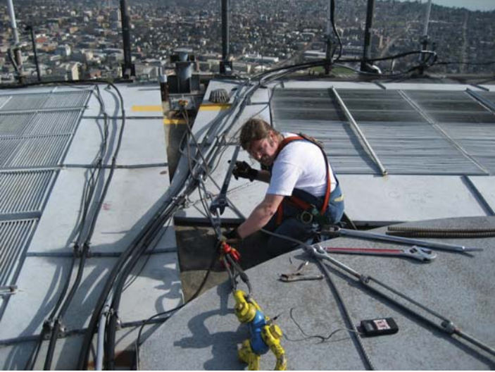
Figure 10. Load testing of a lifeline/tieback anchorage. By reacting against another anchorage on the opposite side of the roof, two anchorages can be tested at the same time. In this case, the lifeline anchorages are intended to be used with a lifeline from a davit across the width of the building; hence the test load is being applied in the correct direction.
