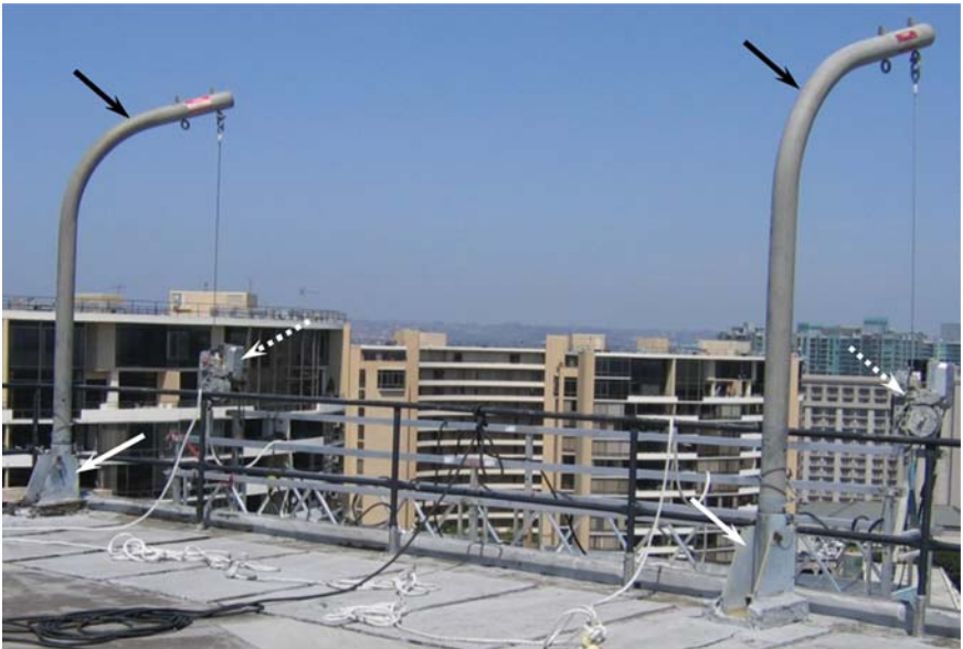
Figure 1. Davit bases (white arrows) and davit arms (black arrows) being used to suspend a platform over the side of a building. Note that the connections of the davit bases to the primary building structure are often hidden from view and cannot be visually inspected without removal of roofing materials. Dotted white arrows indicate the hoists (motors).
