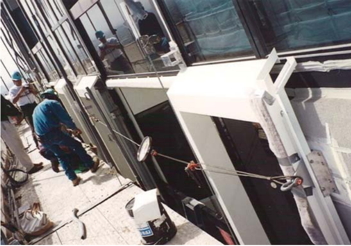
Figure 12. Load testing intermediate stabilization anchors on the face of a building. The test pulled from one anchor to the adjacent anchor to generate the required load parallel to the building face, effectively testing two anchors at one time.
