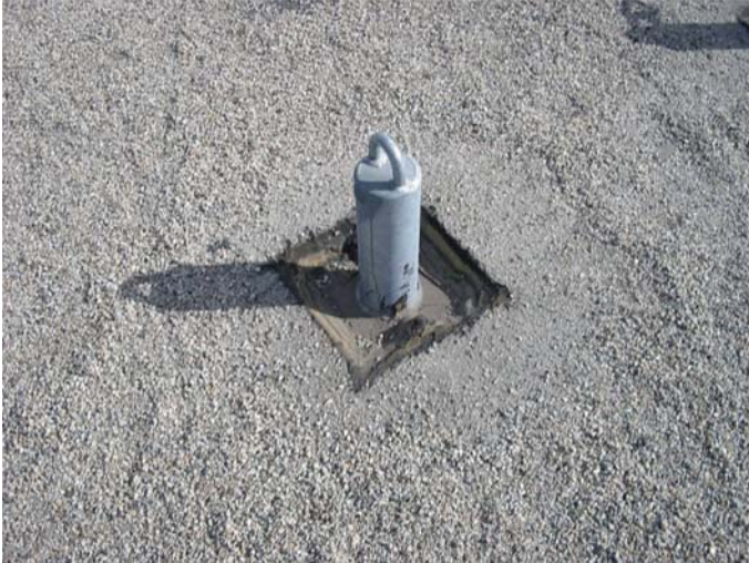
Figure 5. Pedestal-type roof anchorage, which may be used as a lifeline anchorage and/or equipment tieback anchorage. The connections of this anchorage to the primary structure are buried in the roofing material, making inspection of the connections impossible without removal of roofing materials.
