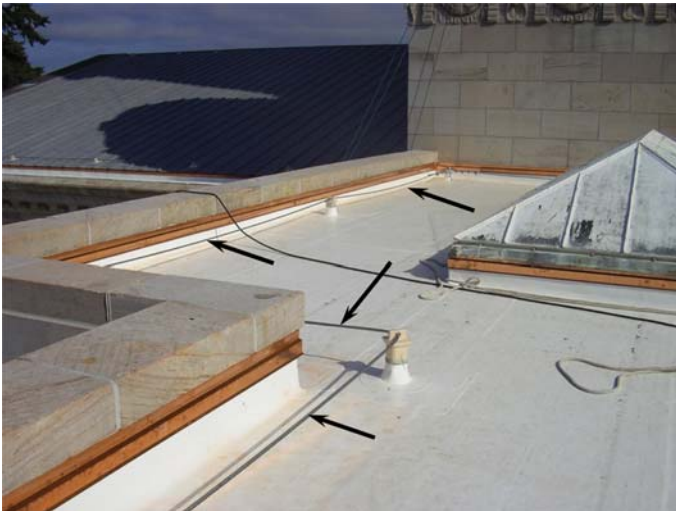
Figure 7. Horizontal cables (black arrows) can be used as points of anchorage for vertical lifelines. Loading a wire rope like the one shown with a 5,000 pound vertical lifeline load can create forces in corner and end anchorages many times larger than 5,000 pounds.
