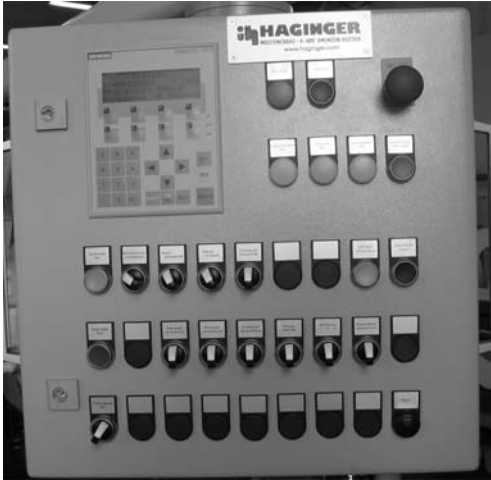
Fig. 6 Panel of a PLC based control system
