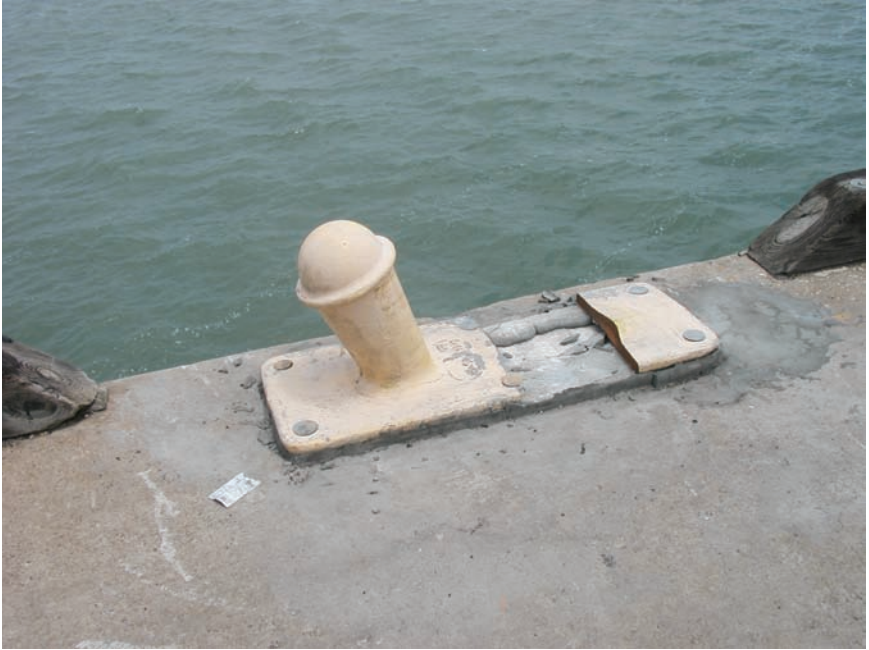
Fig. 6-1. Failed double bitt that occurred with thunderstorm wind gust Note: Poor grout bedding likely contributed to overstressing of the bollard base, which also likely had a defect
