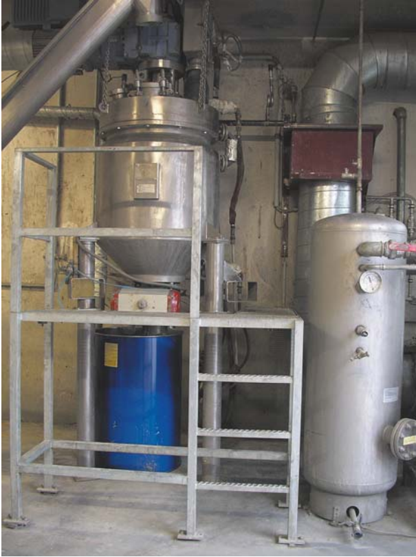
Fig. 3. Solvent treatment with a distillation plant
