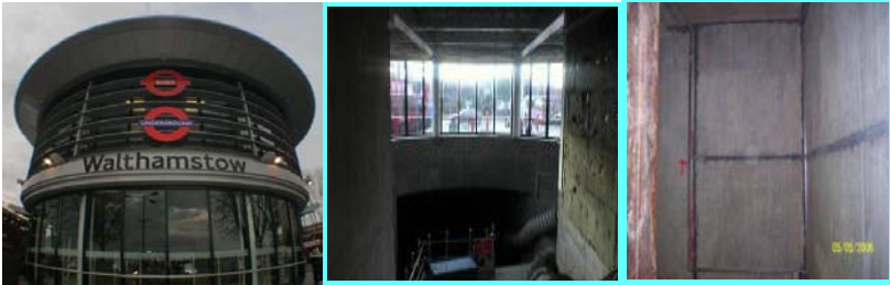
Figure 7: MPS® Installation Pictures for Walthamstow Underground Station
