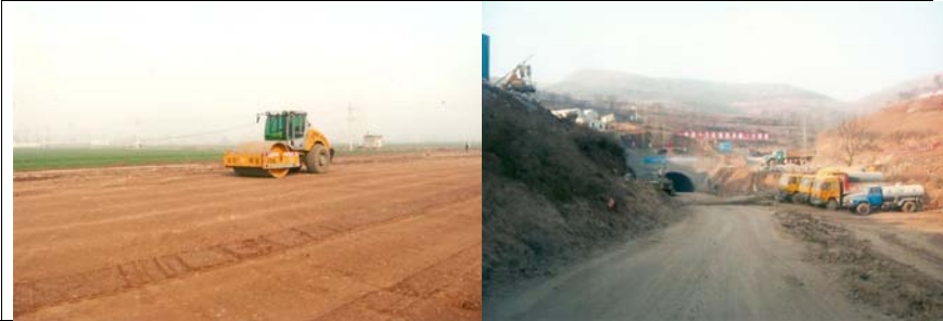
FIGURE 3. Subgrade preparation and compaction in December 2006 (left). South entrance of one of the twin tunnels in December 2006 (right).
