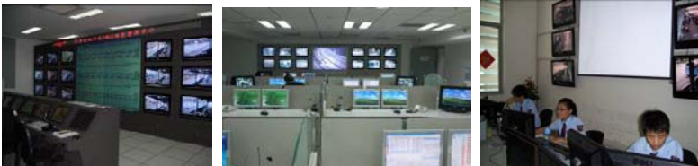
Figure 10. Control center of Changzhou, Beijing and Xiamen BRT
