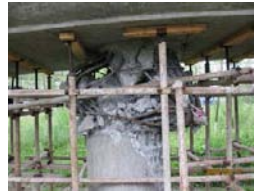
Fig. 2. Plastic failure at top zone of columns
