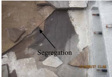
Fig. 6. Segregation of mortar
