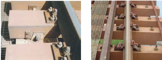
Figure 3.1-1 K type fastener and elastic rod fastener on the resin sleeper of the Shinkansen Japan
