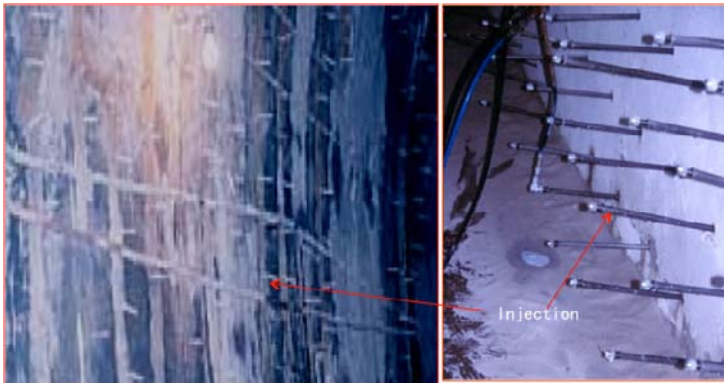
Figure 2. Concrete Wall Calcification from Water Ingress & Polyurethane Injection
