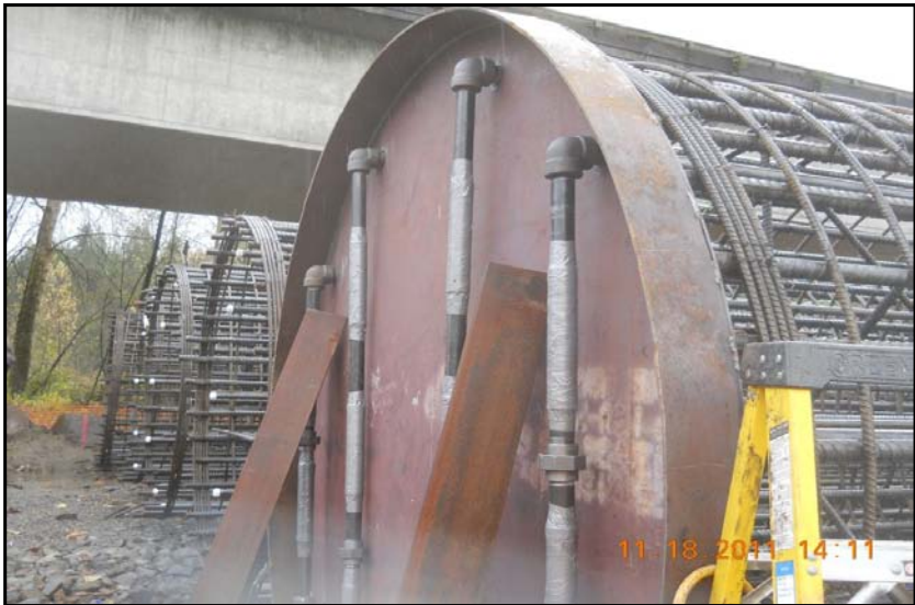
Figure 4 Tip Grout (Base Grout) for Pier 7 & 8 (the existing bridge is on the left)
