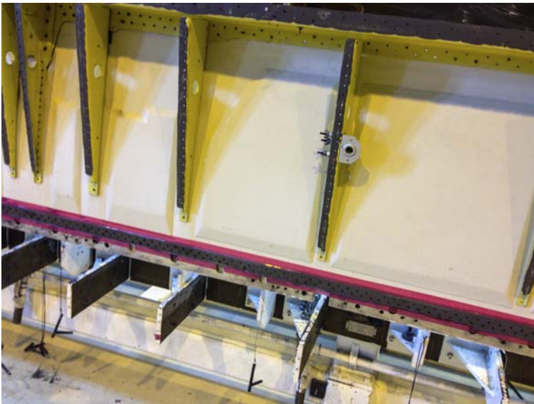
Figure 3.3 Tolerance accumulation brings gaps, and shimming is necessary to fill them during assembly.
