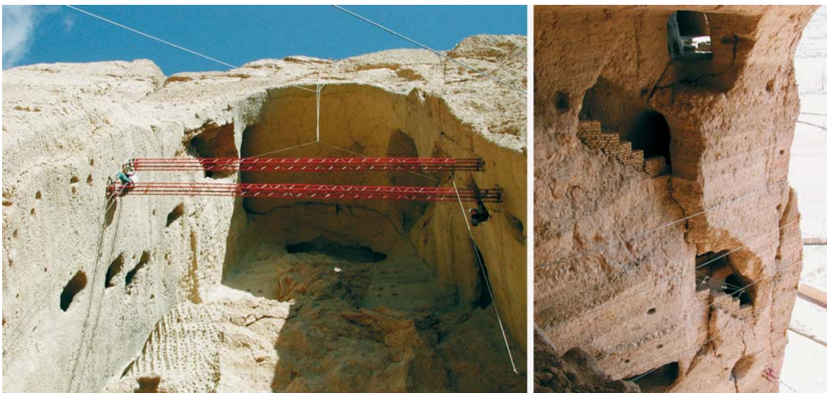
Fig. 8.4. The beam (left) and steel rope (right) for the temporary support of upper Eastern part of small Buddha
