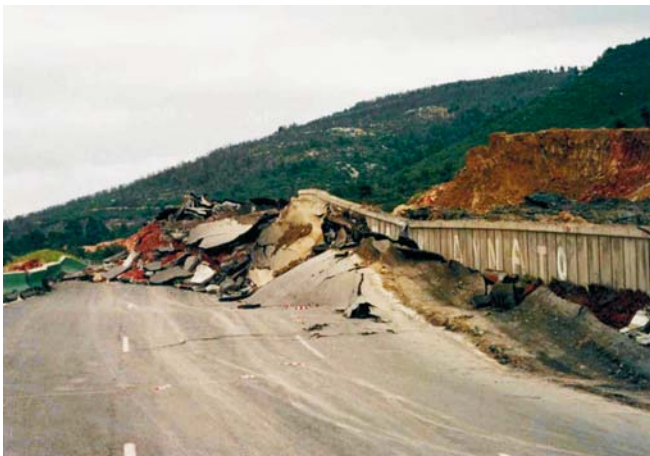
Fig. 37.6. Malakasa landslide, February 1995. Damages on the new highway from Athens to Thessaloniki. The landslide manifested in the tectonized and weathered zone of schists covered by debris
