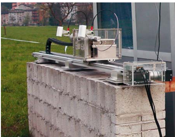
Fig. 43.3. Picture of the LiSA system installed in front of the Cortenova rock slide. The radar rail was placed on a concrete wall specifically built for the monitoring
