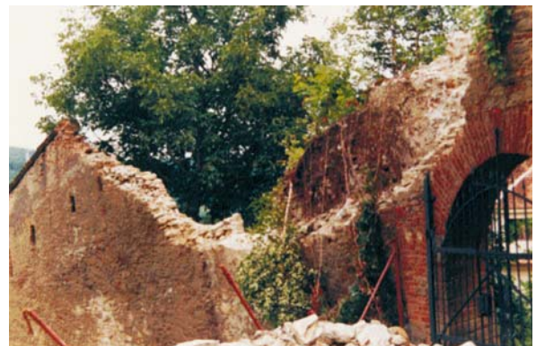
Fig. 45.5. The damage produced by a landslide on the citadel wall
