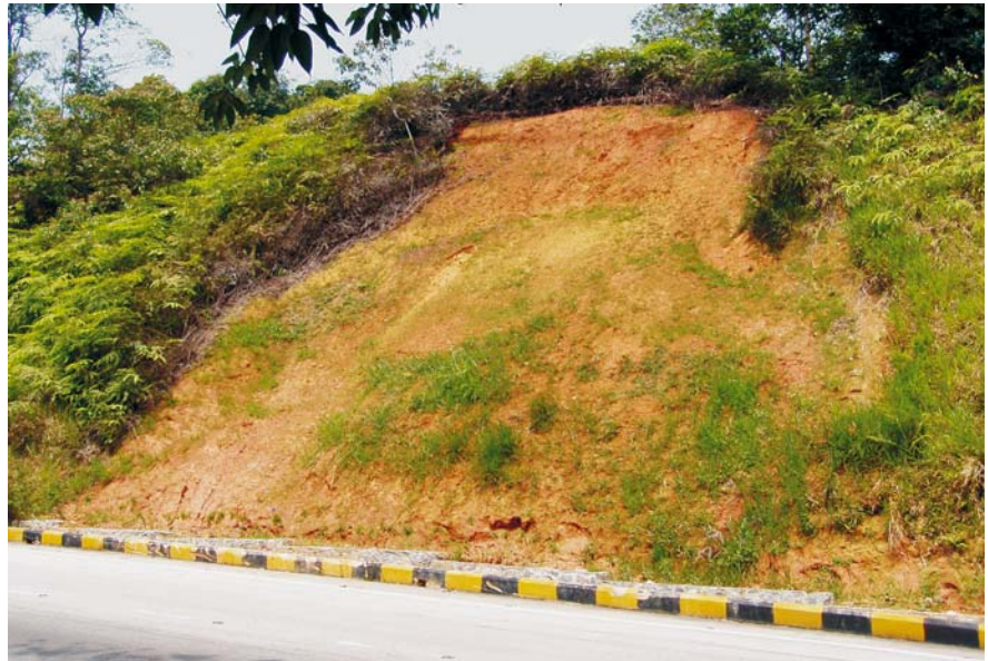
Fig. 24.6. Soil erosion feature at Fraser Hill
