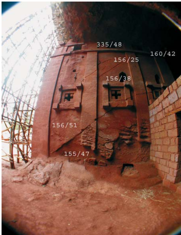
Fig. 26.8. The discontinuities detected on the lateral wall of Bet Aba Libanos; data refers to dip direction and dip
