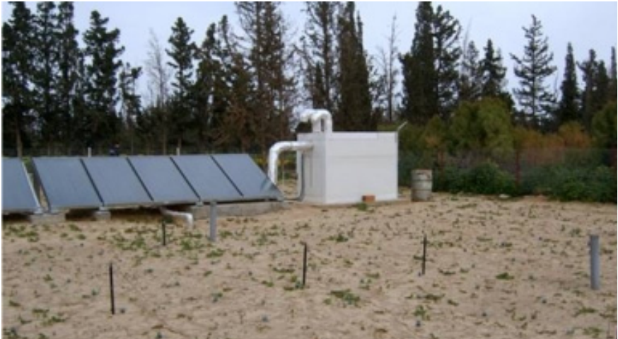
Figure 5: Pilot plant at the INRGREF in Tunisia. Ambient air is heated and humidified using solar collectors. The soil temperature and humidity are measured in the ground around drainage pipes.
