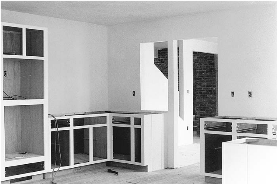
FIGURE 7.30 Prepainted wood kitchen cabinets installed before the installation of shelves, drawers, doors, and countertops. (Photo by Edward Allen)
