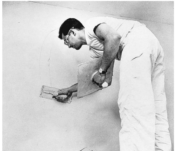
FIGURE 23.21 Applying veneer plaster with a hawk and trowel. (Courtesy of United States Gypsum Company)
