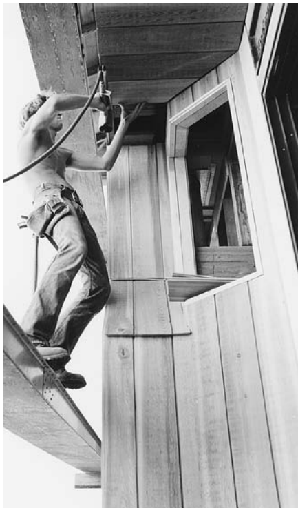
FIGURE 6.18 A carpenter applies V-groove tongue-and-groove redwood siding to an eave soffit, using a pneumatic nail gun. (Courtesy of Senco Products, Inc.)
