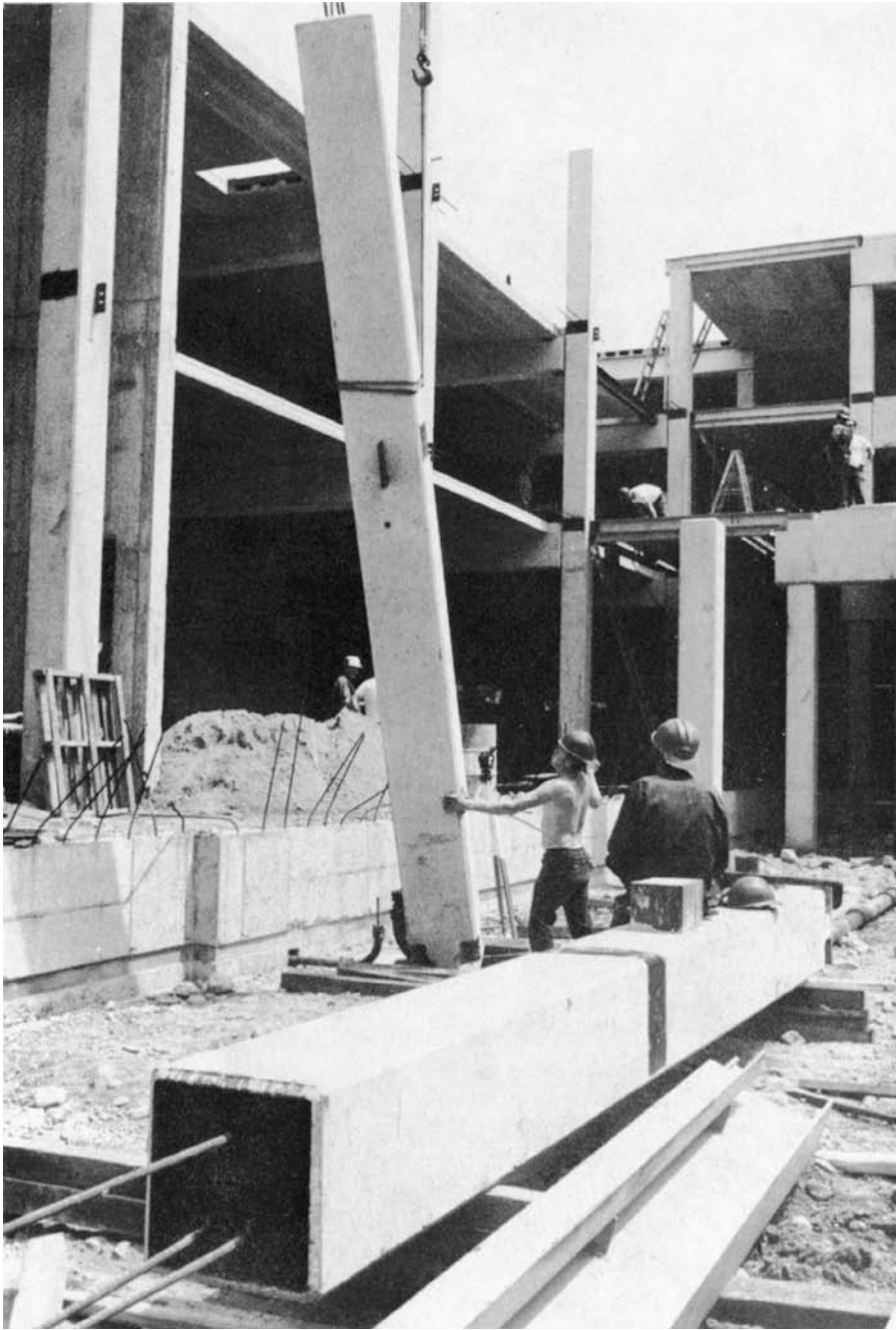
FIGURE 15.31 A precast column section is lifted from the ground by a crane. (Courtesy of Blakeslee Prestress, Inc.)
