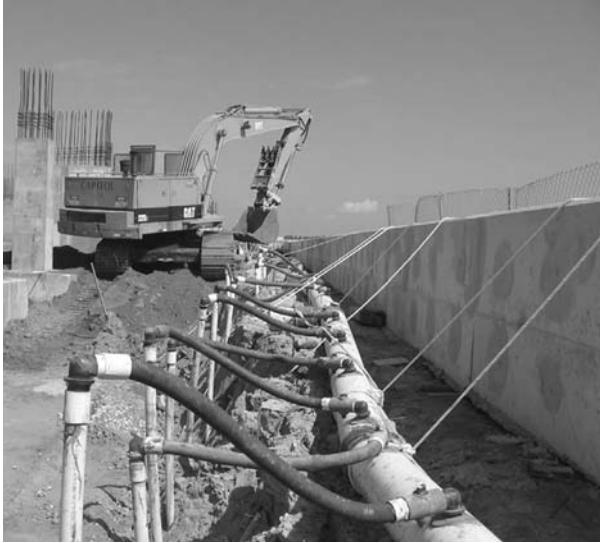
FIGURE 2.27 Well point dewatering. Closely spaced vertical well points connect to the larger-diameter header pipe. (Courtesy of Griffin Dewatering Corporation)
