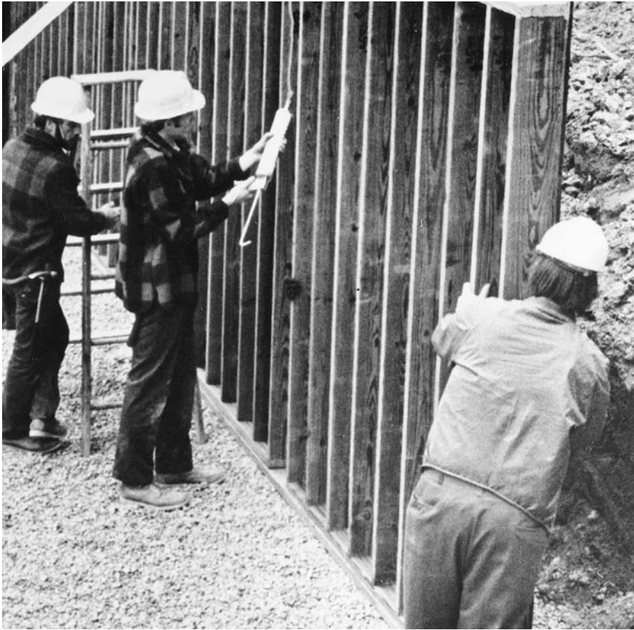
FIGURE 5.14 Erecting a permanent wood foundation. One worker applies a bead of sealant to the edge of a panel of preservative-treated wood components as another prepares to push the next panel into position against the sealant. The panels rest on a horizontal preservative-treated plank, which, in turn, rests on a drainage layer of crushed stone. Wood foundations can be constructed in any weather and can be insulated in the same way as the superstructure of the building. (Courtesy of APA—The Engineered Wood Association)
