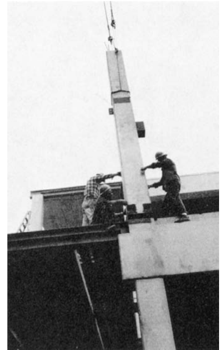
FIGURE 15.32 Erecting an upper-story column, using a connection of the type illustrated in Figure 15.14. (Courtesy of Blakeslee Prestress, Inc.)
