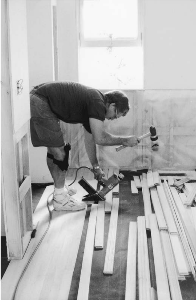
FIGURE 24.33 An installer of hardwood strip flooring uses a pneumatic nail gun to drive the diagonal blind nails that fasten the flooring to the subfloor. The nail gun is a special type that is activated by a blow from a mallet that also serves to drive the flooring pieces tightly together. Asphalt-saturated felt paper cushions the flooring and helps to prevent squeaking. (Photo by Rob Thallon)
