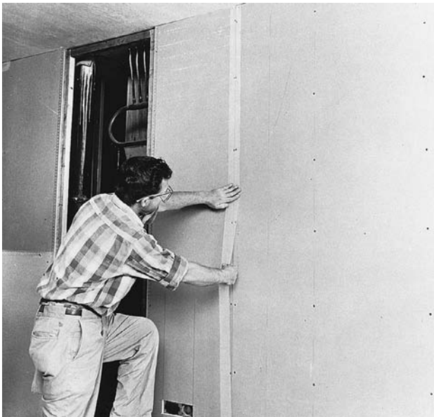
FIGURE 23.20 Reinforcing the panel joints of veneer plaster base with a self-adhesive glass fiber mesh tape. A panel opening for access to mechanical equipment is visible behind the installer. (Courtesy of United States Gypsum Company)
