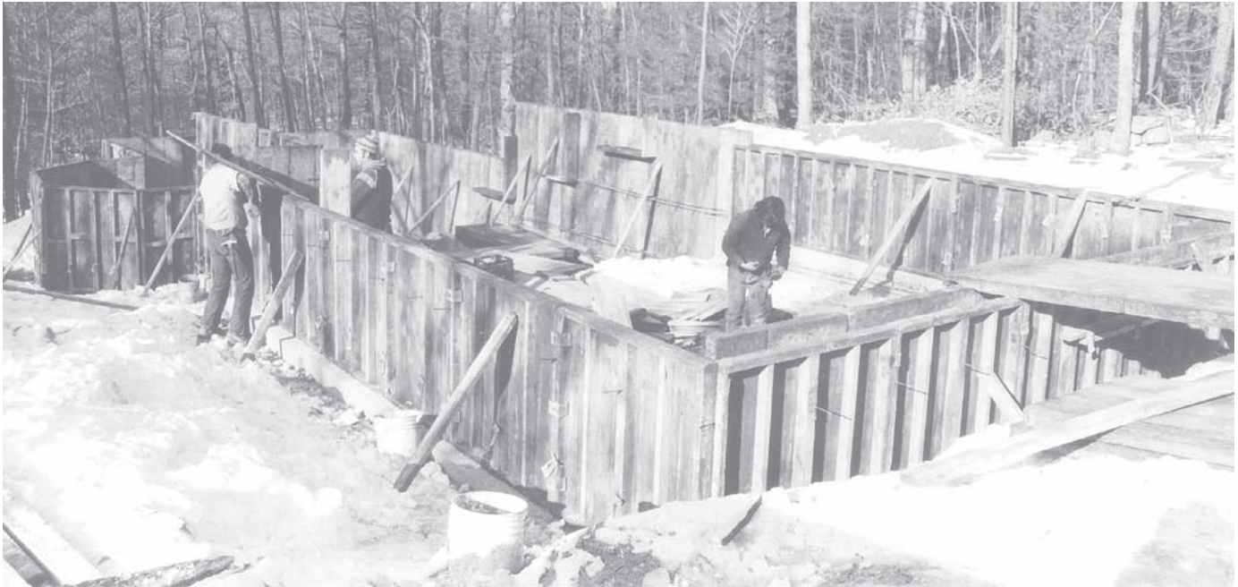
FIGURE 5.10 Erecting formwork for a sitecast concrete foundation wall. The footing has already been cast and its formwork removed. It is visible in front of the worker at the left. (Photo by Joseph Iano)
