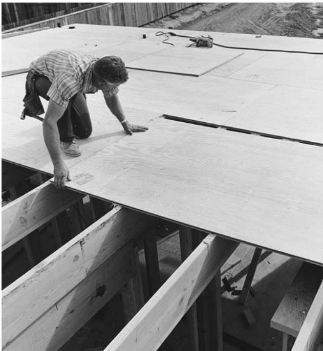
FIGURE 5.49 Installing upper-floor combination subflooring/underlayment. The grade of the plywood panels used is C-C Plugged. Its top (plugged) face has all surface voids filled and is lightly sanded, making it sufficiently smooth to allow carpeting to be installed directly over the subfloor without additional underlayment. The long edges of the panels have interlocking tongue-and-groove joints to prevent deflection of panel edges under a heavy concentrated load such as a standing person or the leg of a piano. (Courtesy of APA—The Engineered Wood Association)
