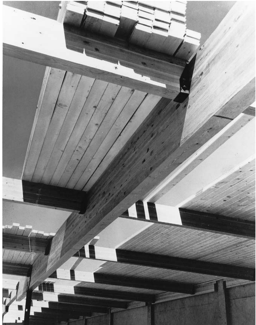
FIGURE 4.20 Installing tongue-and-groove roof decking over laminated beams and girders. (Courtesy of American Institute of Timber Construction)
