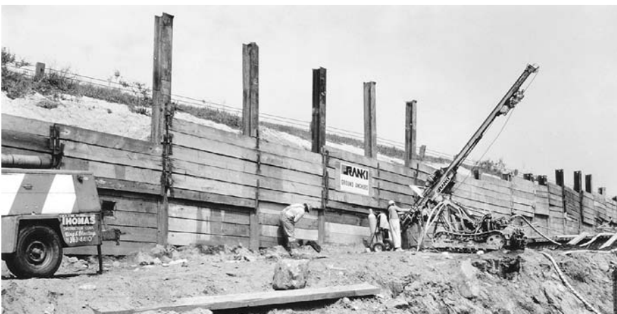
FIGURE 2.12 Soldier beams and lagging. Lagging planks are added at the bottom as excavation proceeds. The drill rig is boring a hole for a tieback to brace a soldier beam. (Courtesy of Franki Foundation Company)
