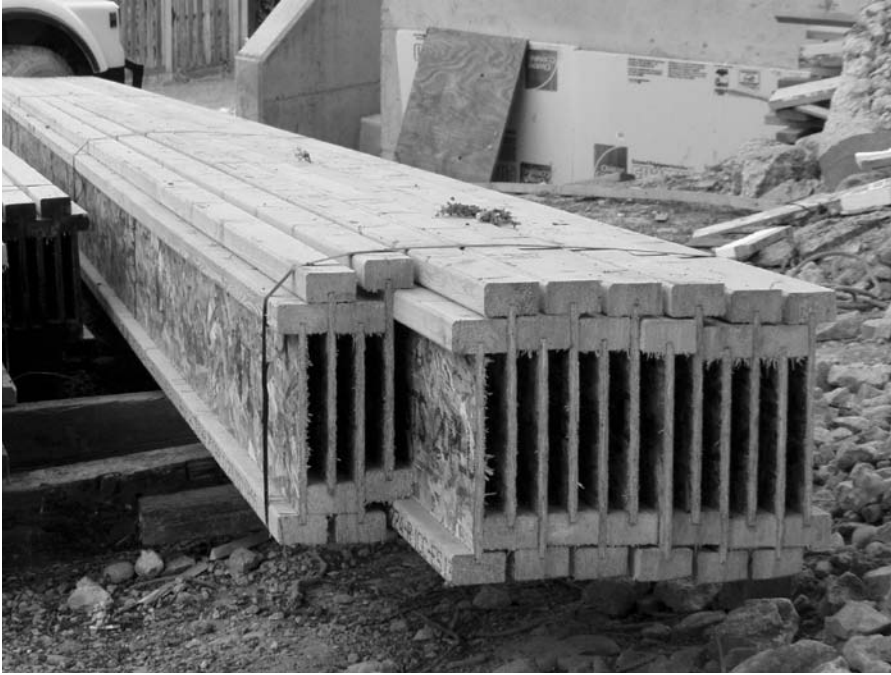
FIGURE 3.48 A bundle of I-joists delivered to the construction site. The webs are made from OSB and the flanges from solid lumber. (Photo by Joseph Iano)
