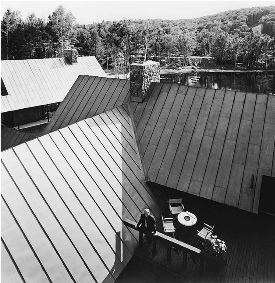
FIGURE 16.48 Standing-seam copper roofs. (Designer: Emil Hanslin. Courtesy of Copper Development Association, Inc.)
