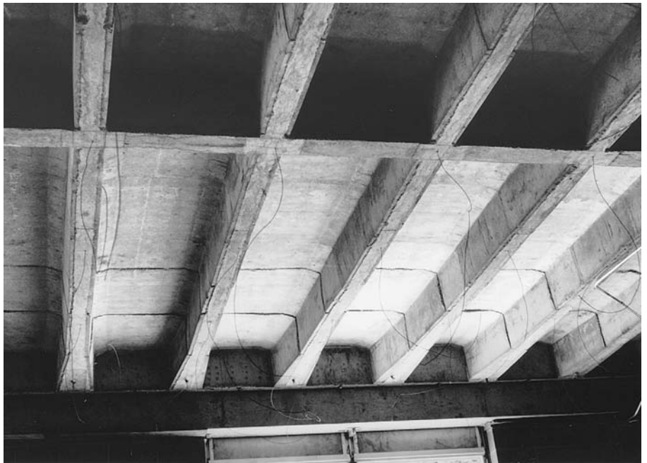
FIGURE 14.25 A one-way concrete joist system after stripping of the formwork, showing broadened joist ends at the lower edge of the photograph and a distribution rib in the foreground. The dangling wires are hangers for a suspended finish ceiling (see Chapter 24). (Reprinted with permission of the Portland Cement Association from Design and Control of Concrete Mixtures , 12th edition; Photos: Portland Cement Association, Skokie, IL)
