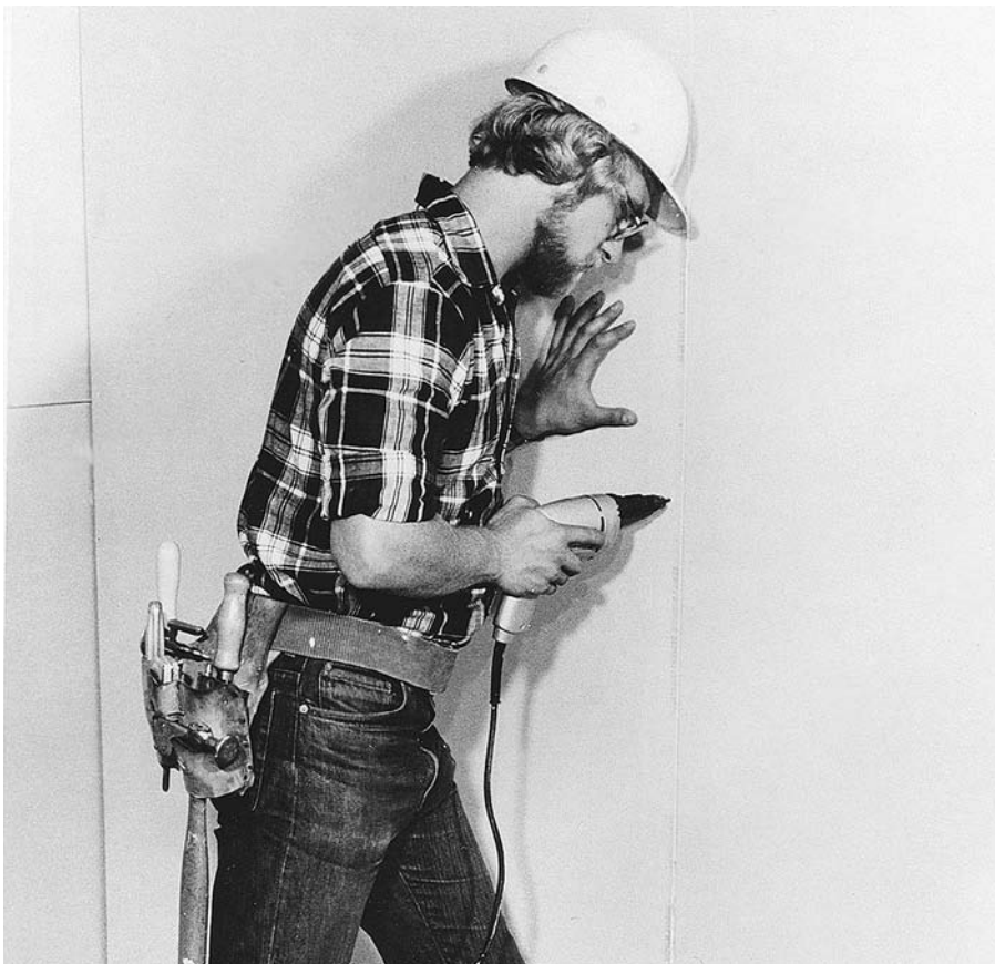
FIGURE 23.25 Attaching gypsum board to studs with a screw gun. (Courtesy of United States Gypsum Company)
