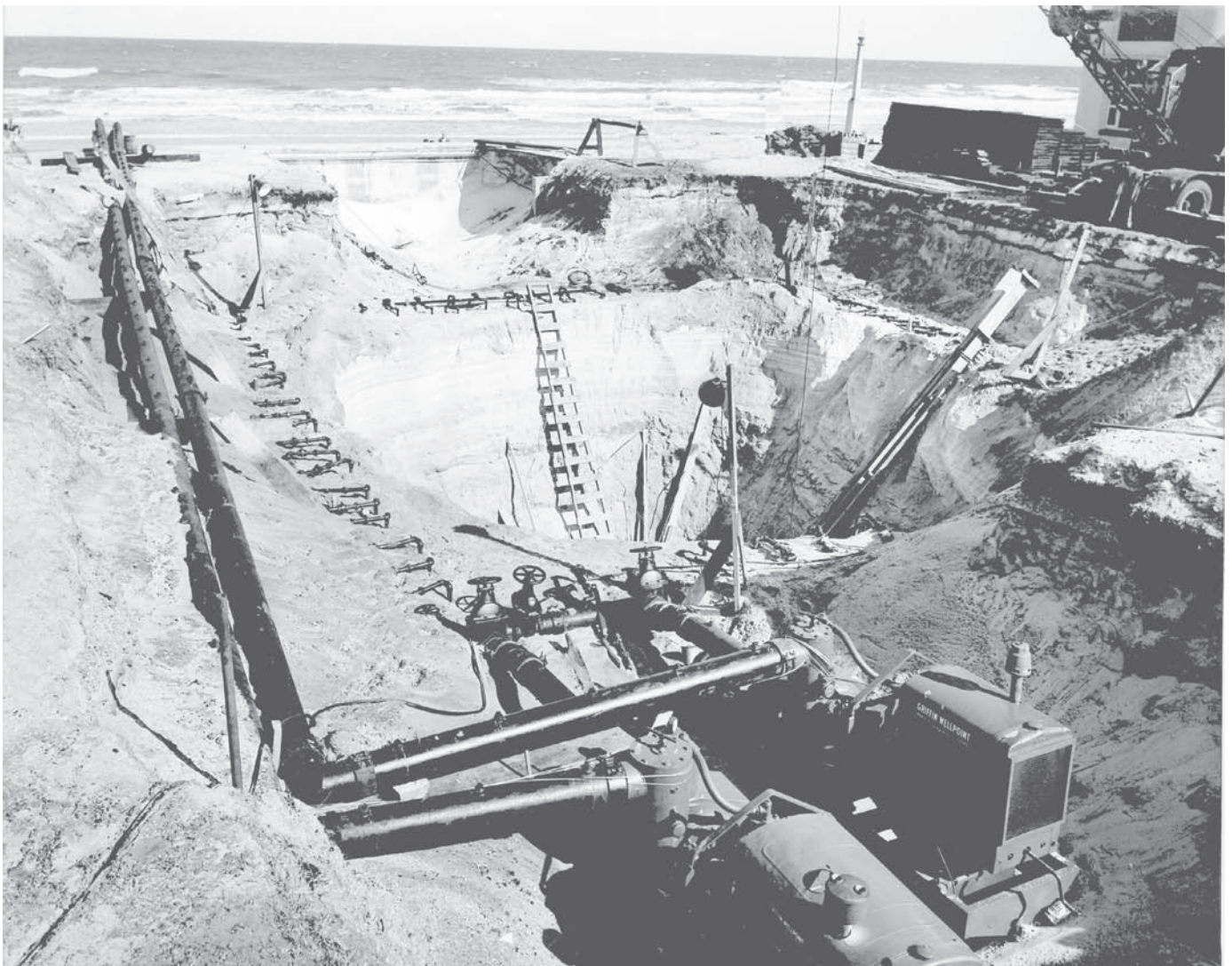
FIGURE 2.28 An excavation is kept dry despite the close proximity of a large body of water. Two dewatering pumps are visible in the foreground. A pair of header pipes and numerous well points can be seen surrounding the excavation. (Courtesy of Griffin Dewatering Corporation)
