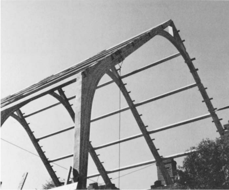
FIGURE 4.22 Three-hinged arches of glue-laminated wood carry laminated wood roof purlins. The short crosspieces of wood between the purlins are temporary ladders for workers. (Courtesy of American Institute of Timber Construction)
