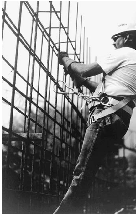
FIGURE 14.6 Protected against falling by a safety harness, a worker stands on the reinforcing bars for a concrete wall to wire another horizontal bar in position. (Photo courtesy of DBI/SALA, Red Wing, Minnesota)
