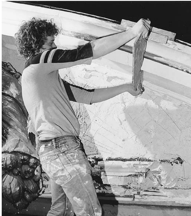
FIGURE B Running a plaster cornice molding in place. (Courtesy of Dovetail, Inc.)
