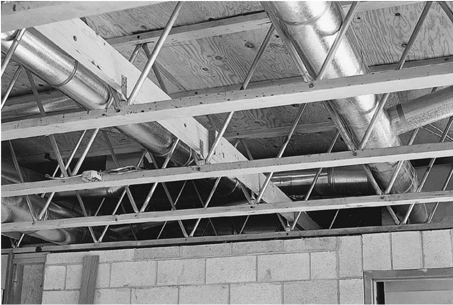
FIGURE 7.9 Ductwork and electrical wiring are installed conveniently through the openings in these floor trusses, making it easy to apply a finish ceiling if desired. The 2 × 6 that runs through the trusses in the center of the photograph is a bridging member that restrains the trusses from buckling. (Courtesy of Trus Joist Corporation)
