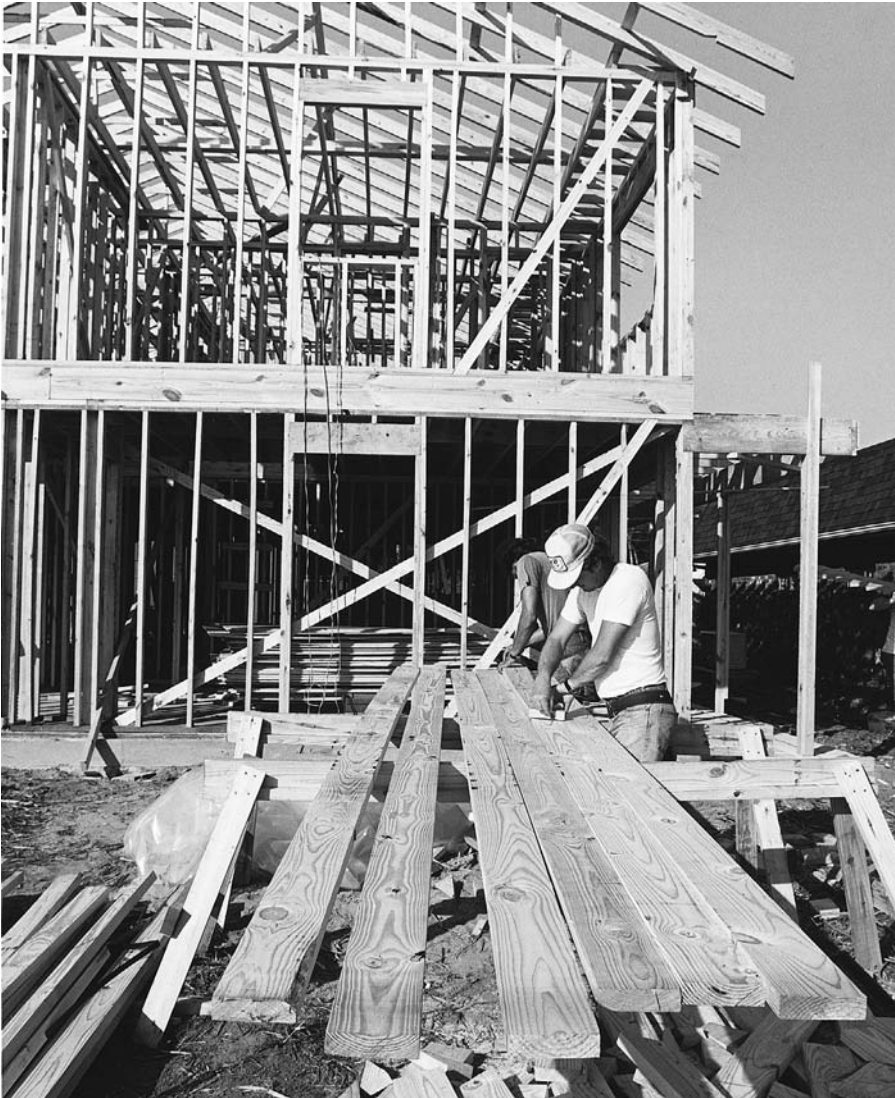
FIGURE 5.59 Tracing a pattern rafter to mark cuts for the rest of the rafters. The corner of the building behind the carpenters has let-in corner braces on both floors, and most of the rafters are already installed. (Courtesy of Southern Forest Products Association)
