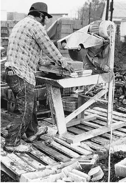
FIGURE 9.25 Concrete blocks and bricks can be cut very accurately with a water-cooled, diamond-bladed saw. For rougher sorts of cuts, a few skillful blows from the mason's hammer will suffice. (Reprinted with permission of the Portland Cement Association from Design and Control of Concrete Mixtures , 12th edition; photos: Portland Cement Association, Skokie, IL)
