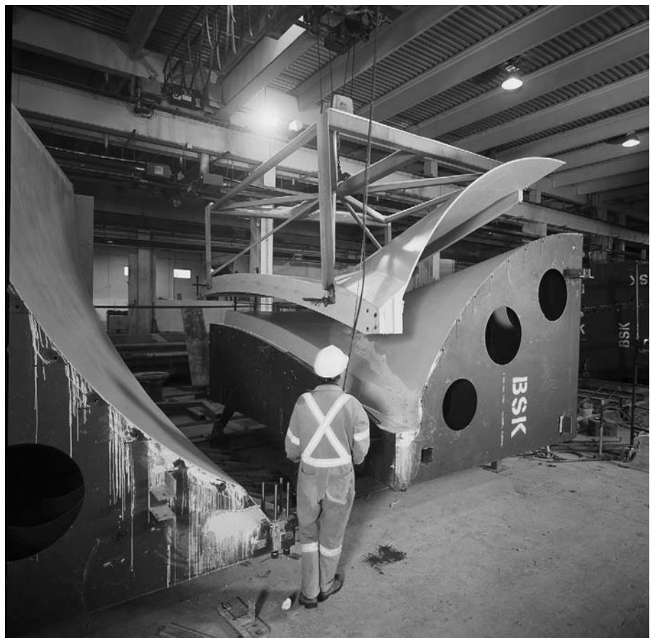
FIGURE 13-44 Casting of a concrete shell for the Shawnessy LRT Station shown in the previous figure. The shells were injection molded, a technique in which the concrete is cast in a fully enclosed mold rather than in a conventional open-sided form. In this photograph, the two halves of a mold have been separated, and the shell is being lifted with the aid of a temporary frame. (Courtesy of Lafarge North America, Inc. Photography by Tucker Photography)
