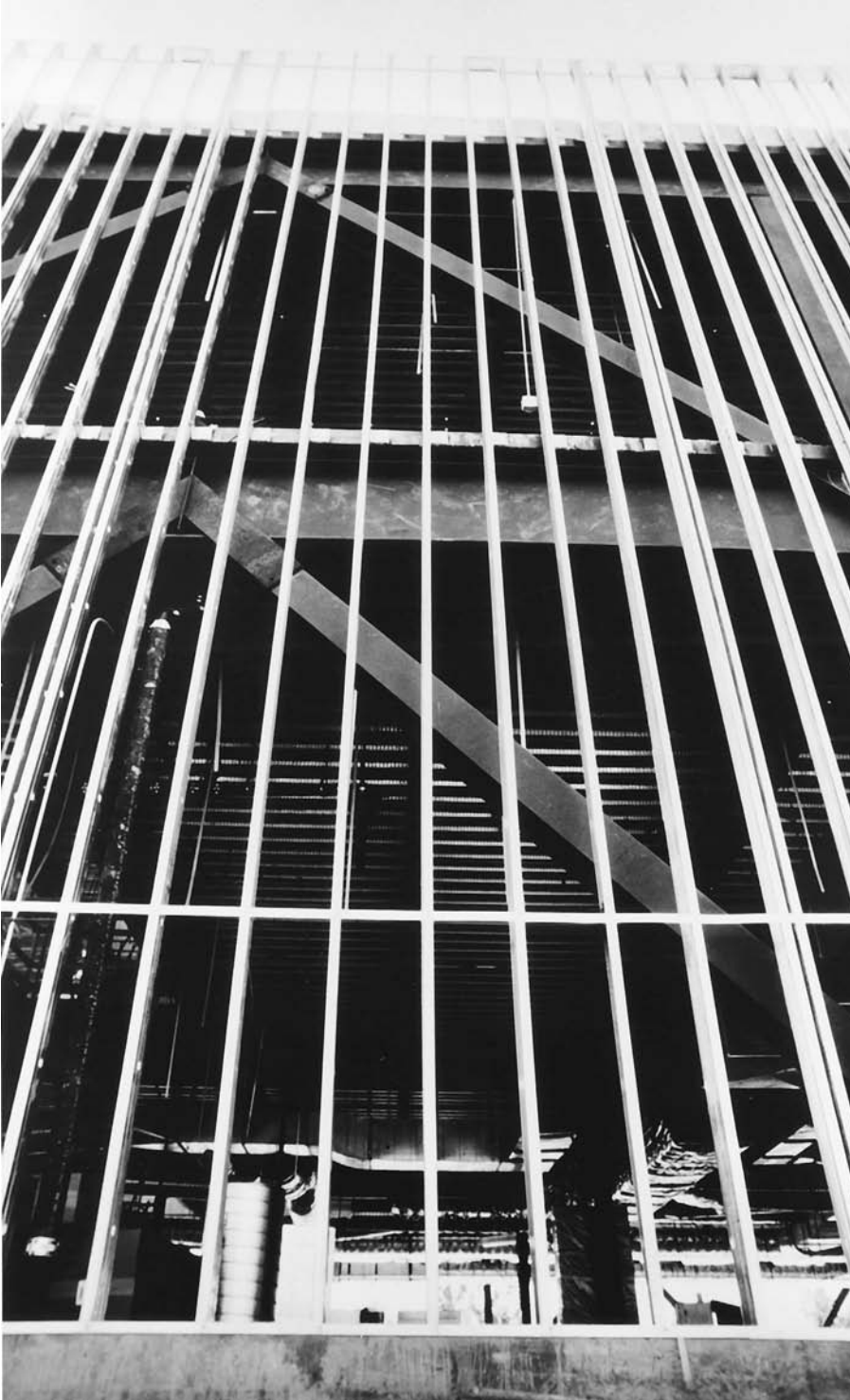
FIGURE 12.14 The straightness of steel studs is apparent in these tall walls that enclose a building framed with structural steel. (Courtesy of Unimast Incorporated— www.unimast.com )
