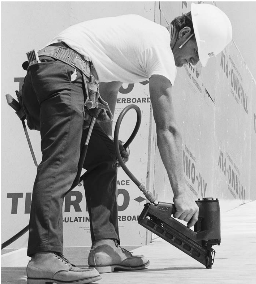
FIGURE 5.62 Fastening roof sheathing with a pneumatic nail gun. (Courtesy of Senco Products, Inc.)
