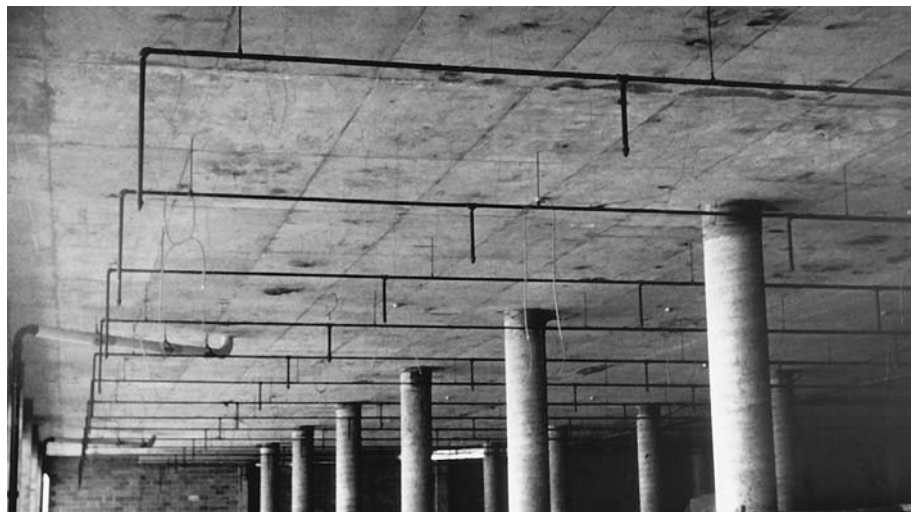
FIGURE 14.31 The underside of a two-way flat plate floor. Pipes have been installed for an automatic sprinkler fire suppression system. (Reprinted with permission of the Portland Cement Association from Design and Control of Concrete Mixtures , 12th edition; Photos: Portland Cement Association, Skokie, IL)
