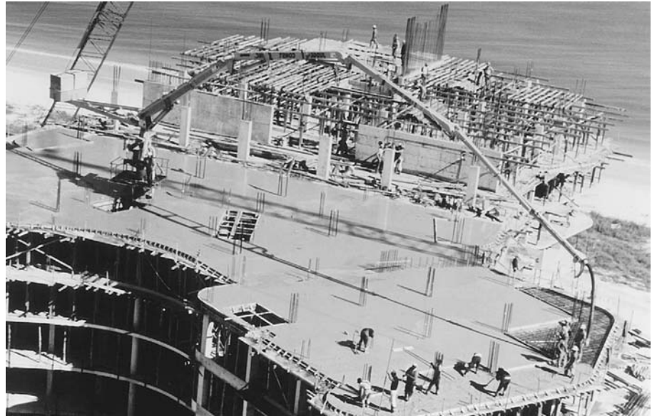
FIGURE 14.30 A two-way flat plate floor of a high-rise apartment building is poured with the aid of a concrete pump at the base of the building. The concrete is delivered up a telescoping tower to a nozzle at the end of an articulated boom. The column dowels in the center of the newly poured area demonstrate the ability of flat plate construction to adapt to irregular patterns and spacings of columns. (Courtesy of Schwing America, Inc.)
