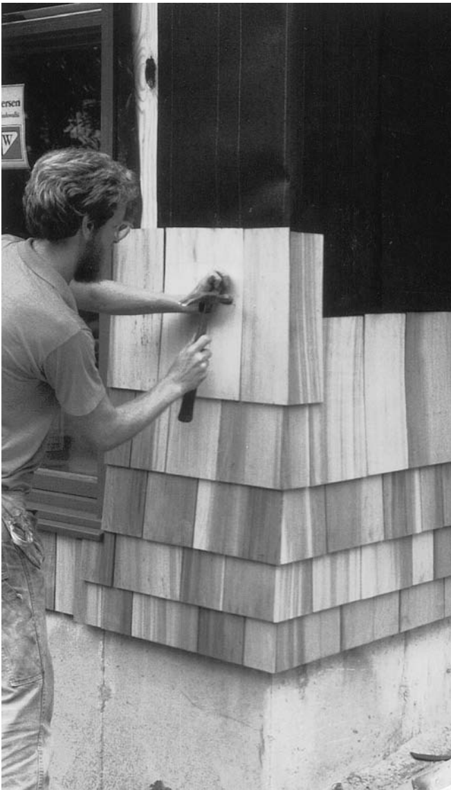
FIGURE 6.22 Applying wood shingle siding over asphalt-saturated felt building paper. The corners are woven as illustrated in Figure 6.24. (Photo by Edward Allen)
