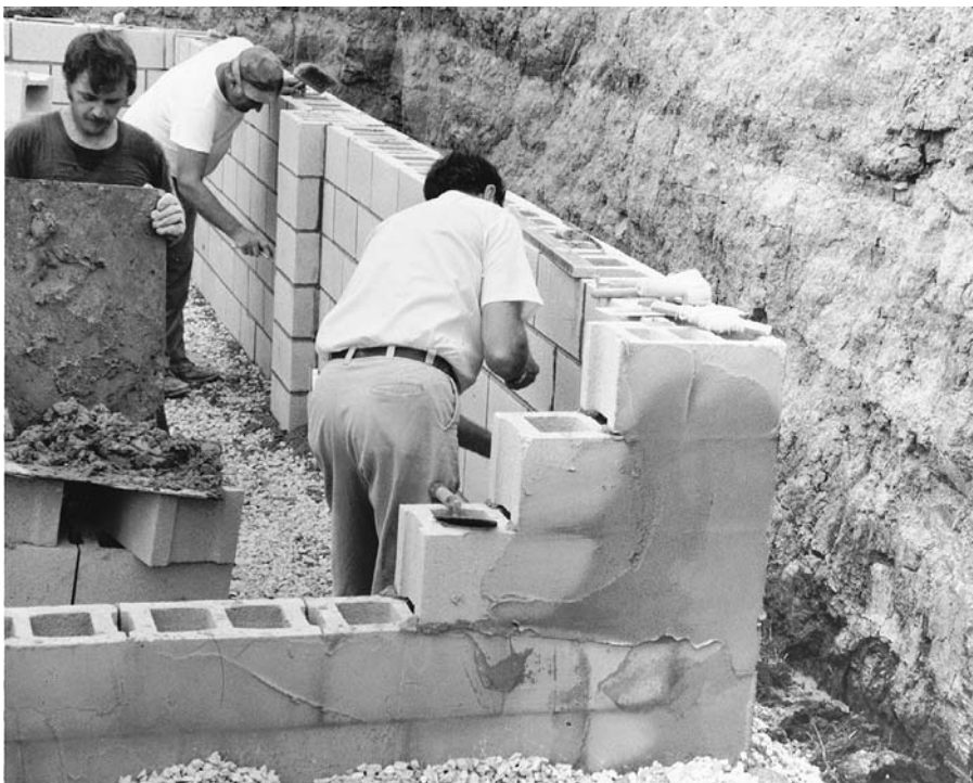
FIGURE 5.11 Masons construct a foundation of concrete masonry. The first coat of parging, which is portland cement plaster applied to help dampproof the foundation, has already been applied to the outside of the wall, and the drainage layer of crushed stone has been backfilled in place. The projecting pilaster in the center of the wall will support a beam under the center of the main floor. After a second coat of parging, the outside of the foundation will be coated with an asphaltic dampproofing compound. (Reprinted with permission of the Portland Cement Association from Design and Control of Concrete Mixtures, 12th edition; Photos: Portland Cement Association, Skokie, IL)
