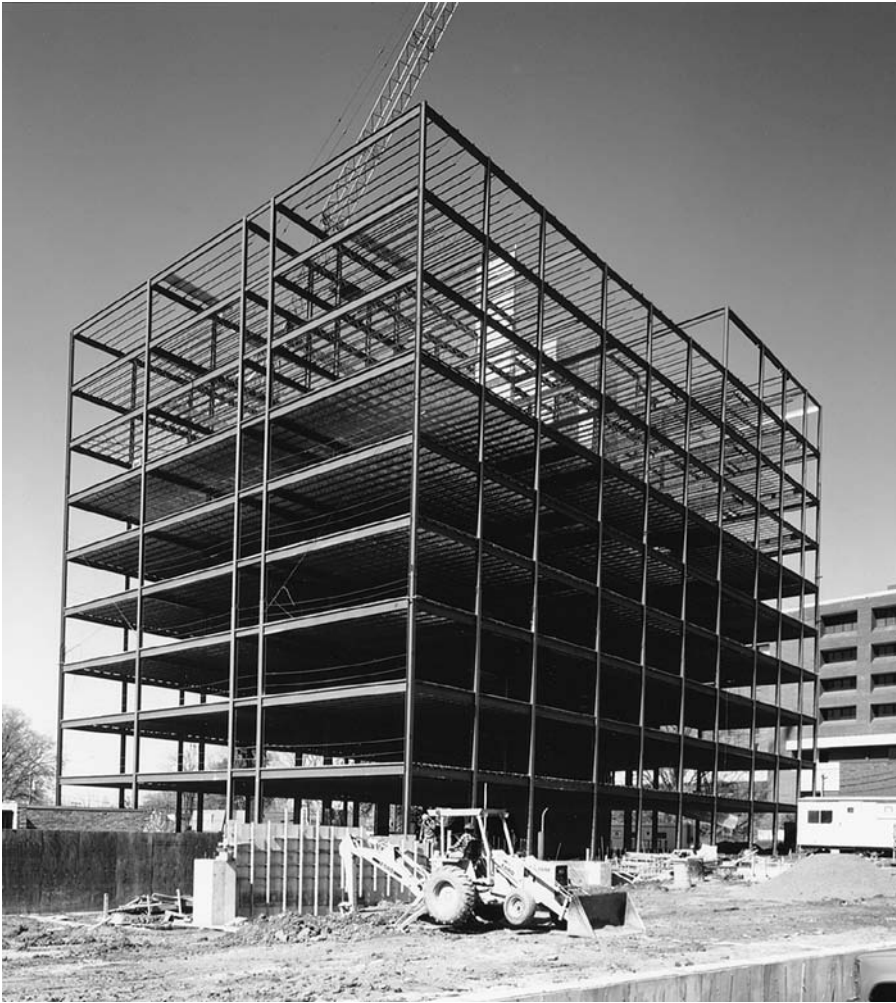
FIGURE 11.57 A 10-story steel frame nears completion. The lower floors have already been decked with corrugated steel decking. (Courtesy Vulcraft Division of Nucor)
