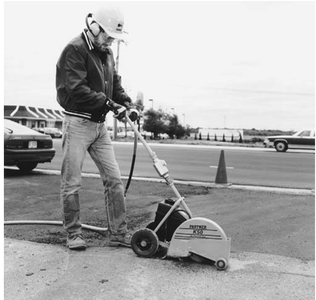
FIGURE C A pneumatically powered diamond circular saw slices a control joint in a concrete pavement. (Courtesy of Partner Industrial Products, Itasca, Illinois)
