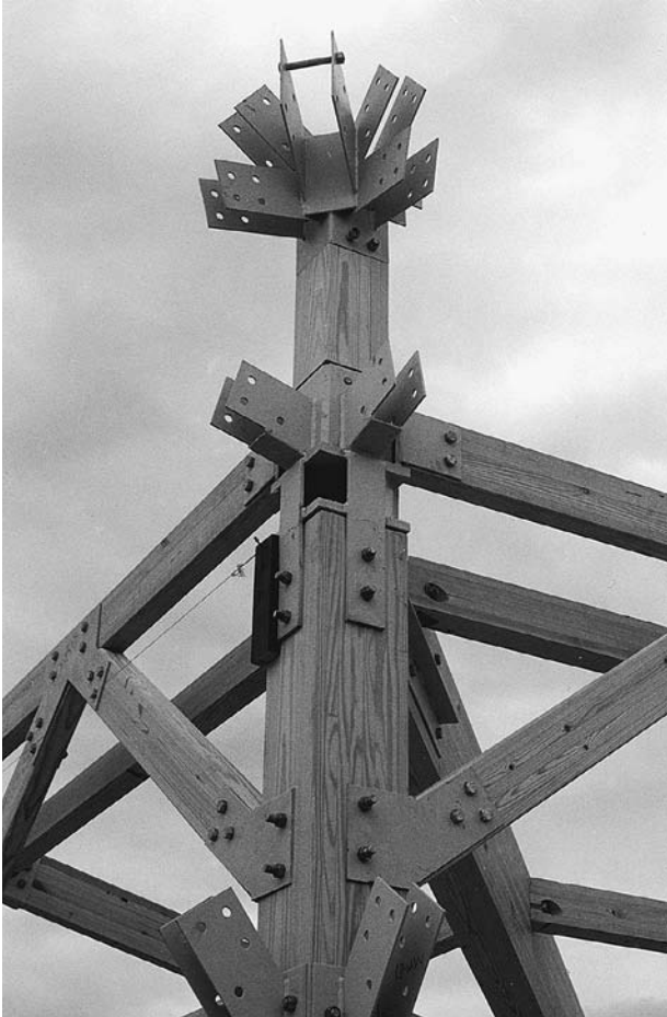
FIGURE 4.28 The Montville Public Library timbers are joined with custom-designed connectors that are welded together from steel plates. (Design and photographs by Eliot Goldstein, The Goldstein Partnership, Architects)
