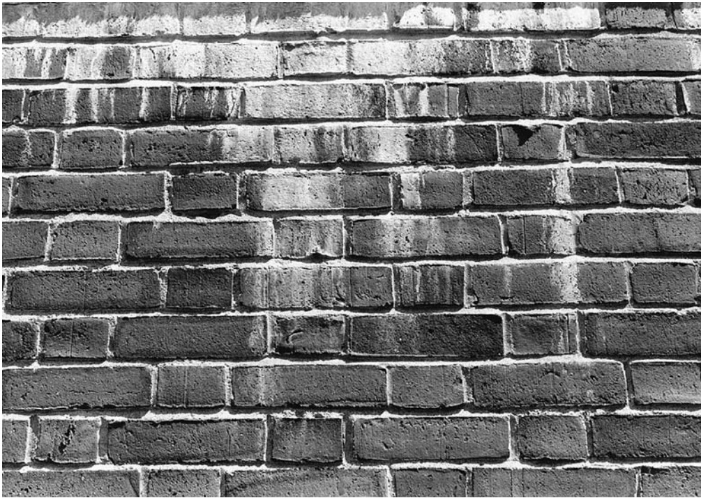
FIGURE 10.22 Efflorescence on a wall of Flemish bond brickwork. (Photo by Edward Allen)
