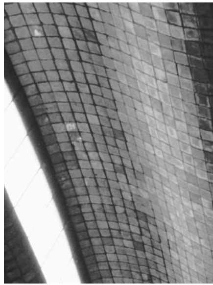
FIGURE 8.46 During the second half of the 20th century, Uruguayan engineer Eladio Dieste constructed hundreds of industrial buildings with long-span roof vaults of reinforced clay masonry, either bricks or, like the example shown here, hollow clay tiles. The span of this roof is about 100 feet (30 m). (Left) The vaults are long strips with clerestory windows between for daylighting. (Right) Each strip is S-shaped in cross section. This stiffens the vault to prevent buckling and also provides the openings for the windows. (Photos by Edward Allen)
