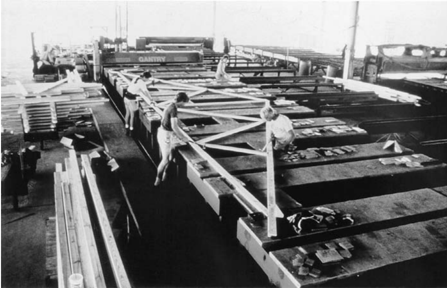
FIGURE 3.47 Manufacturing and transportation of wood trusses. (a) Factory workers align the wood members of a roof truss and position toothed-plate connectors over the joints, tapping them with a hammer to embed them slightly and keep them in place. The roller marked “Gantry” then passes rapidly over the assembly table and presses the plates firmly into the wood. (b) The trusses are transported to the construction site on a special trailer. (c) Trusses can be designed and produced in almost any configuration. (Photos courtesy of Wood Truss Council of America)
