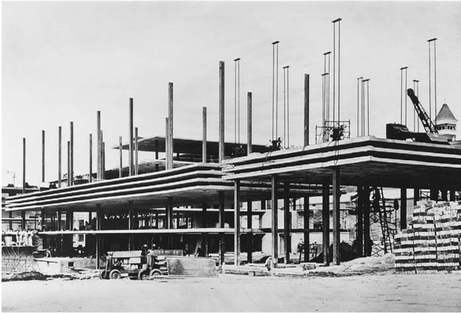
FIGURE 14.45 Lift-slab construction in progress. The paired steel rods silhouetted against the sky to the right are part of the lifting jacks seen at the tops of the columns. In North America, this form of construction is used infrequently, in part due to a history of past construction accidents. (Reprinted with permission of the Portland Cement Association from Design and Control of Concrete Mixtures, 12th edition; Photos: Portland Cement Association, Skokie, IL)
