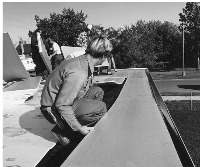
FIGURE 16.7 Installing extruded polystyrene foam insulation over a roof membrane to create a protected membrane roof. (Photograph provided by the Dow Chemical Company)
