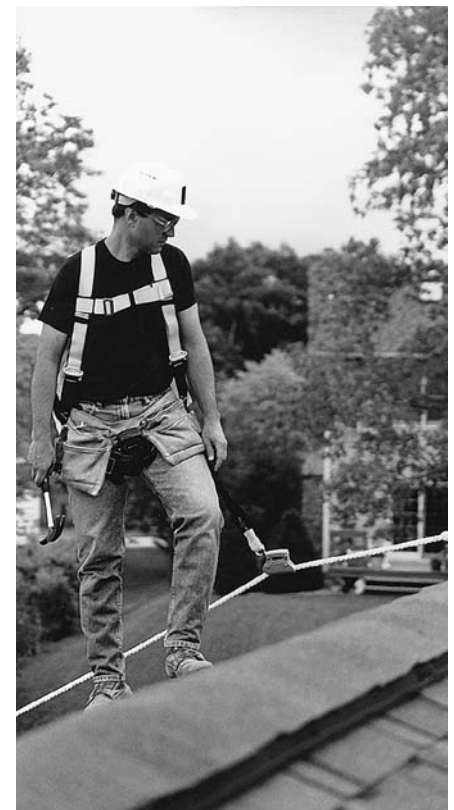
FIGURE 16.47 Protective devices keep workers from falling long distances off steep roofs. (Courtesy of DBI/SALA, Red Wing, Minnesota)
