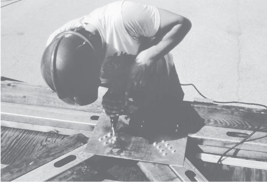
FIGURE 12.15 A worker tightens the last screws to complete a connection in a light gauge steel roof truss. The truss members are held in alignment during assembly by a simple jig made of plywood and blocks of framing lumber. (Courtesy of Unimast Incorporated— www.unimast.com )
