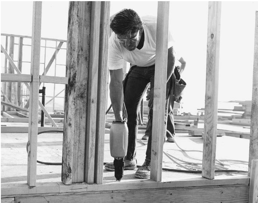
FIGURE 5.36 Fastening a wall to the floor platform. Horizontal blocking between studs as seen toward the left in this photo is typically installed to provide a solid substrate for the later attachment of bathroom hardware, exterior panels, or any number of possible other items. (Courtesy of Senco Products, Inc.)
