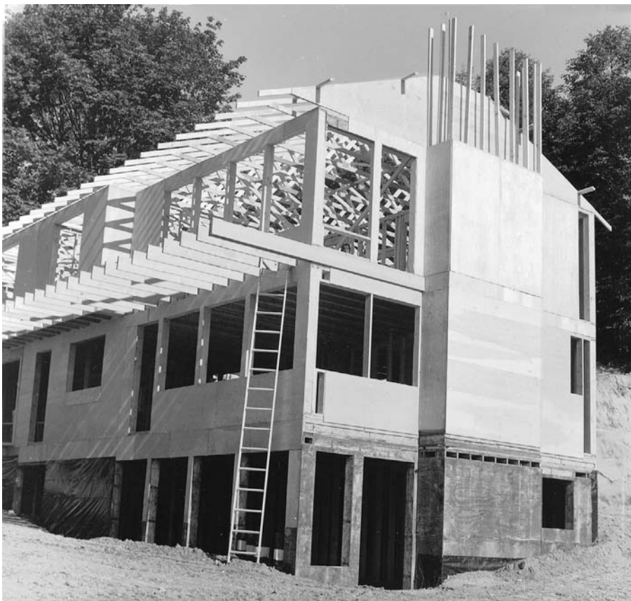
FIGURE 5.15 The difference in color makes it clear where the preservative-treated wood foundation leaves off and the untreated superstructure of the building begins. (Courtesy of APA—The Engineered Wood Association)
