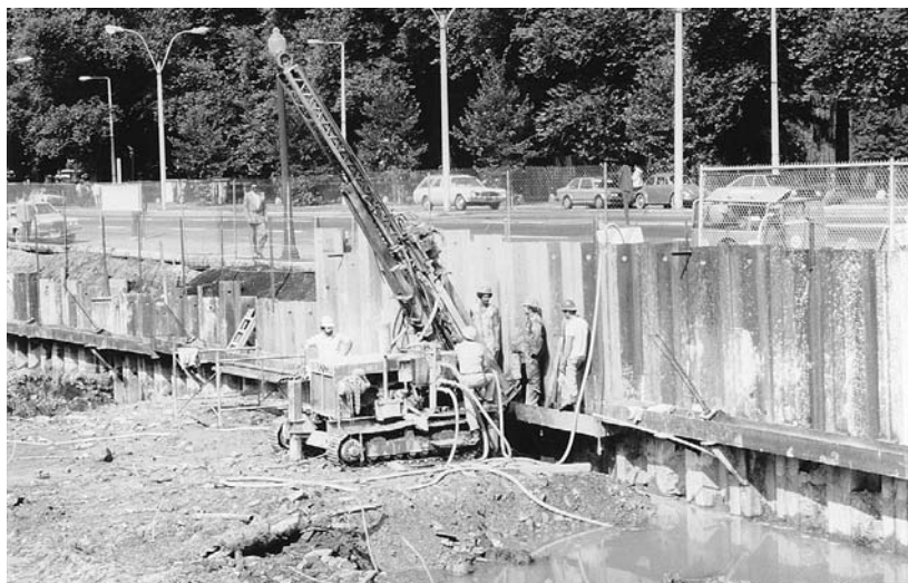
FIGURE 2.14 Drilling tieback holes for a wall of steel sheet piling. Notice the completed tieback connections to the horizontal waler in the foreground. The hole in the top of each piece of sheet piling allows it to be lifted by a crane. (Courtesy of Franki Foundation Company)
