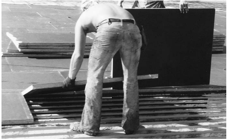
FIGURE 16.11 Workers bed rigid insulation boards in strips of hot asphalt over a corrugated metal roof deck. (Courtesy of GAF Corporation)
