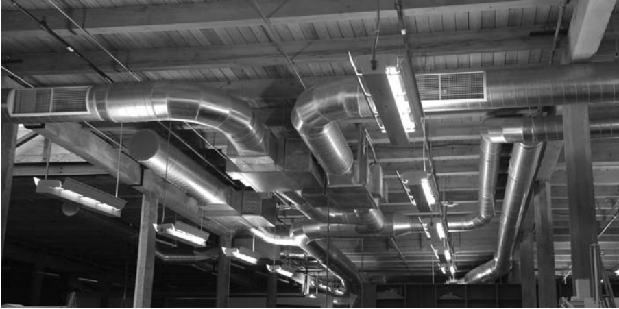
FIGURE 4.19 When floors and roofs are heavy timber framed, lighting, communications wiring, ductwork, fire sprinklers, and other services are exposed to view. (Photo by Joseph Iano)
