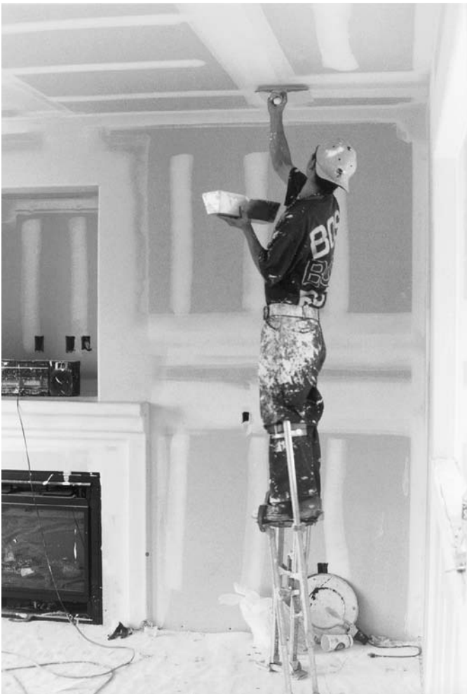
FIGURE 23.34 Plasterers and drywall finishers often work on stilts to avoid having to erect and move scaffolding. The stilts, which are strapped to the legs of the workers, are very sophisticated, stable devices that keep the worker's foot fully supported and parallel to the floor. (Photo by Rob Thallon)
