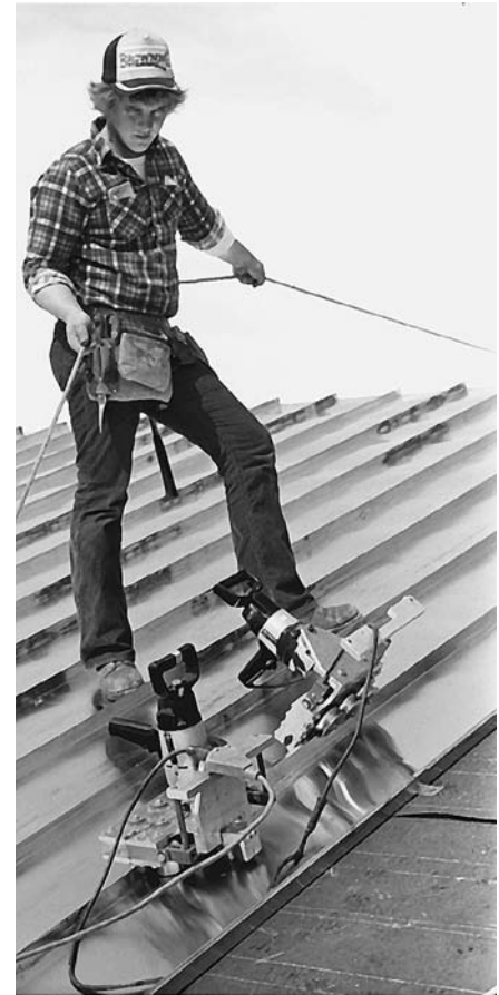
FIGURE 16.49 An automatic roll seamer, moving under its own power, locks standing seams in a copper roof. A cleat is just visible at the lower right. (Courtesy of Copper Development Association, Inc.)
