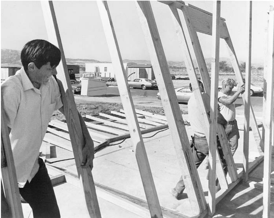
FIGURE 5.35 Tilting an interior partition into position. The gap in the upper top plate will receive the projecting end of the upper top plate from another partition that intersects at this point. (Courtesy of APA—The Engineered Wood Association)
