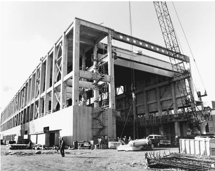
FIGURE 15.36 Precast concrete girders span the roof of a paper mill in British Columbia. (Engineer: Swan Wooster Engineering Co., Ltd. Courtesy of Precast/Prestressed Concrete Institute)
