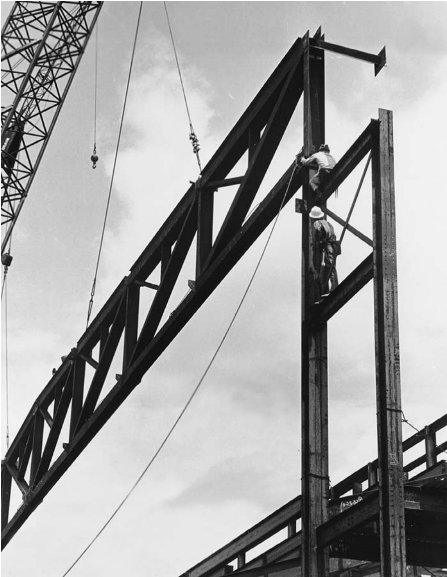
FIGURE 11.83 Ironworkers seat the end of a heavy roof truss made of wide-flange sections. (Permission of American Institute of Steel Construction)
