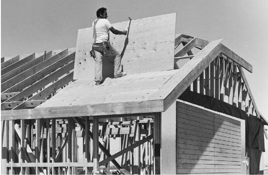
FIGURE 5.61 Applying plywood roof sheathing to a half-hipped roof. Blocking between rafters at the wall line (far left in the photo) has been drilled with large holes for attic ventilation. The line of horizontal blocking between studs is to support the edges of plywood siding panels applied in a horizontal orientation. (Courtesy of APA—The Engineered Wood Association)
