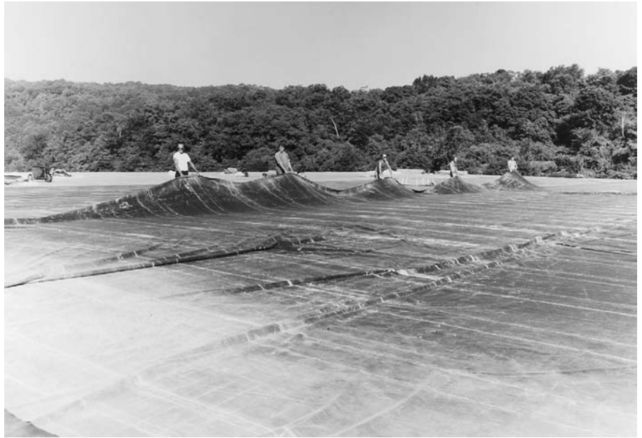
FIGURE 16.18 Workers unfold a large single-ply roof membrane. (Courtesy of Carlisle SynTec Systems)
