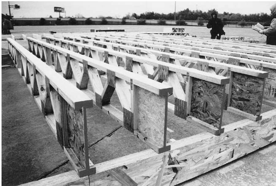
FIGURE 5.25 These floor trusses (shown here being set up for a demonstration house in a parking lot) are made of sawn lumber members joined by toothed-plate connectors. The OSB web at each end provides a section of truss that can be sawn by workers to easily adjust the length of the truss if necessary. Trusses are deeper than sawn joists or I-joists but can span farther. And even though they are deeper than other joist products, they may result in a thinner floor ceiling assembly, as pipes and ductwork can run through the passages within the truss rather than below it. (Courtesy of Wood Truss Council of America)
