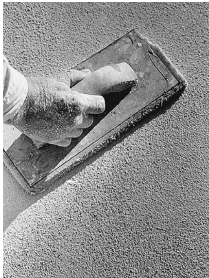
FIGURE 23.15 A sponge-faced float can be used to create various rough surface textures on plaster. (Reprinted with permission of the Portland Cement Association from Design and Control of Concrete Mixtures, 12th edition ; Photos: Portland Cement Association, Skokie, IL)
