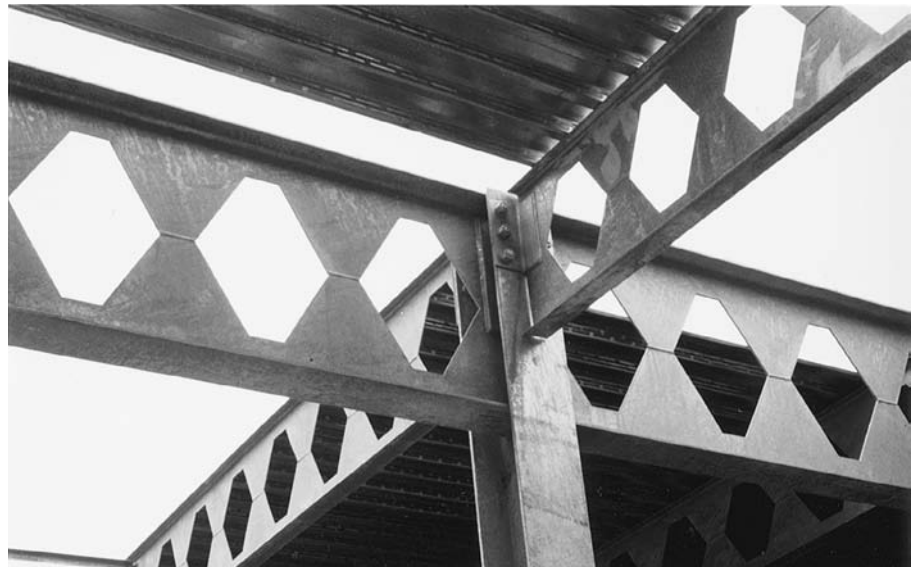
FIGURE 11.78 Castellated beams and girders frame into a wide-flange column. (Courtesy of Castelite Steel Products, Midlothian, Texas)
