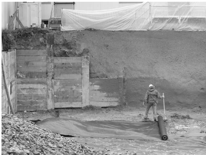
FIGURE 2.15 Where slope support turns the corner in this excavation and the soil can be sloped at a lesser angle, less expensive shotcrete takes the place of soldier beams and lagging. (Photo by Joseph Iano)
