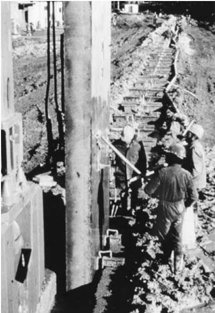
FIGURE 2.18 Workers apply a nonstick coating to a section of precast concrete slurry wall as it is lowered into the trench.
