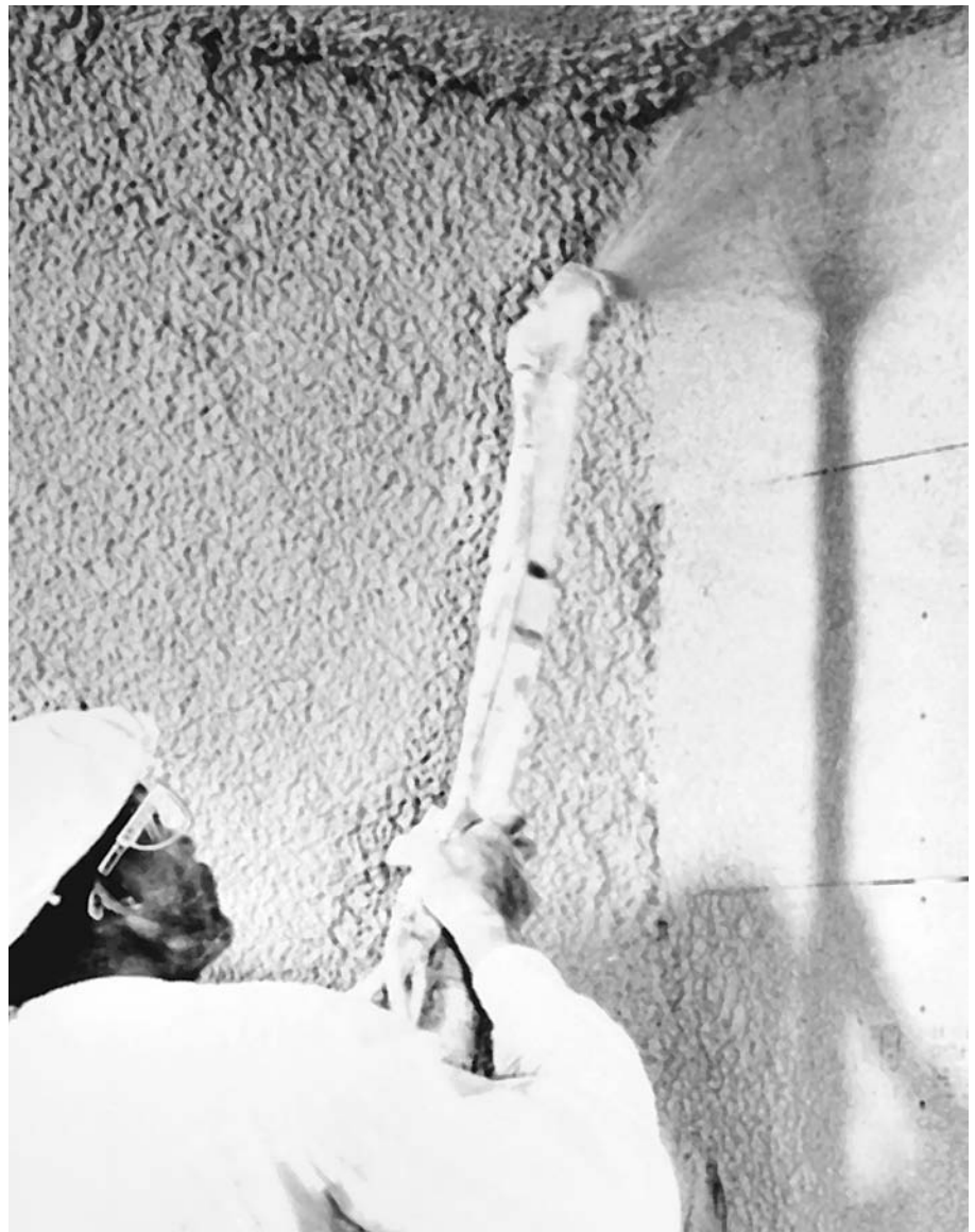
FIGURE 23.8 Spray applying a scratch coat of plaster to gypsum lath. (Courtesy of United States Gypsum Company)
