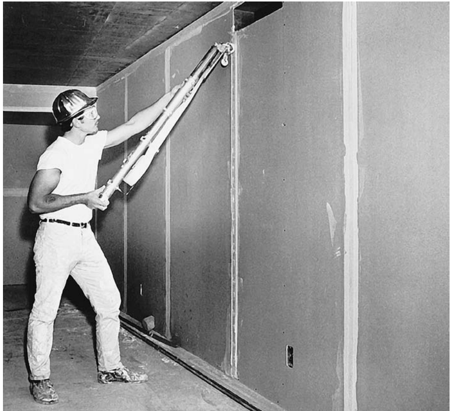
FIGURE 23.33 An automatic taper simultaneously applies tape and joint compound to gypsum board joints. (Courtesy of United States Gypsum Company)
