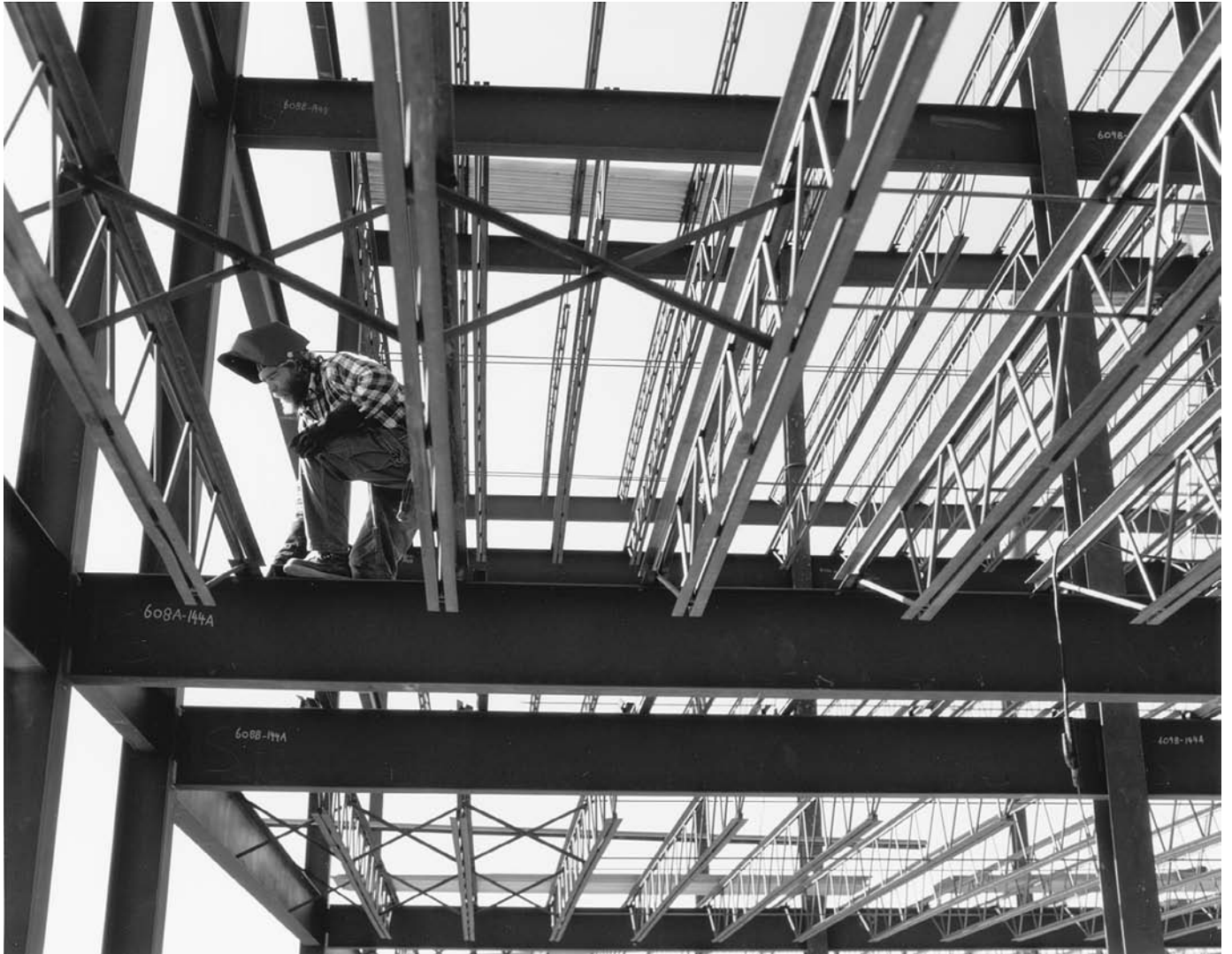
FIGURE 11.55 Welding open-web steel joists to a wide-flange beam. (Courtesy Vulcraft Division of Nucor)
