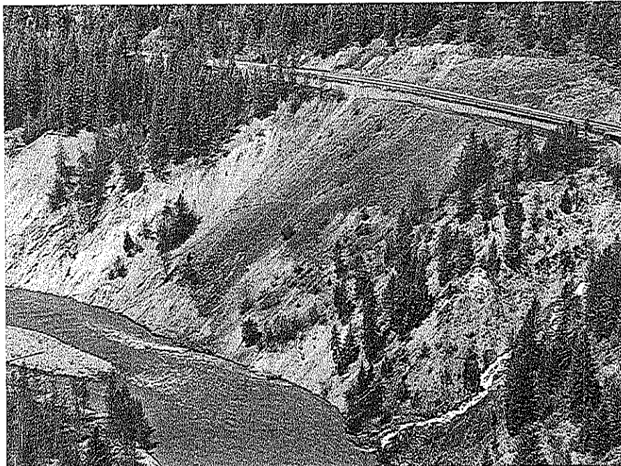
Figure CH-9.2 Goat Lick Slide. Highway 2 is supported by a reinforced earth wall. Below the wall, the slope is at 38° to the horizontal (Photo: May 14, 1993).
