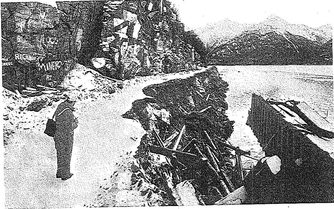
Figure CH-7.12 Skagway Marine Slide. View of the landslide headscarp from the end of the remaining wooden dock (Photo: November 14, 1994).
