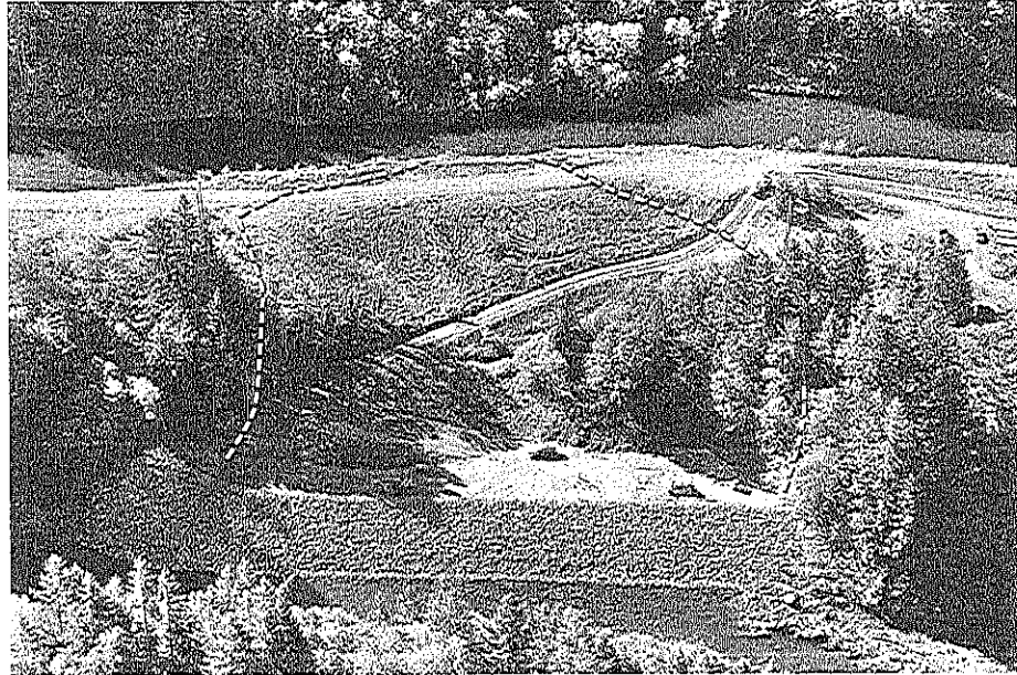
Figure CH-8.1 Faraday Slide. Rockfill buttress nearing completion. Outline of the landslide is shown by the dashed white line. Clackamas River in foreground; Faraday Canal at top of photograph (Photo: September 28, 1989).
