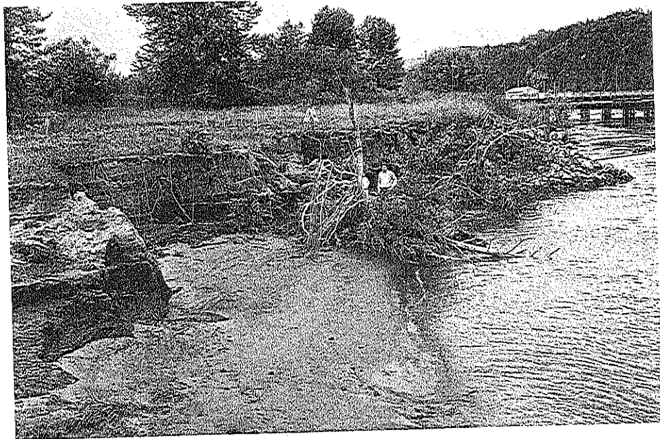
Figure CH-2.3 Beaver Shoreline Erosion. Erosion bowl with near-vertical faces of sand fill and "beach" of silt alluvium with thin covering of sand.
