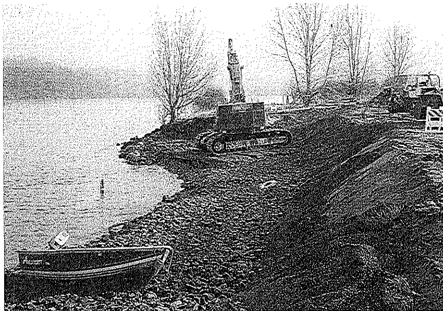
Figure CH-2.6 Beaver Shoreline Erosion. Beach area infilled with coarse filter to elev. +9 feet. Headscarp cut to 1.5:1 with fine filter partially spread on it. Trackhoe on timber spreaders at east end of project. D-7 dozer with winch is above trackhoe. In the foreground is a boat and lifebelt for safety purposes.
