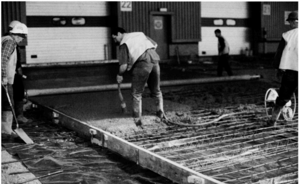
Fig. 5.81. The cracked slabs were broken out and reconstructed with mesh reinforcement placed near the upper surface of the slabs. Timber formwork was used with holes drilled for dowel bars
