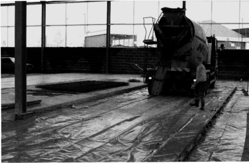
Fig. 5.27. A slip membrane has been laid and formwork has been fixed prior to concreting. The concrete truck reverses along the strip to the discharge position. Care has to be taken to avoid rutting the sub-base and disturbing the slip membrane. The mesh reinforcement cannot be installed prior to concreting as it would interfere with access
