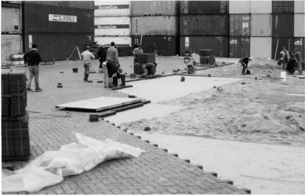
Fig. 5.112. Concrete block paving is being installed as an overlay on this container handling yard. Only 30% of the area needed to be taken out of service at any one time. By careful planning of both construction and container handling, disruption to the handling of containers was minimised
