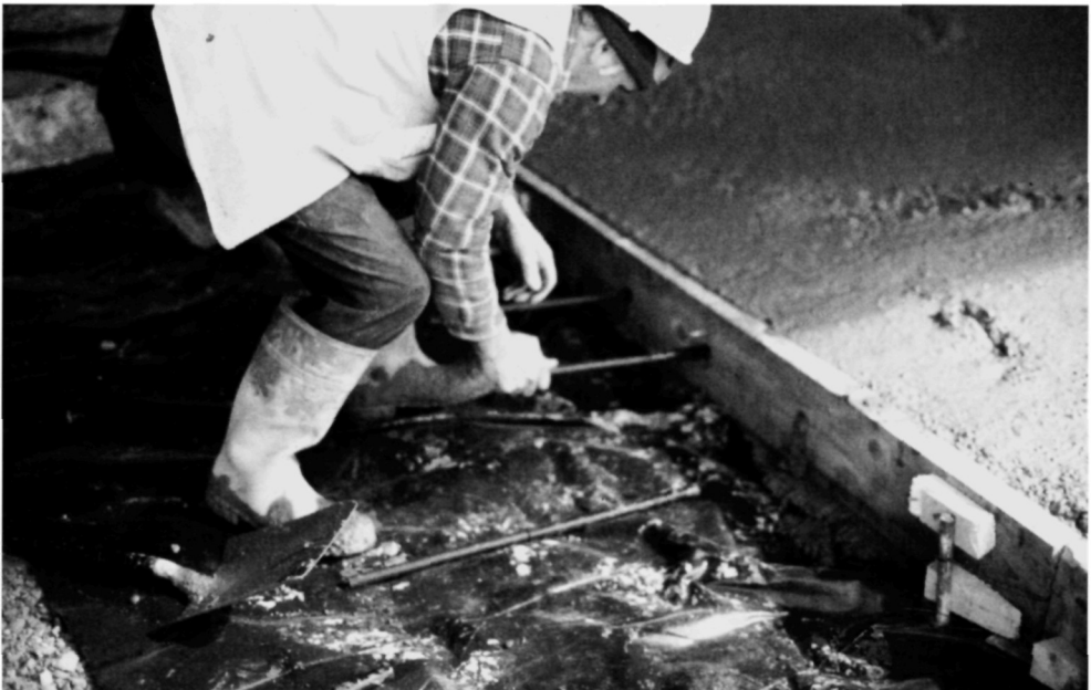
Fig. 5.85. Dowel bars are inserted into the holes drilled through the timber formwork. It can be difficult to ensure that all of the dowel bars remain parallel
