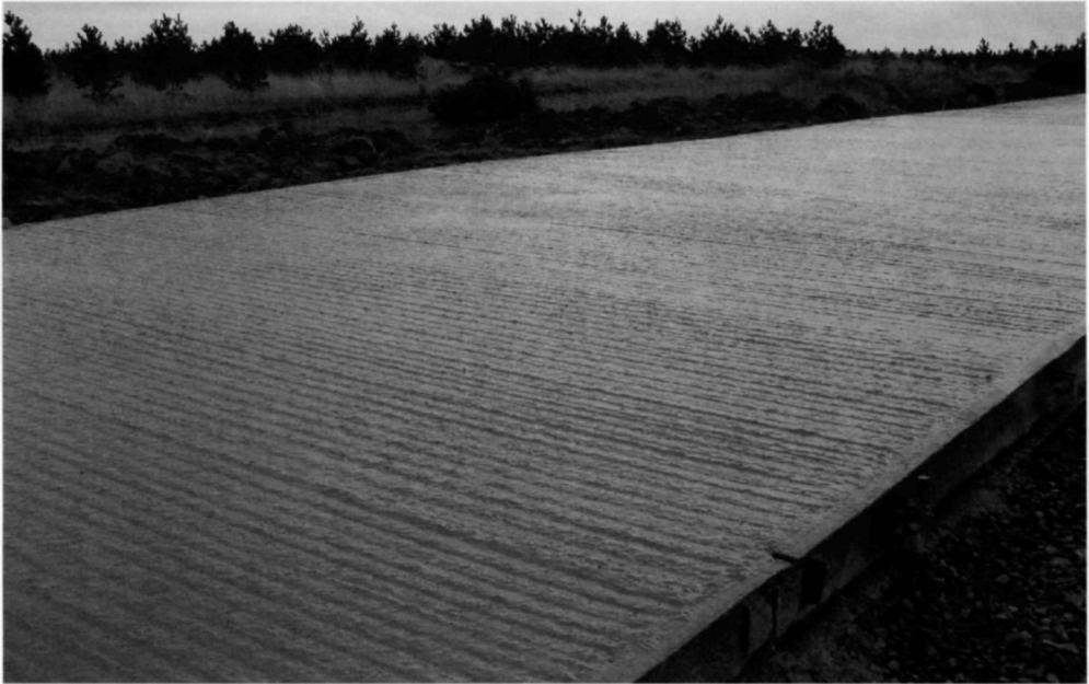
Fig. 5.70. The concrete has been compacted and a tamped finish has been introduced. This will ensure sufficient skid resistance. Curing compound is about to be sprayed on to the surface of the concrete
