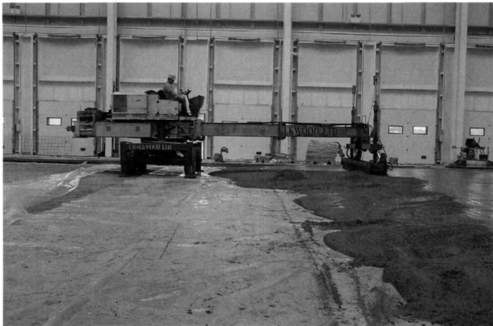
Fig. 5.15. Laser guided screeding machine spreading, compacting and finishing a large pour concrete slab. As the machine places the concrete, stabilising legs are extended so that the wheels no longer touch the ground. Here, the carriage is fully extended. Note the absence of reinforcement mesh. Steel fibres have been added to the concrete
