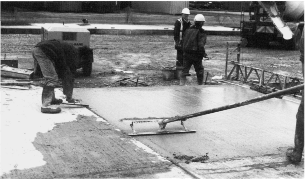
Fig. 5.46. Finishing the surface with the float prior to applying the brushed finish
