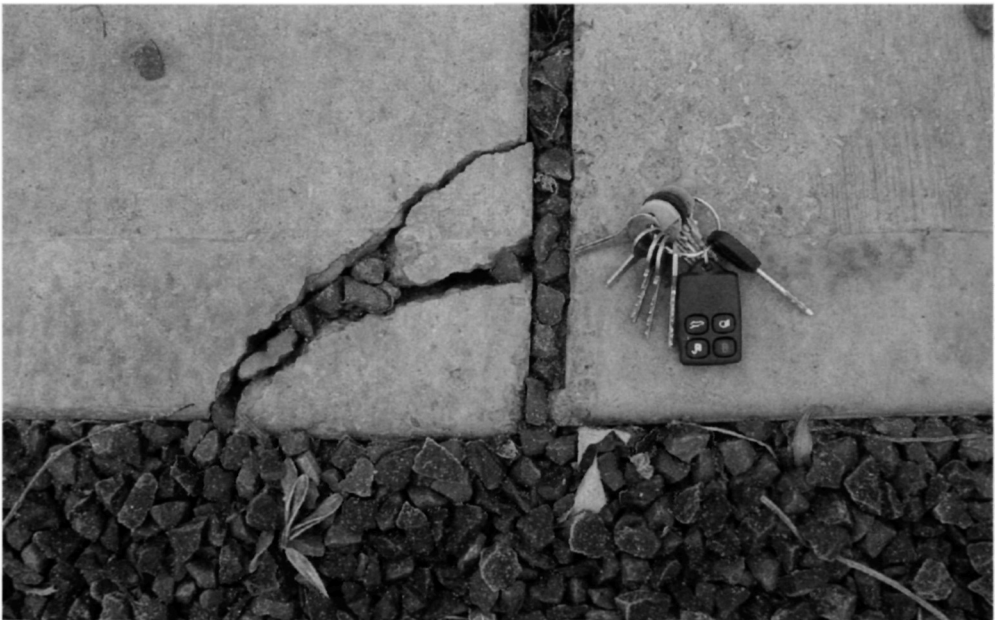
Fig. 5.107. This corner detail from Fig. 5.106 has deteriorated as a result of stones initially entering the unsealed joint, so prising the concrete apart. The same stones then entered the cracks and caused local failure of the corner of the slab
