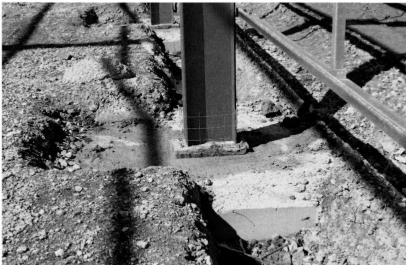
Fig. 5.24. The prop columns along the centre of the building have been bolted to their concrete foundations which are below the level of the underside of the floor slab. The floor slab will surround these columns
