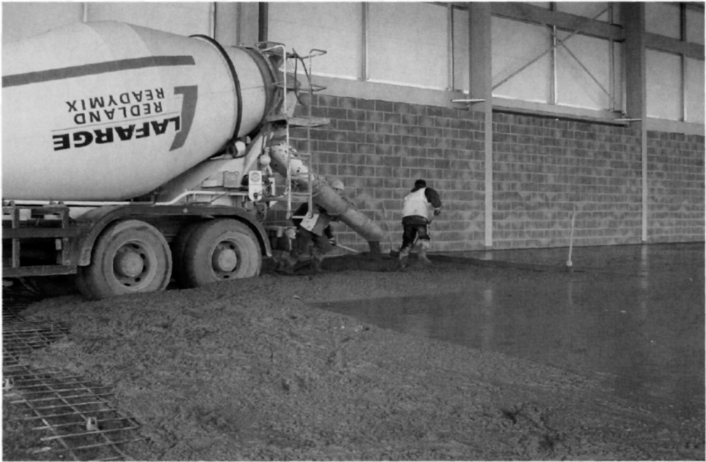
Fig. 5.95. The concrete delivery truck has to run over the mesh and this can lead to its being displaced. In this case, the mesh is positioned towards the underside of the concrete so the displacement is minimal. Designers should be aware of this
