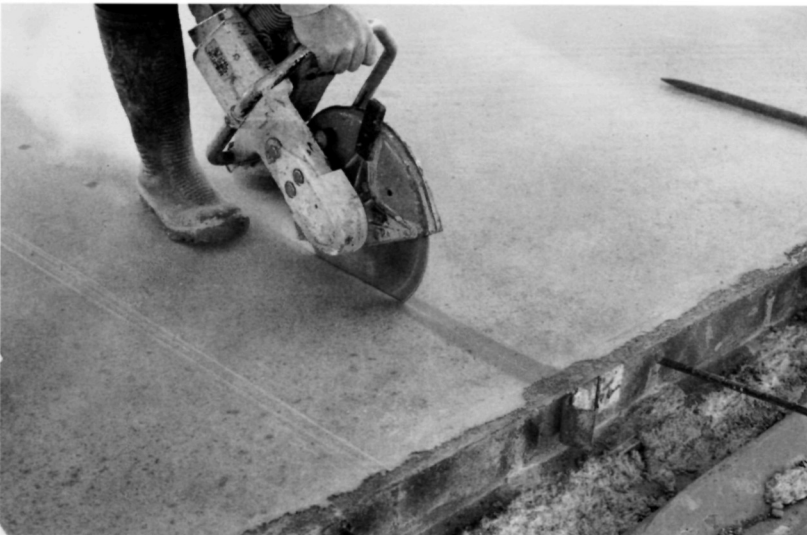
Fig. 5.41. A 3 mm wide by 40 mm deep groove is cut into the concrete using a hand-held saw. Care has to be exercised to ensure a straight cut. The reduction in cross-sectional area and second moment of area ensures that cracking occurs here. Note that the main mesh is stopped here and a shorter piece having its main bars running along the line of the cut contributes to the weakening at such joints
