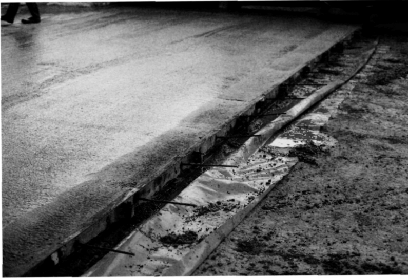
Fig. 5.34. The concrete is left to set. Note the excess slip membrane material and the tie bars. Because the roof sheets are fixed and the weather is cool, there is no need to take special measures to reduce moisture loss from the upper surface of the concrete
