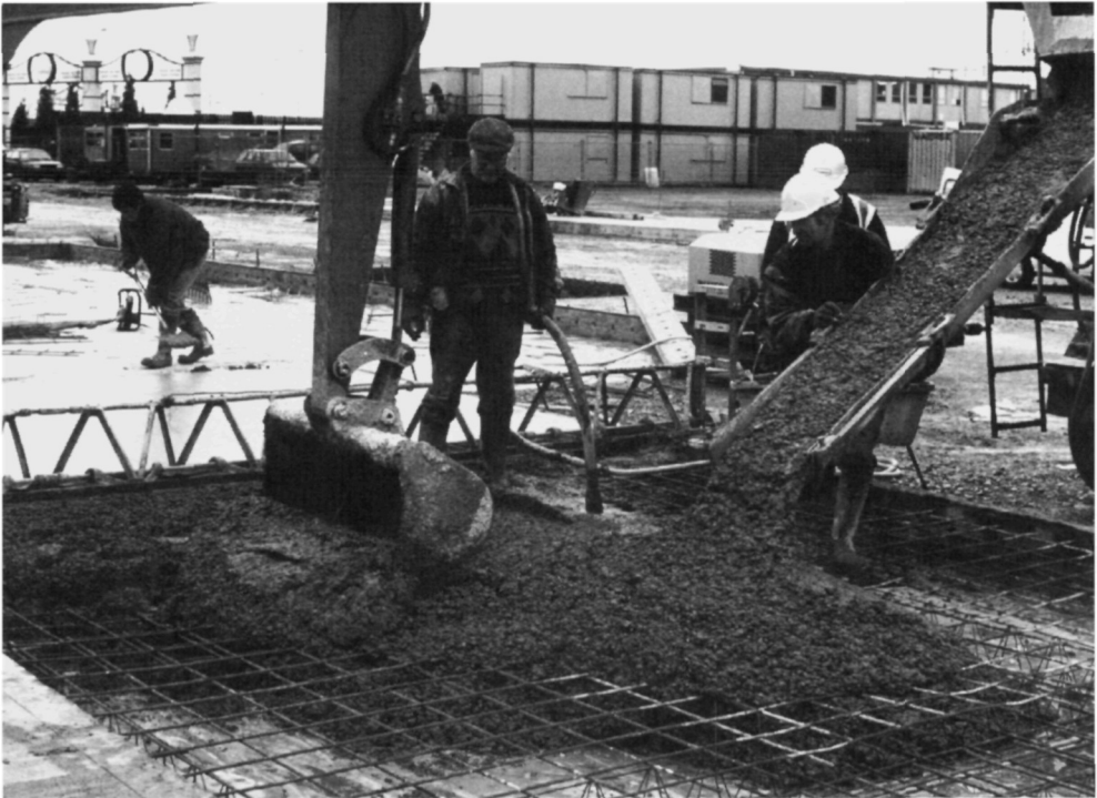
Fig. 5.48. A small excavator helps in placing the concrete. Because hardstanding concrete is of low workability, this saves much labour
