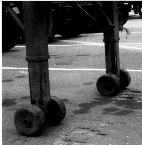
Fig. 3.8. These trailer dolly wheels have indented the bituminous material surfacing
