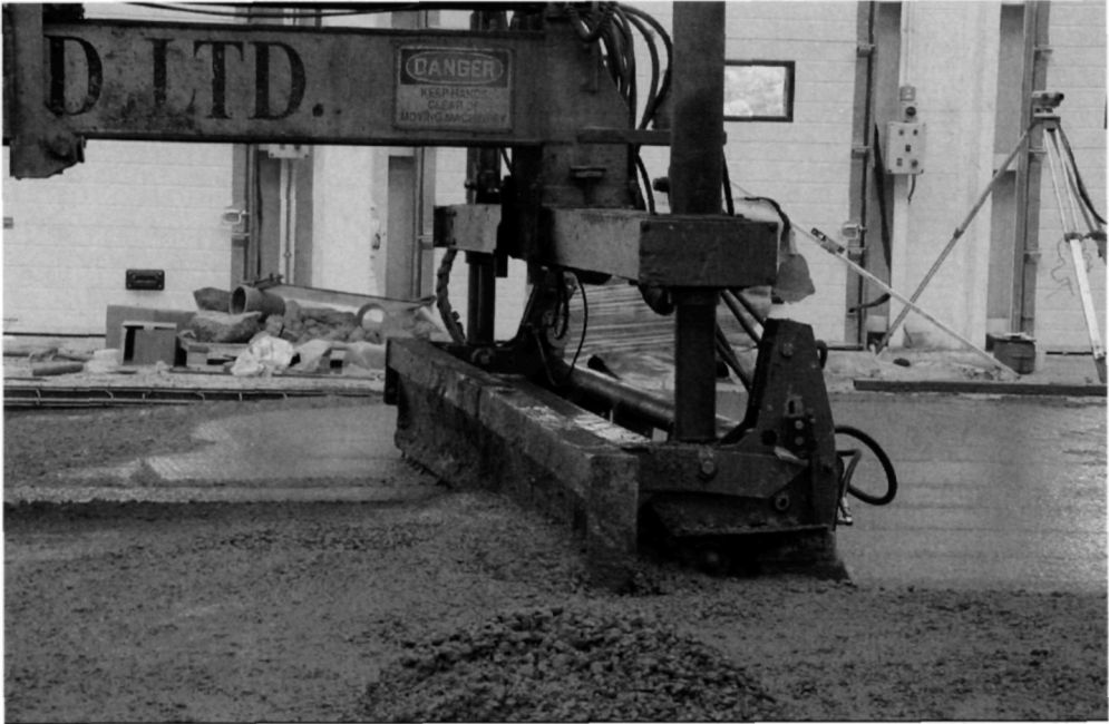
Fig. 5.16. Details of a laser guided screeding machine's screed carriage. A rotating vibrating tube places, compacts and finishes the concrete as the carriage is moved progressively towards the machine operator
