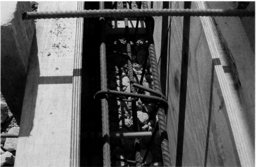
Fig. 5.90. The reinforcement has been fixed firmly to avoid disturbance when the concrete is poured
