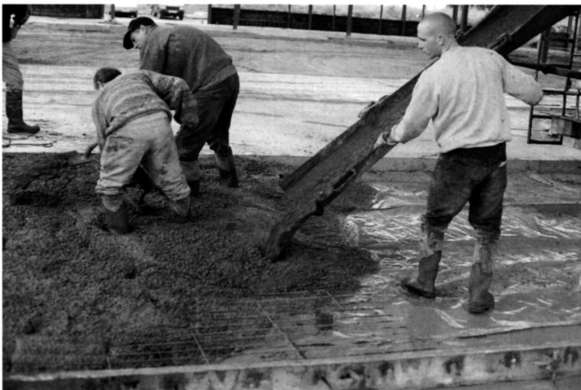
Fig. 5.28. The concrete is discharged between the formwork and, in this case, a previously constructed strip. A piece of mesh reinforcement has been installed. The concrete is discharged as close as possible to its required position and is moved by hand as required
