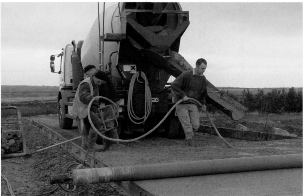
Fig. 5.69. Additional vibration is introduced using a poker vibrator to ensure that full density is achieved throughout the full depth of the concrete. The vibrating tube is most effective close to the surface of the concrete
