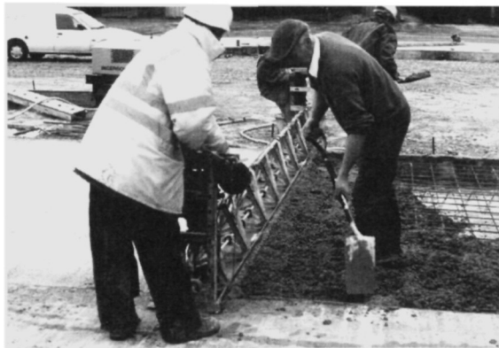
Fig. 5.44. The concrete is being compacted while the operative ensures that there is a little concrete surcharge in front of the twin beam compactor
