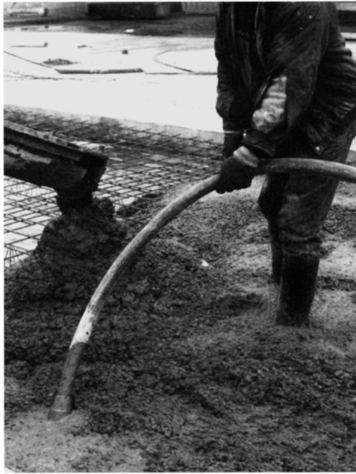
Fig. 5.51. A poker vibrator ensures that compaction is achieved to full depth. Care must be undertaken to avoid over vibrating which will lead to segregation
