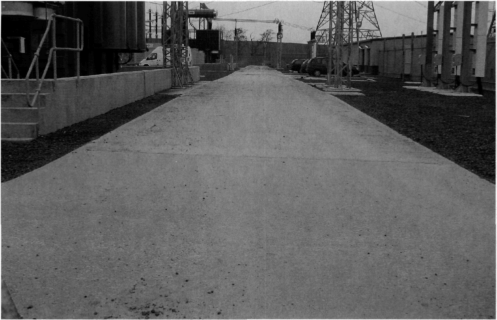
Fig. 5.102. This 5 m wide single lane industrial road was heavily trafficked during construction but should receive only light traffic during its service life. Construction traffic caused a number of defects
