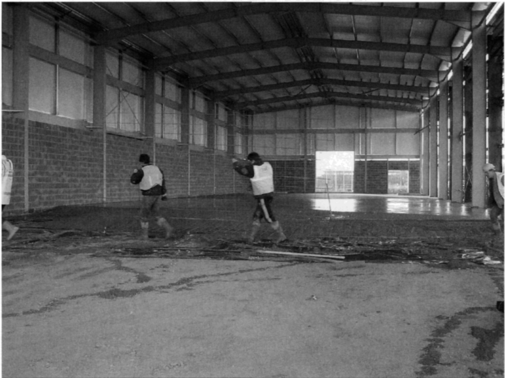
Fig. 5.94. A concrete floor is being installed in an extension to a building on a retail development in North Shields, UK. A piece of A142 mesh is being carried towards the concrete laying face. The floor is being cast against a concrete block wall to the left and an existing concrete floor to the right
