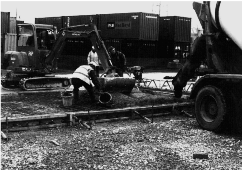
Fig. 5.50. It is common for industrial hardstandings to be extended and care needs to be exercised to balance the needs of the contractor with those of the hardstanding operator
