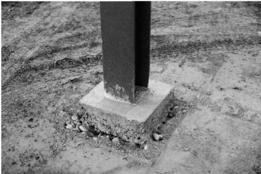
Fig. 5.26. Concrete has been cast around the column through the depth of the floor slab. A strip of compressible material will be fixed around the perimeter of this concrete to the full depth of the floor to ensure that the floor and the structural frame can move independently of each other
