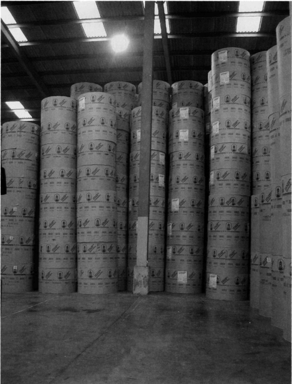
Fig. 5.74. Newsprint reels stored on this floor are leaning as the floor falls away from hard points at the internal columns. The columns had been piled and the floor has been concreted over the pile caps. The subgrade comprises fill material overlying peat. Consolidation settlement of the peat led to the floor settling differentially and cracking. This could have been avoided by allowing the floor to move vertically relative to the pile caps at the columns
