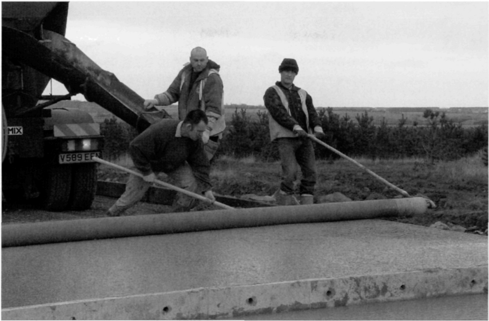
Fig. 5.68. The vibrating tube compacts the concrete as it is pulled along the formwork. Note the daywork joint in the foreground with holes in the formwork for the introduction of dowel bars
