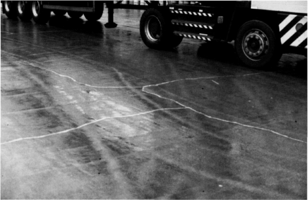
Fig. 5.80. Cracks have been sealed and the external hardstanding remains serviceable
