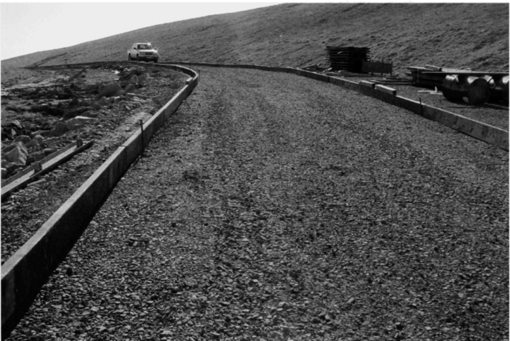
Fig. 5.61. The 150mm thick granular sub-base material has been installed and formwork has been pinned to the sub-base. The sub-base has been compacted using a vibrating roller — see Section 1.2
