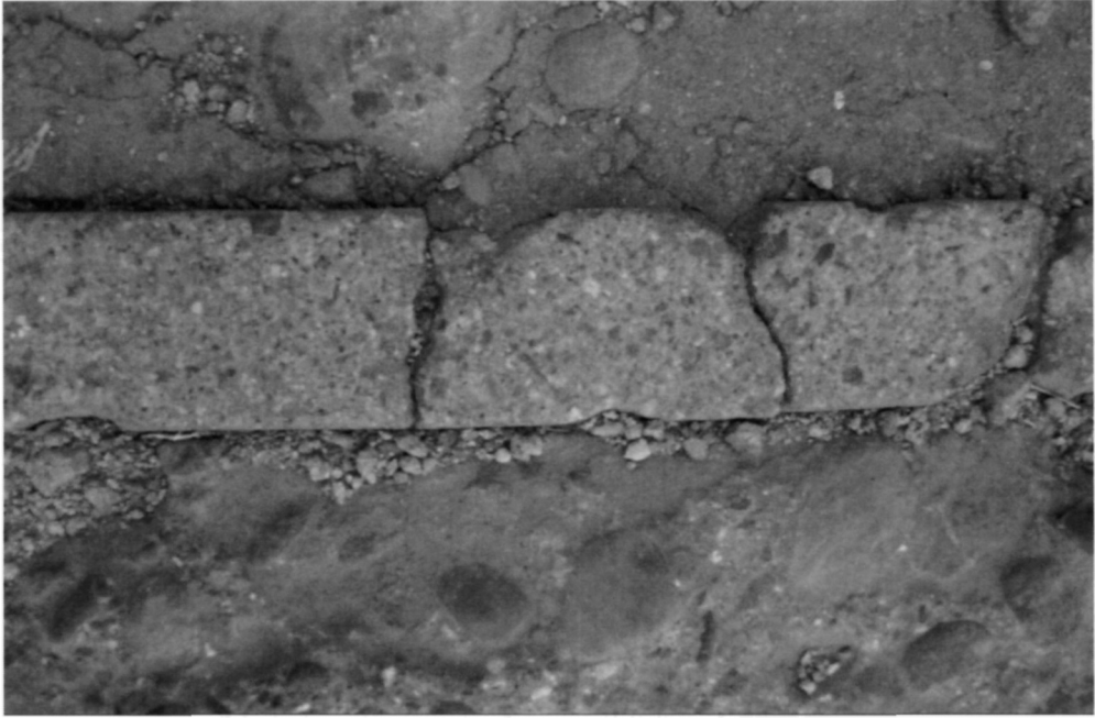
Fig. 5.109. Precast concrete units had been installed previously as permanent formwork at the slab joints. These had performed particularly poorly and were one of the reasons for the need for an overlay
