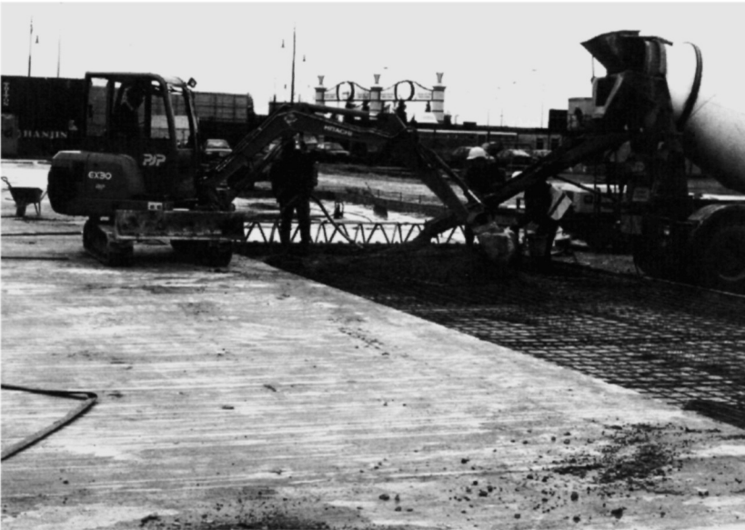
Fig. 5.49. The excavator allows concrete to be placed at a rate of 15 m 3 per hour
