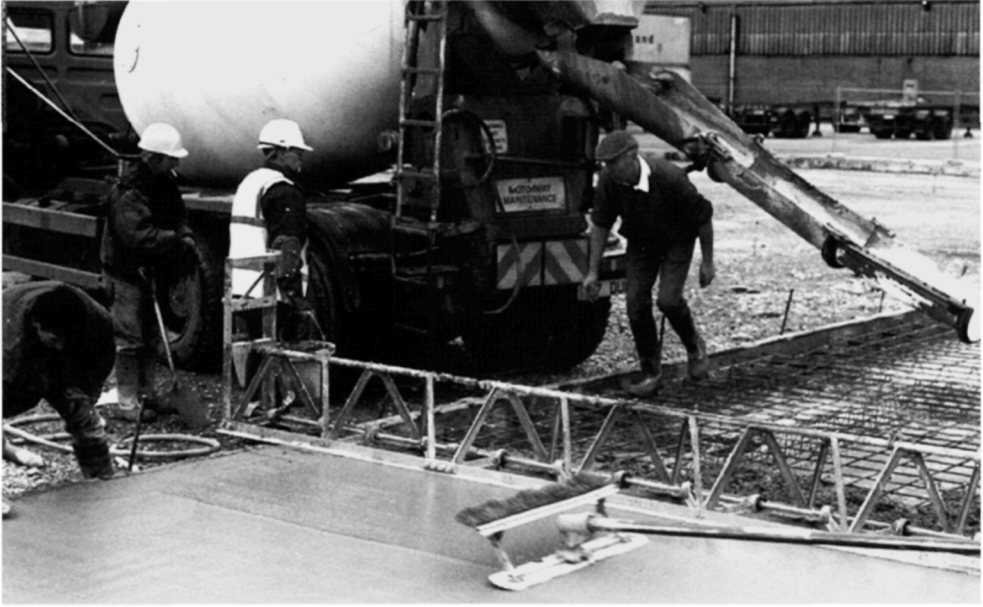
Fig. 5.47. The next bay is ready for concreting as finishing continues on the previous bay
