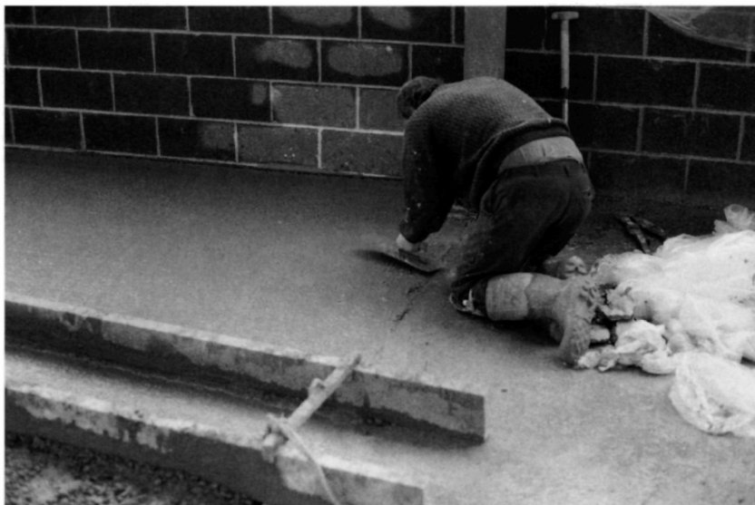
Fig. 5.33. The edges of the slab are trowelled to improve the quality of the longitudinal joint. This trowelling takes place immediately after the concrete has been compacted. Additional concrete may be placed to make up levels
