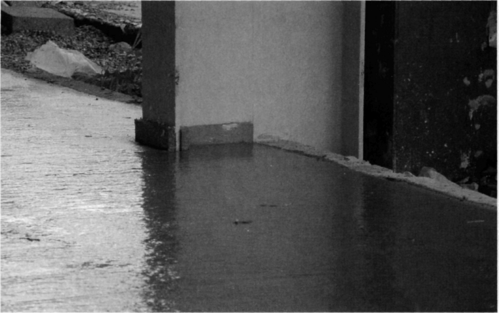
Fig. 5.99. The concrete has been compacted and screeded, and awaits power floating when it has gained sufficient strength to support the trowelling equipment. The fibre boards have ensured structural separation between the floor and the column, and will be trimmed later
