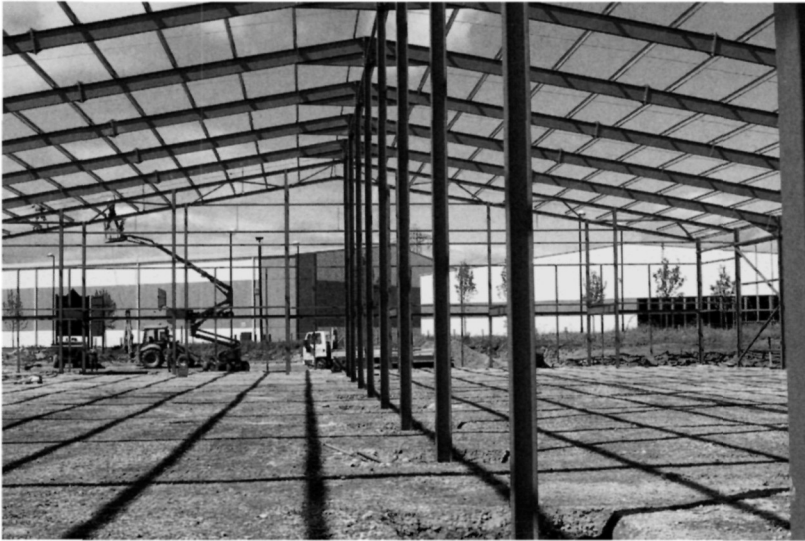
Fig. 5.23. The propped portal frame has been completed and the sub-base has been laid. Floor construction cannot start until the roof sheets have been fixed otherwise the sun could lead to rapid moisture loss from the concrete. This in turn could cause plastic cracking in the floor
