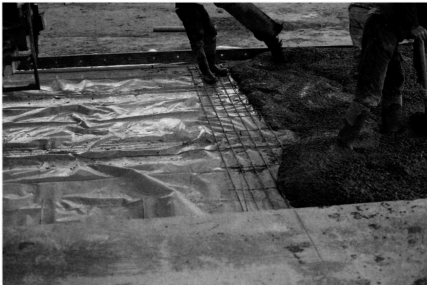
Fig. 5.32. A short length of mesh is placed near the underside of the concrete to act as the tie at a transverse tied joint. The main mesh reinforcement near the upper surface of the concrete is stopped short of the tied joint. Note that the main reinforcement runs normal to the longitudinal long strip direction. A transverse groove has already been cut in the neighbouring bay to complete the tied joint
