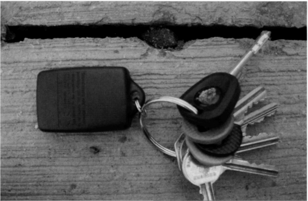
Fig. 5.105. This joint has not been sealed so allowing a stone to become lodged between the concrete slabs and spalling the concrete
