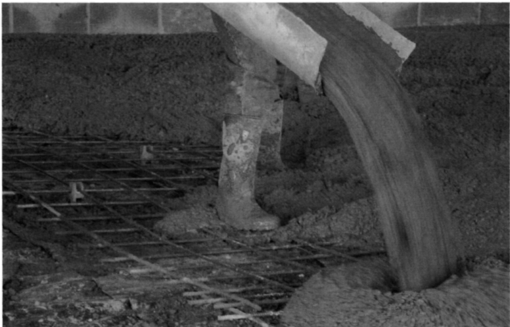
Fig. 5.96. The concrete is placed so as to avoid further movement of the material by hand. Inevitably, the reinforcement is deformed by the operatives and by the weight of the concrete
