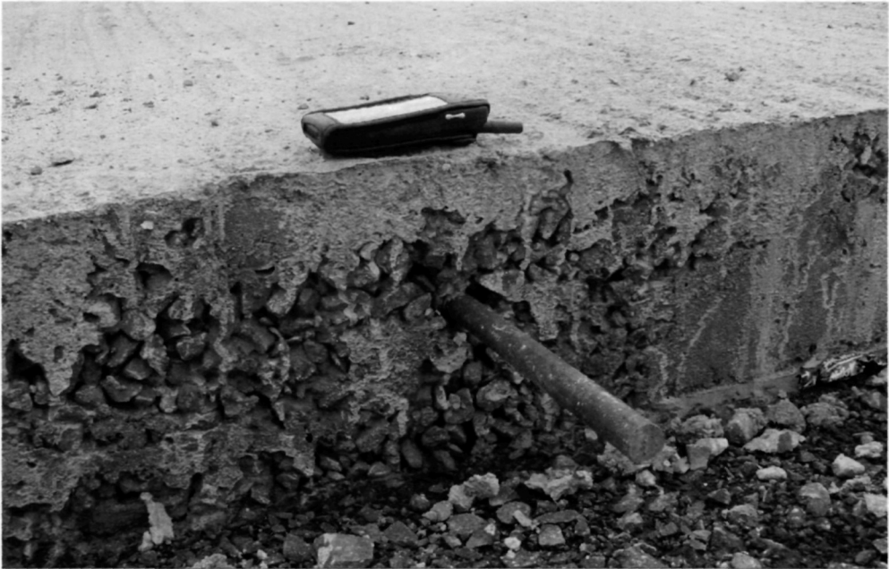
Fig. 5.72. Even with good levels of workmanship and supervision, lack of compaction can occur. Whether such material should be removed will depend upon the anticipated loading in the vicinity of the uncompacted concrete and upon the need to protect the dowel bars from corrosion
