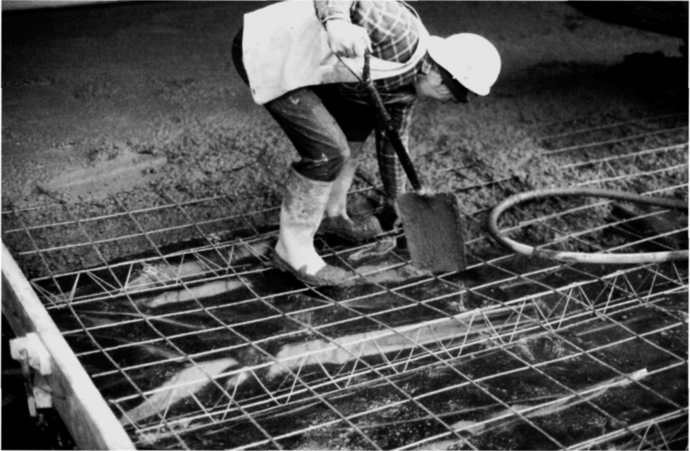
Fig. 5.84. Note how the operative deforms the mesh as he gains access to the concrete. It is common for mesh to vary in location as a result of its having been displaced in this manner
