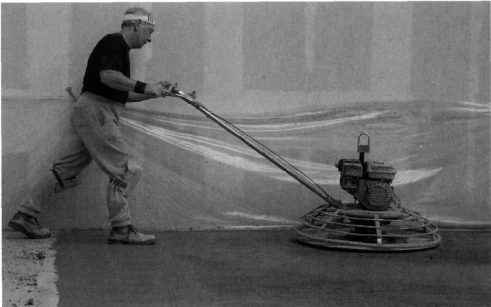
Fig. 5.17. Power trowelling machines ensure a durable abrasion resistant finish. The operator rides on larger machines (see Fig. 5.19) but smaller machines are operated as shown in this figure
