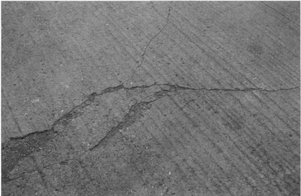
Fig. 5.108. This concrete hardstanding has proven inadequate to sustain regular trafficking by front lift trucks with 95 t front axles handling 40 ft containers. In order to continue using the concrete in the same way, it was decided to undertake a concrete block paving overlay
