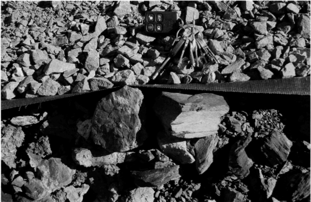
Fig. 5.63. A woven geotextile fabric separates the sub-base from the underlying mudstone fill. This prevents the sub-base material from penetrating the fill, while allowing the free drainage of water
