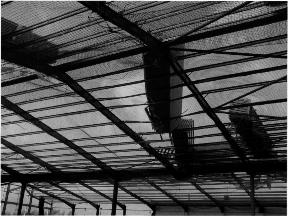
Fig. 5.101. Although high wind has little impact upon floor installation, high winds during January 2002 caused sheeting stored on the roof of the adjoining portal framed building to blow over and damage the purlins. The safety nets would not arrest any heavy falling sheets. Gusts in excess of 35 m/s were measured nearby and this should be compared with the basic design wind speed of 46 m/s at this location. The basic design wind speed is the average speed of a three second gust likely to recur every 50 years. Because concrete floor construction always takes place in the context of the construction or modification of a building, factors such as high wind may impact floor installation
