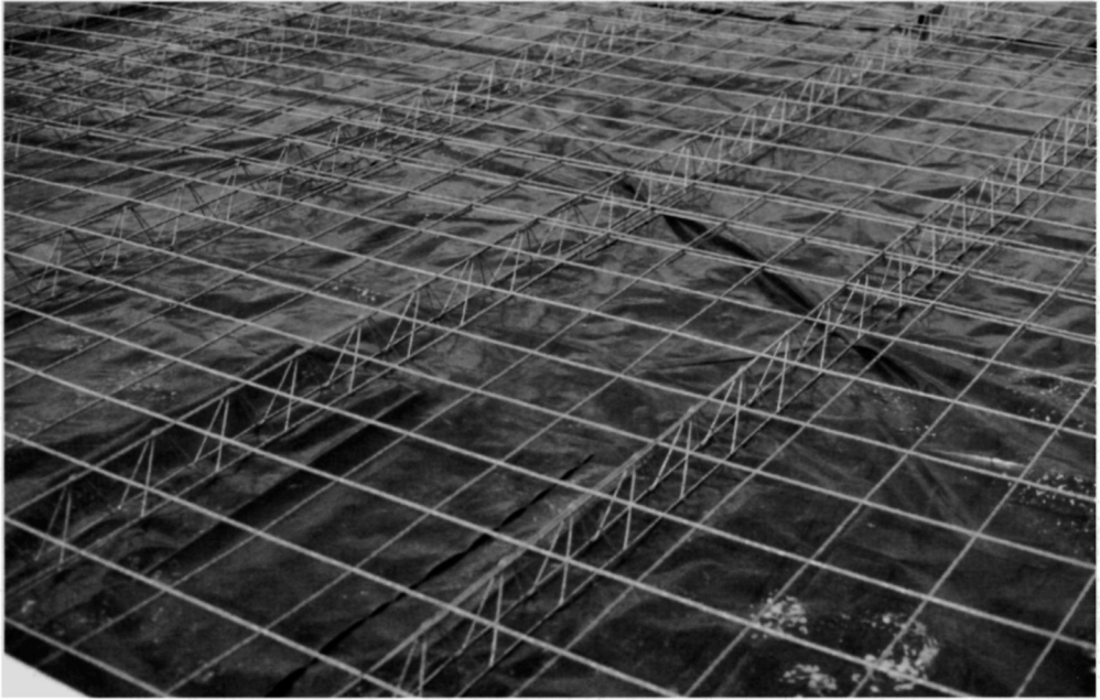
Fig. 5.82. A polyethylene slip membrane was introduced and the mesh was supported on fabricated supports
