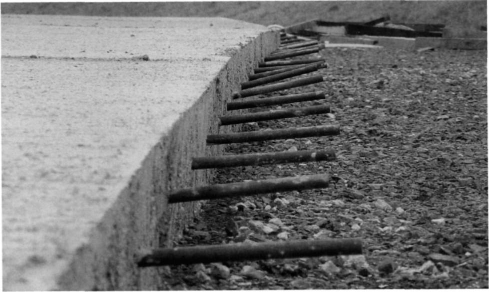
Fig. 5.66. Dowel bars have been fixed along the edge of the road where a passing lay-by is to be concreted. Note the difficulty in ensuring that the dowel bars are all parallel. Even one misaligned dowel bar can lead to the joint locking, which can cause cracking of the concrete
