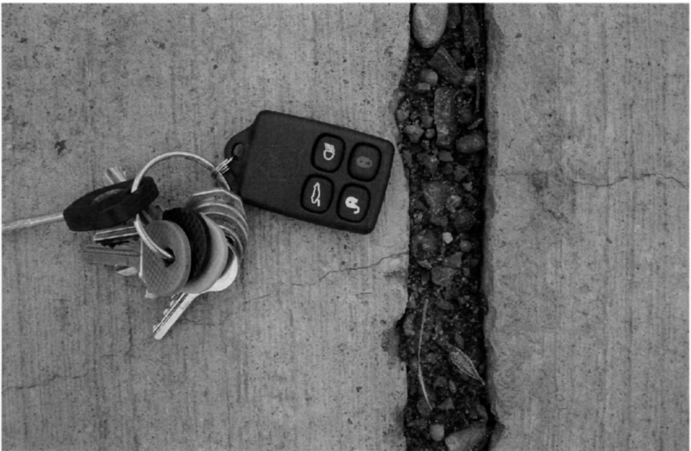
Fig. 5.103. Minor longitudinal cracks caused by hogging moments when heavy construction vehicles trafficked the site here meet a full movement joint
