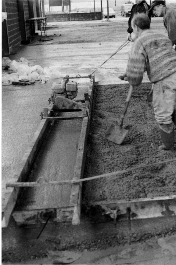
Fig. 5.31. A double vibrating beam is pulled along the formwork to compact the concrete. A member of the team ensures that there is sufficient concrete along the length of the beam. Tie bars have been inserted in holes in the formwork
