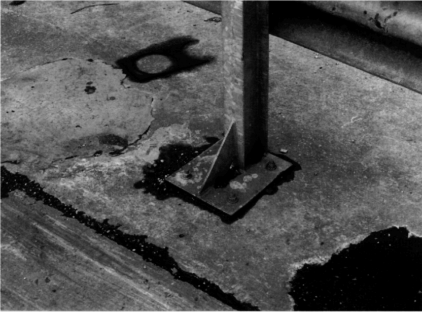
Fig. 5.57. It is common for safety fencing to be fixed to the surface of the concrete using expanding bolts
