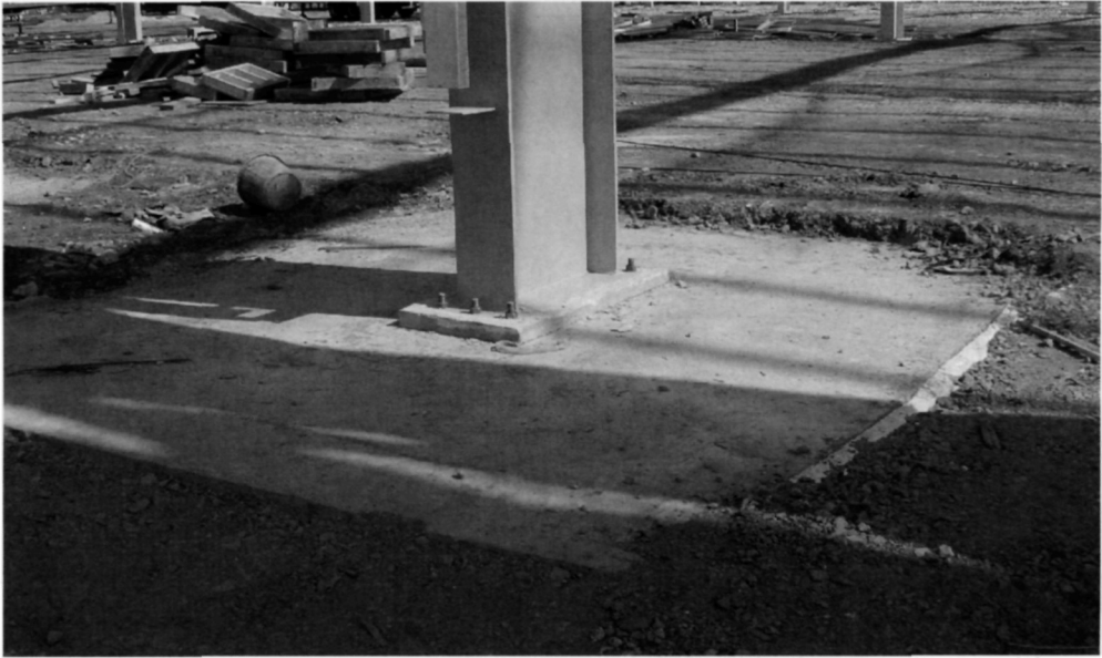
Fig. 5.87. Note the 3 × 3 m pad foundation. This spreads the column load so as to avoid overstressing the underlying weak fill material which had been used to fill the old Tyne Dock
