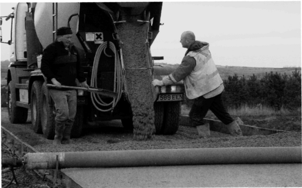
Fig. 5.67. Concrete being delivered. This narrow road required the concrete delivery vehicle to reverse the whole length of the road. This can lead to rutting of the sub-base and it is sometimes necessary to recompact the sub-base material between deliveries. The rotating tubular beam compacts the concrete
