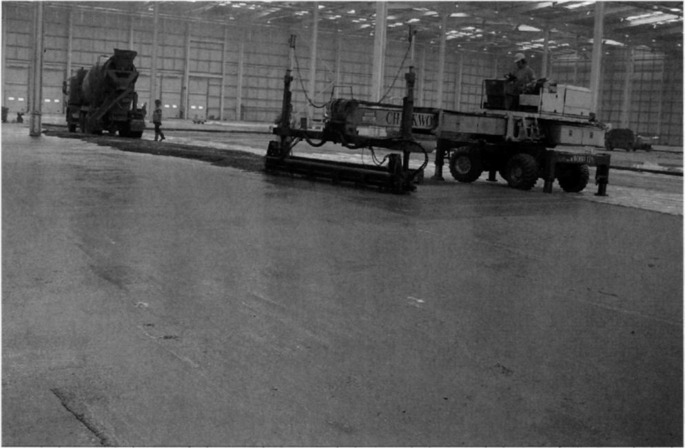
Fig. 5.18. The management of the delivery of concrete is a crucial element in single pour floors. It is common for over 500 m 3 of concrete to be placed in one day
