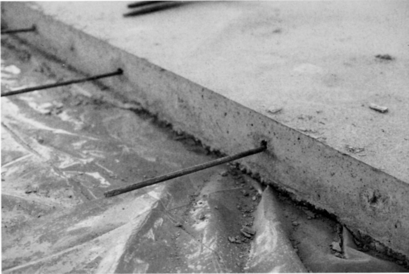
Fig. 5.38. The finished slab with the formwork removed showing the tie bars ready for the neighbouring long strip. This concrete can be used as formwork for the next long strip. Sometimes the alternate strip method is used whereby the initial long strips require formwork at each side and the intermediate strips use the previously cast concrete. In this case, one central long strip was cast using formwork at each side. All of the subsequent strips were cast using one existing concrete long strip and one side of formwork
