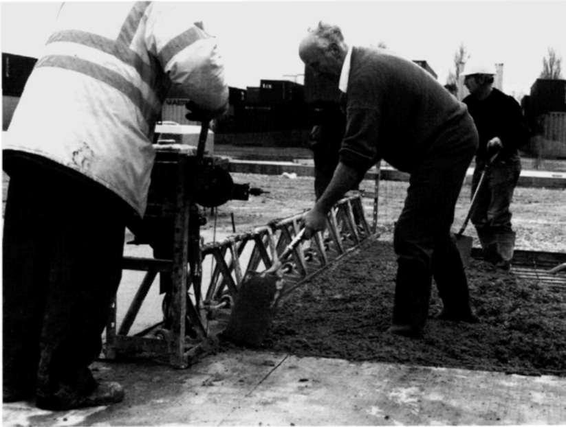
Fig. 5.55. The winching of the twin beam compactor is coordinated with the maintaining of surcharge to ensure uniform compaction
