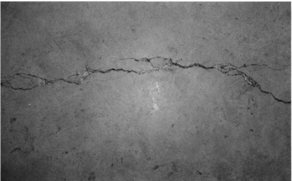
Fig. 5.78. The movement of the floor is causing a tearing action to occur. The concrete is being held together by steel fibres spanning the tear. Trafficking will remove the torn pieces leading to a severely spalled joint
