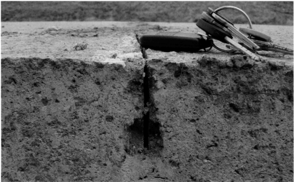
Fig. 5.71. 4 mm wide by 60 mm deep saw cuts are formed at 6 m centres to reduce stresses resulting from temperature related volume changes. The saw cuts will be sealed to prevent the ingress of detritus. The saw cuts are made as soon as the concrete can be cut without damage. Waiting too long could lead to mid-bay cracking
