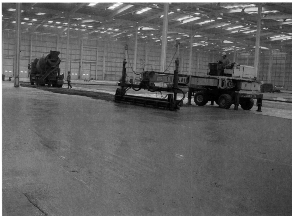
Fig. 2.2. Laser guided screeding machine. The carriage to the left is pulled towards the remainder of the machine and thereby places, compacts and levels the concrete in one operation. The levels are controlled automatically so the operator can focus upon moving the concrete. 2000 m 2 can be installed daily using this technique
