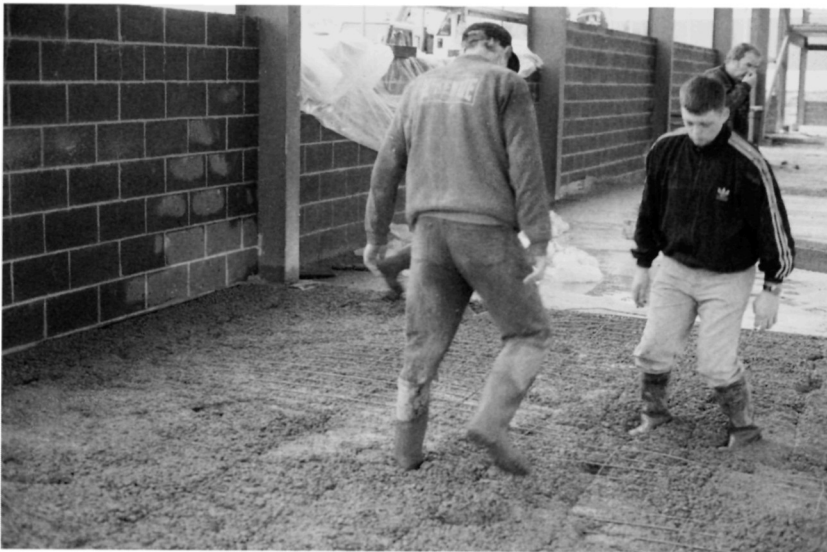
Fig. 5.30. The mesh is pressed into the concrete by members of the concrete gang walking over it. The mesh can be located with a surprising degree of accuracy by a skilled team. Care is taken to ensure sufficient overlap with neighbouring pieces of mesh. A cropping tool is on hand to deal with obstructions
