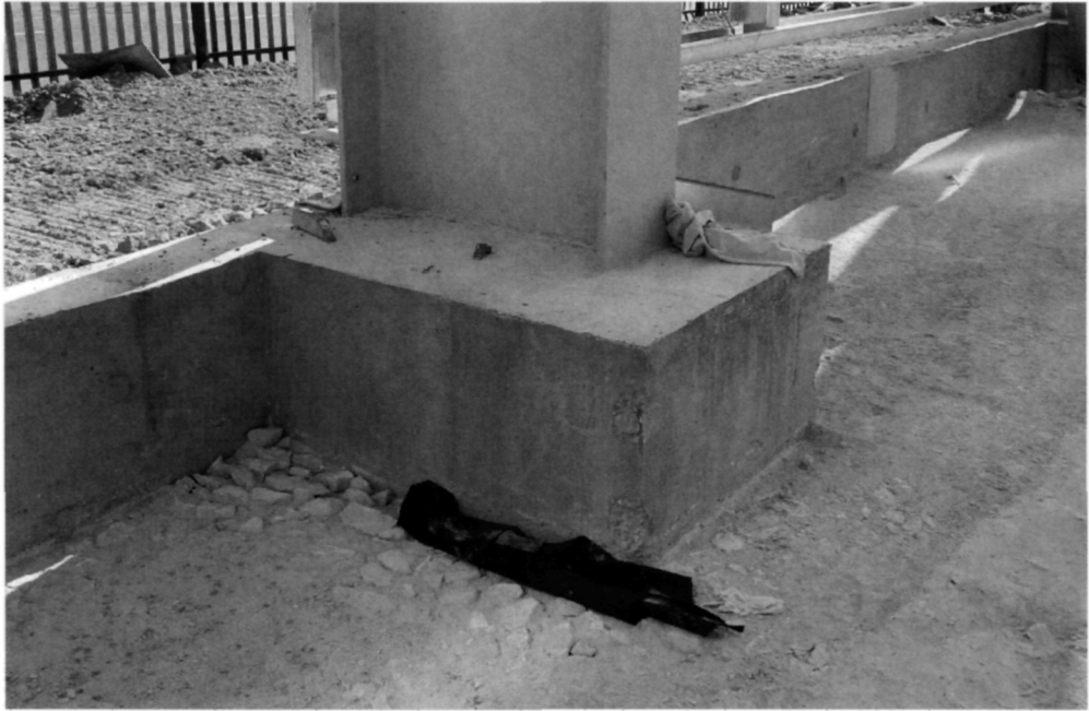
Fig. 5.93. The perimeter beam has been cast successfully around this column. Note the absence of air pockets in the concrete indicating a good level of compaction
