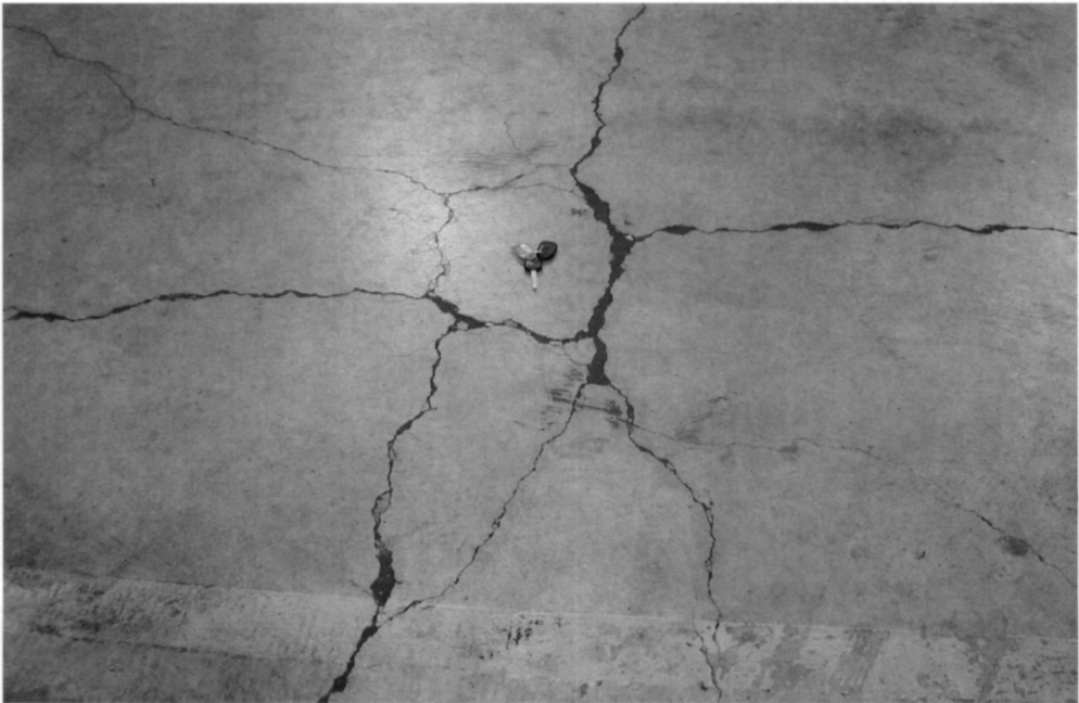
Fig. 5.76. A hard spot has been left in place beneath the floor leading to this pattern of cracking. The concrete near the keys is higher than the surrounding concrete
