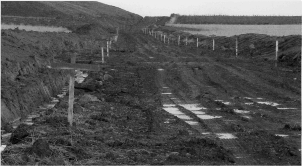
Fig. 5.60. Vegetation has been stripped and subgrade fill has been installed. Timber profiles have been fixed along the length of the road to allow levels to be established and verified. The granular sub-base material will be installed following the drying and final preparation of the subgrade. Note the open drainage ditch to the left of the line of the road
