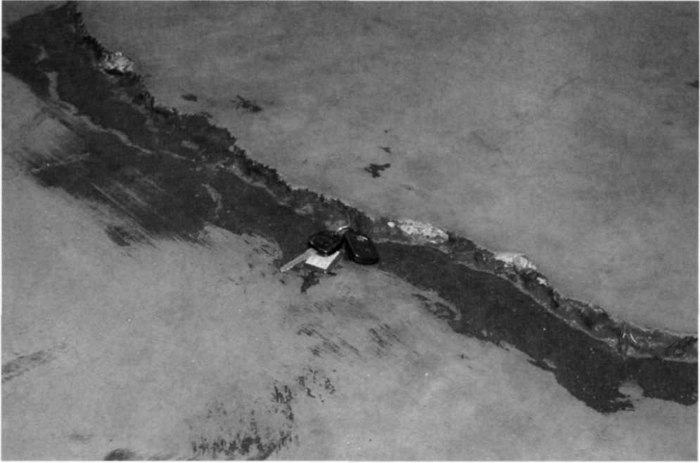
Fig. 5.77. An attempt has been made to seal a crack but continued relative vertical movement of the slabs each side of the crack is leading to the need for continued maintenance
