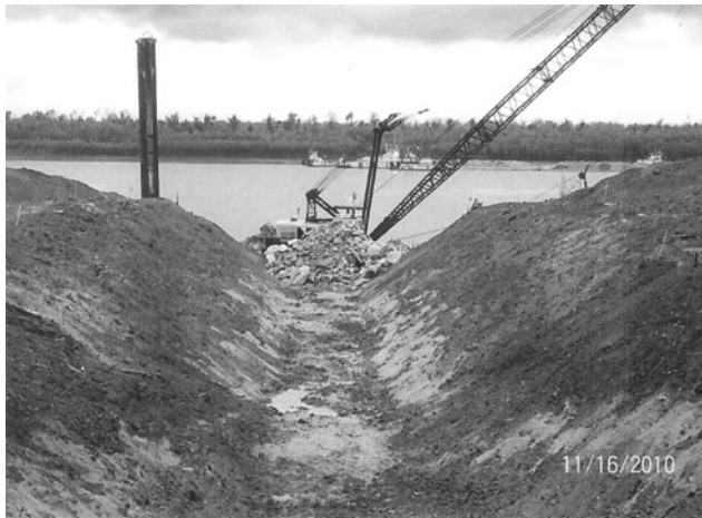
Fig. 5-5. Excavated trench for stone root on the Mississippi River Source: USACE Vicksburg District
