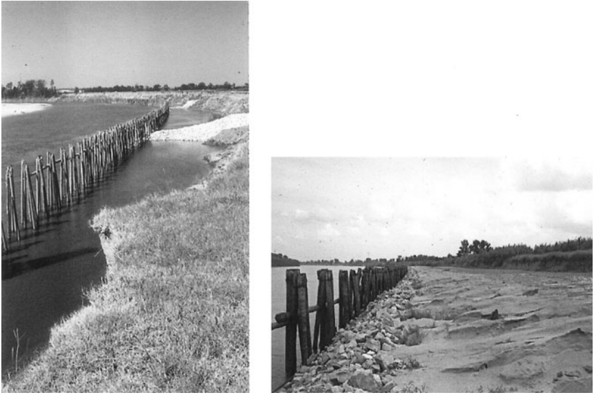
Fig. 6-4. Pile revetment on the Red River in Louisiana immediately after construction (a) and after sediment deposition had occurred (b)
