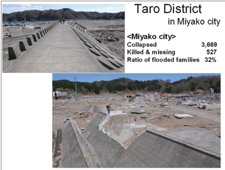
Fig. 7 Tsunami banks in Taro district destroyed by 2011 EJ tsunami
