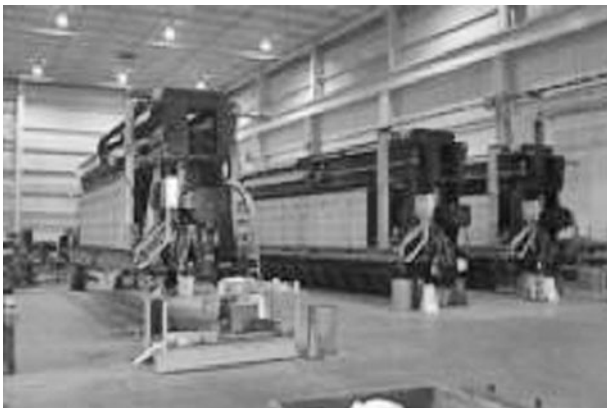
FIGURE 9.22 An example of filter presses at a steel works plant (courtesy of Siemens Water Technologies).
