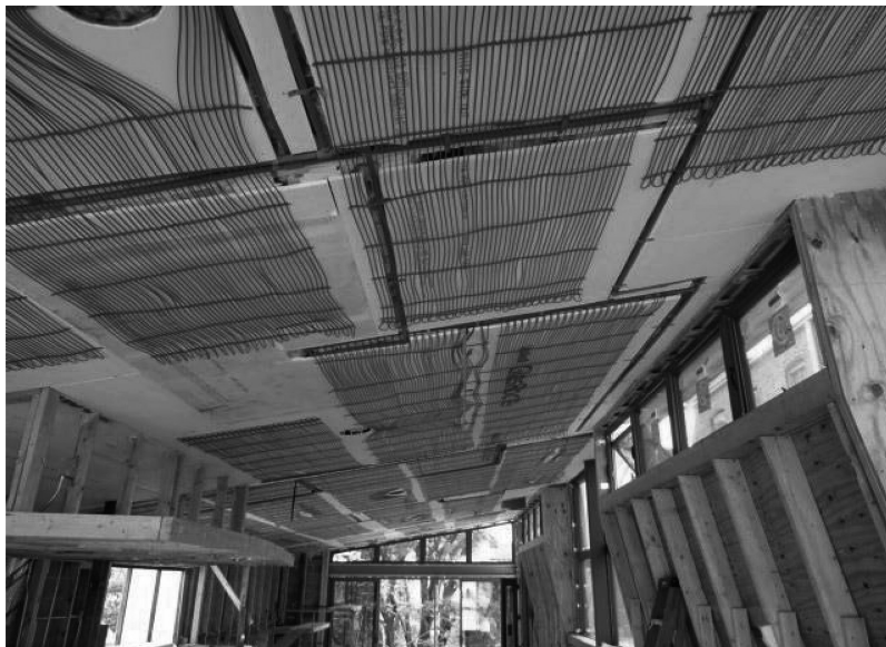
FIGURE 18.13 Photograph of a capillary tube network of radiant ceiling cooling coils.
