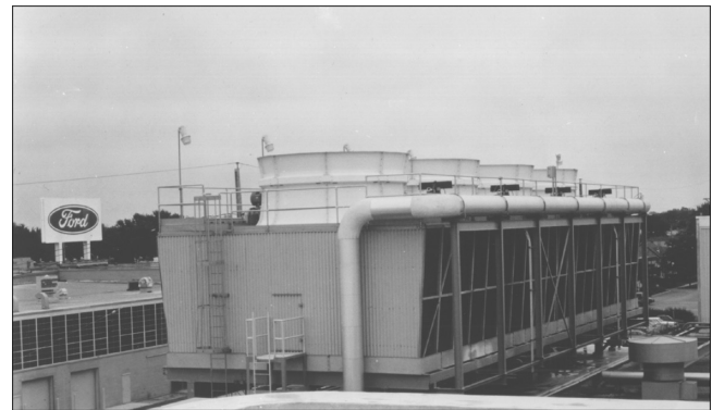
FIGURE 11.27 Induced draft cooling tower system (four separate towers are shown).
