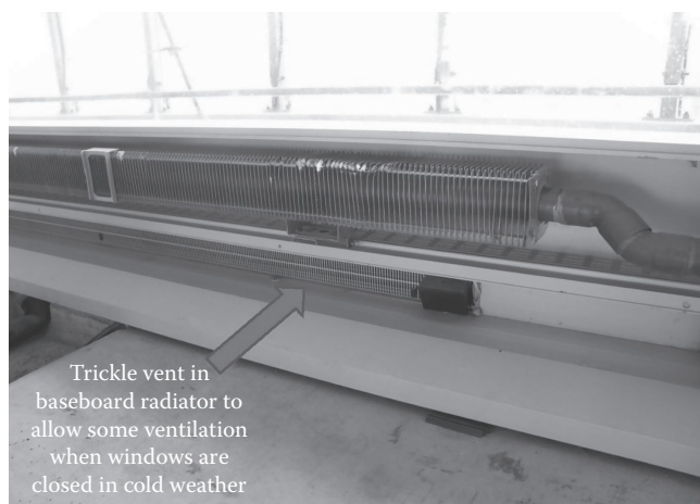
FIGURE 20.1 Photo of a room with trickle ventilation along with baseboard heating. (Image courtesy of Erik Kolderup.)
