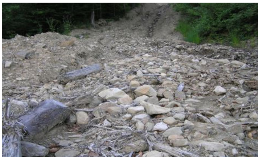
Fig. 4.3 The fan of the mudflow activated by deforestation of slopes in summer 2004 and a heavy rainfall event on 10 June 2005 (an intensity of 56 \text{ mm} \cdot \text{day}^{-1} recorded at the meteorological station in Oriava) (photo by O. Pylypovych)
