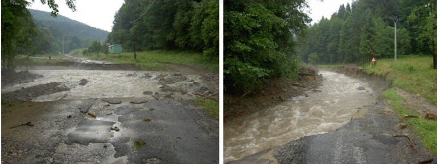
Fig. 3.5 Damaged road passing the Topľa River during flood, on 23 July 2008 (photo by M. Frandofer)
