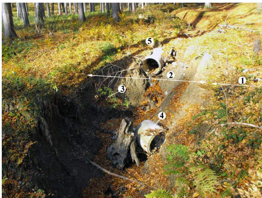
Fig. 19.8 Culvert in the Bozsok Valley on October 30, 2010. 1 – Valley floor. 2 – Channel. 3 – Caved-in channel side. 4 – Displaced concrete ring. 5 – Stable concrete ring
