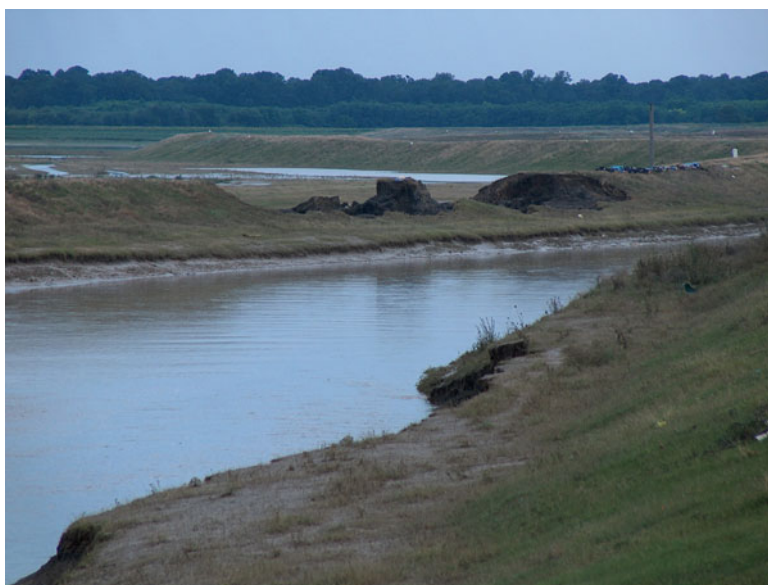
Fig. 7.2 Dam breach at Condrea village
