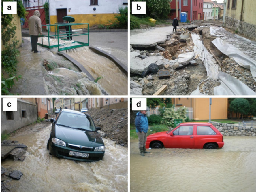
Fig. 22.6 Damages in the Vince Street on 17 May 2010. (a) Clogged drainage filter at the northern end of the street; (b, c) damaged road surfaces; (d) accumulation of deposits at the southern end of the street and on Ágoston Square (Photos by L. Ronczyk)
