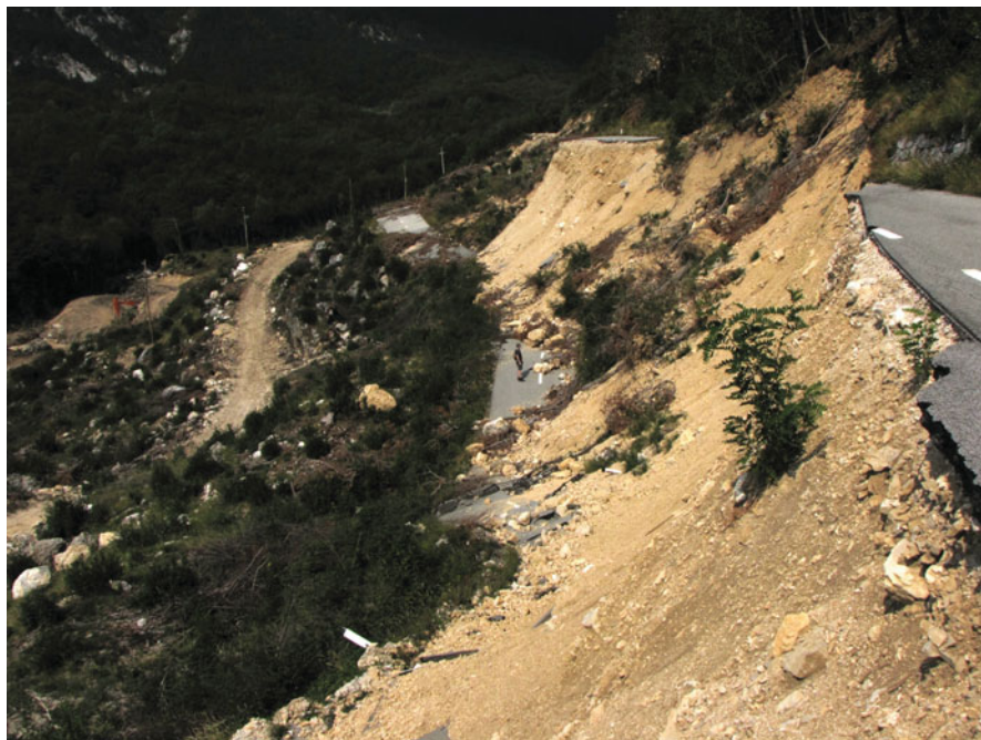
Fig. 8.7 During extensive precipitation in September 2010, the Stogovce landslide was triggered, which destroyed a kilometer of the road between Ajdovščina and Predmeja (photo by M. Zorn)
