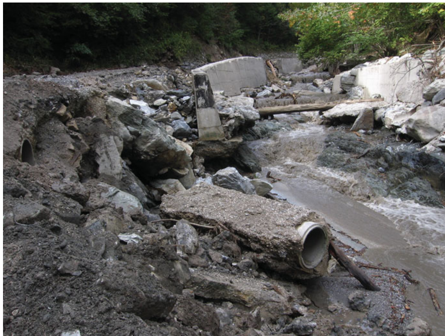
Fig. 8.4 Consequences of flash floods in the Davča Valley (western Slovenia) during the 2007 floods (photo by M. Zorn)
