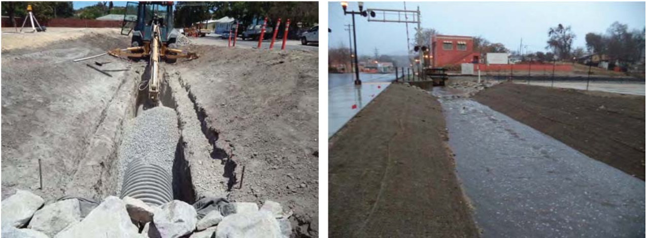
Figure 9. Construction of Drainage Trench on 21 st Street (Left); Drainage Trench During Storm Event (Right).
