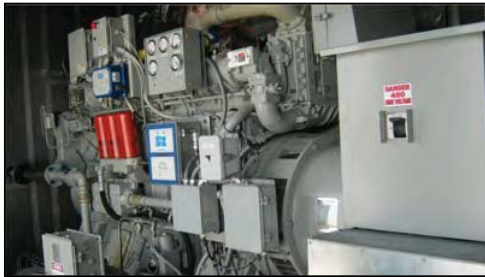
Photo 6 – 375KW Biogas Engine Generator
