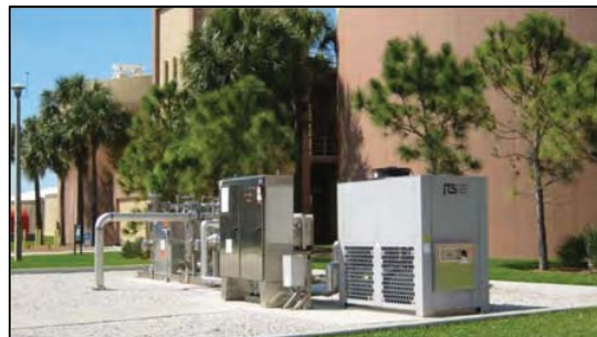
Photo 8 – Gas Pretreatment System
