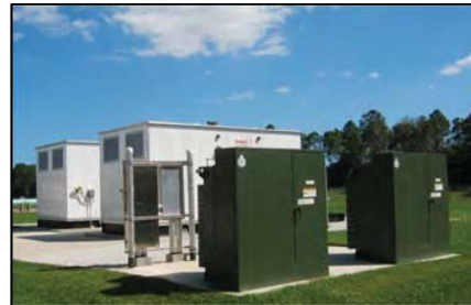
Photo 7 - Biogas Generator Enclosures with Transformers
