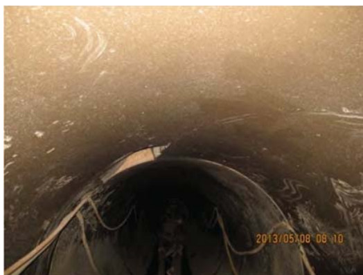
Figure 7-a- Crack in pipe
