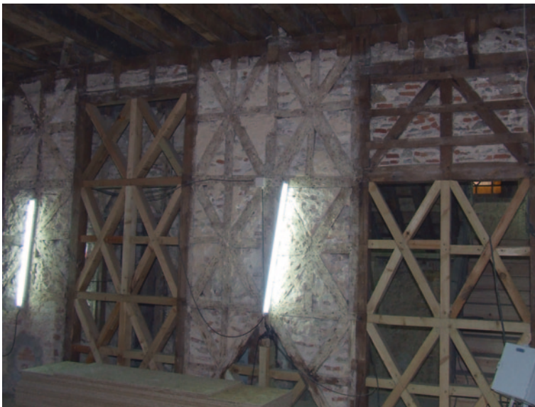
Fig. 26 Wall systems in the reconstruction after the 1755 Lisbon earthquake. Contemporary intervention on such a Pombalina type house
