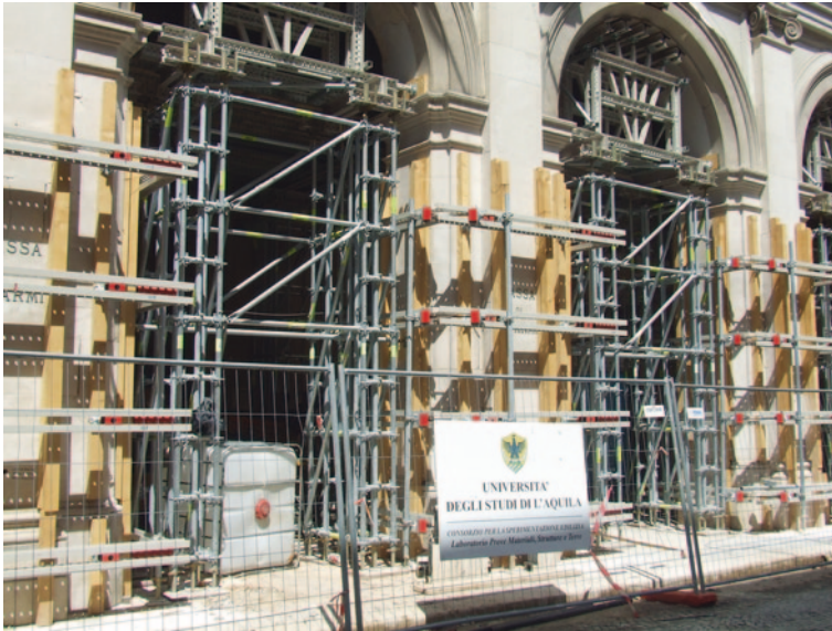
Fig. 25 Temporary propping in L'Aquila one year after the earthquake. Inspiration for Michele de Lucchi. Photo M. Bostenaru 2010
