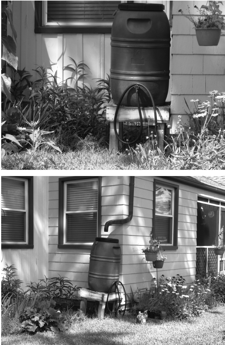
FIGURE 1.4 Household rain barrel collection system. (Photographs by author.)
